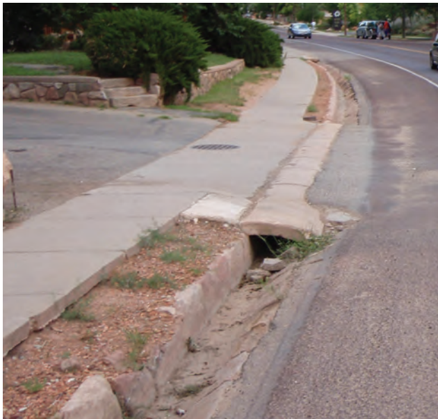
Debris in gutter and deterioration of the rock ditch wall at the elk ranch
