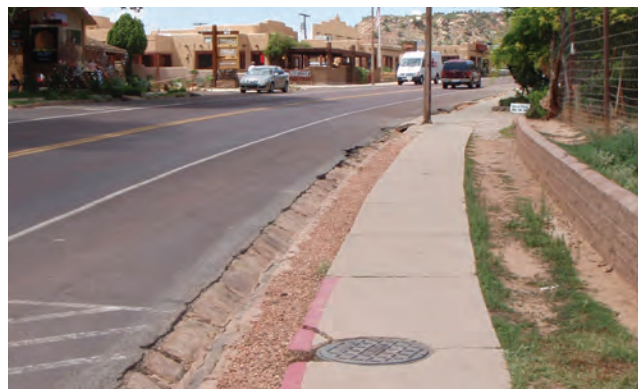
Sidewalk cracking at manhole cover
