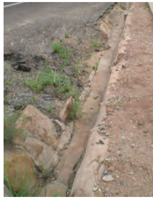
Eroding gutter at Terrace Brook Lodge
