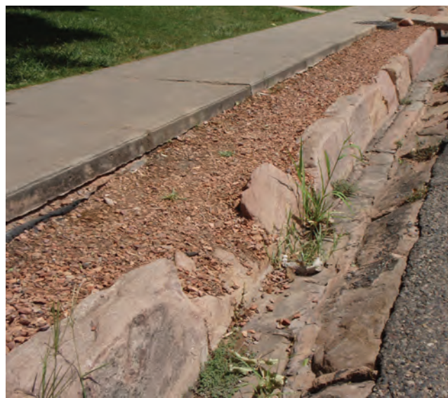
Rock ditch in disrepair between the elk ranch and Pioneer Lodge
