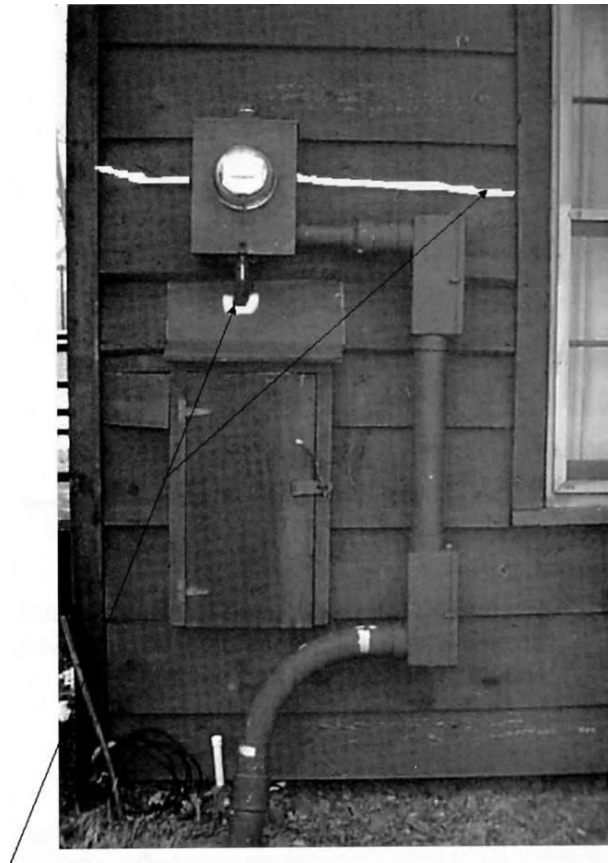
Calk used to eliminate hole around utility line and crack in siding
