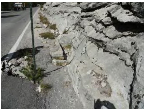
FIGURE 32. EROSION ALONG ROAD SHOULDER
