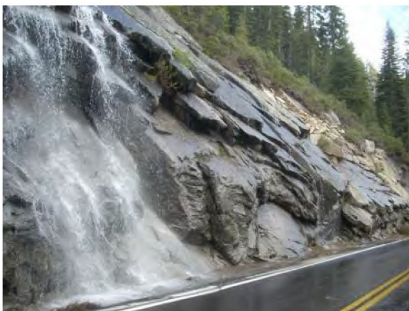
FIGURE 16. POOR DRAINAGE ALONG TIOGA ROAD
