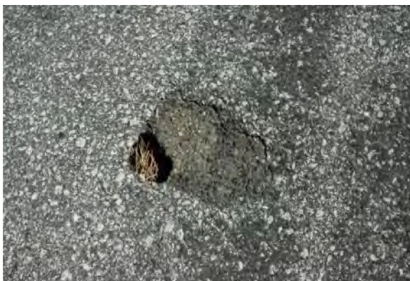
FIGURE 23. HOLES IN ASPHALT
