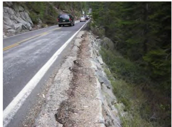
FIGURE 3. FAILURE OF CURB/ROAD SHOULDER
