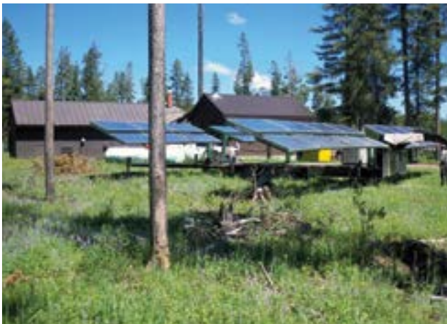
This portable photovoltaic system at Bechler provides power during the summer season, meeting 90% of the site's electrical needs.
