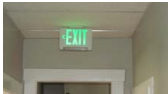
FIGURE 408. Exit light at corridor 105. Photograph by Alvine, May 15, 2013.
