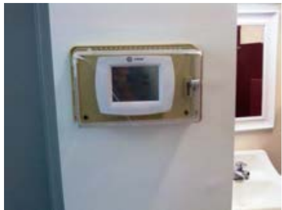
FIGURE 456. HVAC system control thermostat at men's restroom 103. Photograph by Alvine, May 15, 2013.
