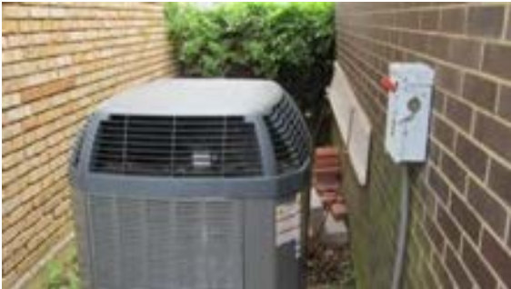
FIGURE 472. The comfort station condensing unit disconnect switch. Photograph by Alvine, May 15, 2013.
