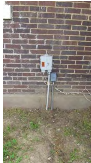
FIGURE 416. Outside telephone DeMark service entrance location. Photograph by Alvine, May 15, 2013.
