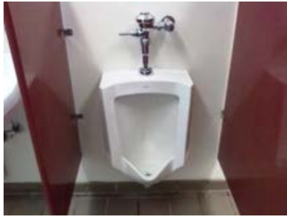
FIGURE 461. Wall-mounted flush-valve urinal at men's restroom 103. Photograph by Alvine, May 15, 2013.
