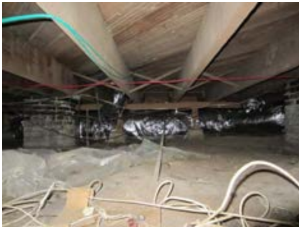
FIGURE 363. Brick masonry piers were partially visible behind HVAC ductwork at the centerline of the house, and supplemental masonry piers were observed supporting spliced joists at midspan. Additionally, concrete footings and 4 by 4 timber framing were later added to provide supplemental support to the first floor joists, view looking north. Photograph by WJE, October 17, 2012.
