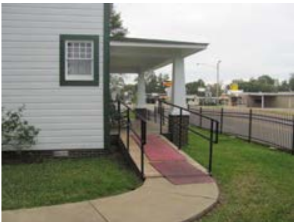
FIGURE 71. A view of the wood ramp leading to the front porch. Photograph by WJE, October 16, 2012.
