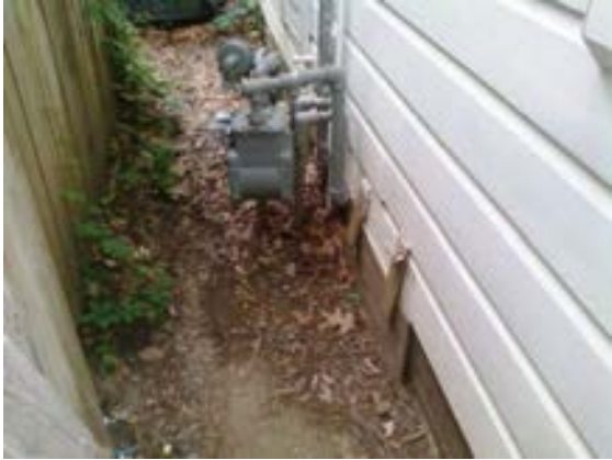
FIGURE 226. Cassidy House gas meter and service entrance location at east side of house. Photograph by Alvine, May 15, 2013.
