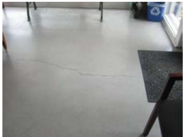
FIGURE 277. Concrete slab floor of the entry, looking north. Photograph by BVH, October 16, 2012.
