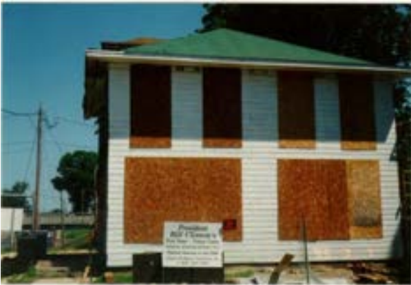
FIGURE 41. New siding and roof installed on the south side wall, July 7, 1995. Window openings are covered by temporary board-ups, and the front porch roof structure has been completely removed. Photo by Terry Huitt from the Clinton Home Restoration Scrapbook prepared by Cromwell Architects, 1997, page 17.
