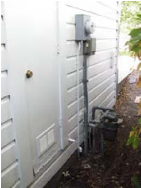
FIGURE 79. The base of the mechanical closet door shows signs of water damage. Photograph by WJE, October 15, 2012.
