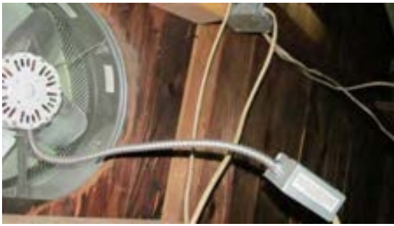
FIGURE 238. Wiring to exhaust fan in attic. Photograph by Alvine, May 15, 2013.
