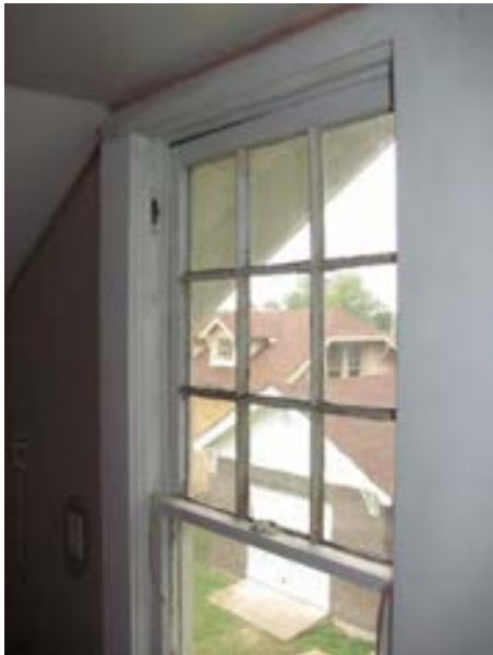
FIGURE 346. Detail of the south windows showing the cut weight cords. WJE, 2012
