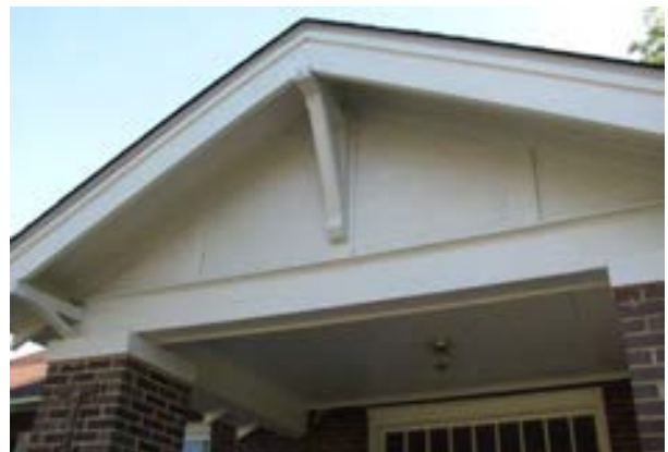
FIGURE 254. A view of the gable end of the front porch. Photograph by WJE, October 15, 2012.
