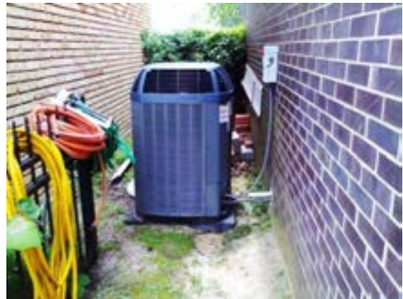
FIGURE 452. Grade-mounted air-cooled condensing unit located at east side of the comfort station. Photograph by Alvine, May 15, 2013.
