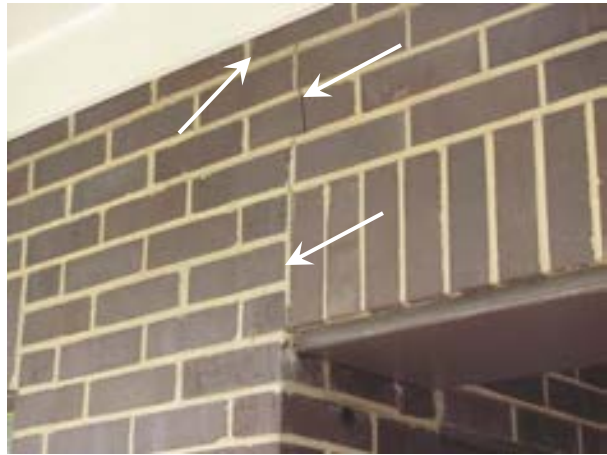
FIGURE 449. Vertical step crack propagating from the north corner of the lintel at the west building entrance. Looking east. Photograph by WJE, October 17, 2012.
