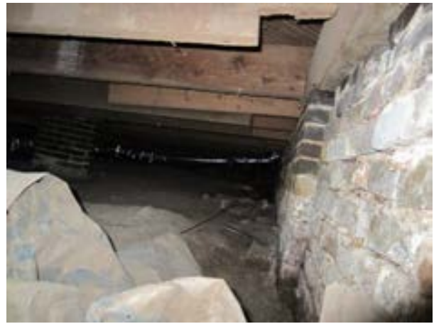
FIGURE 378. Brick deterioration and staining due to water damage at the interior of the perimeter foundation wall. Note, some mortar joints are eroded, view looking east. Photograph by WJE, October 17, 2012.
