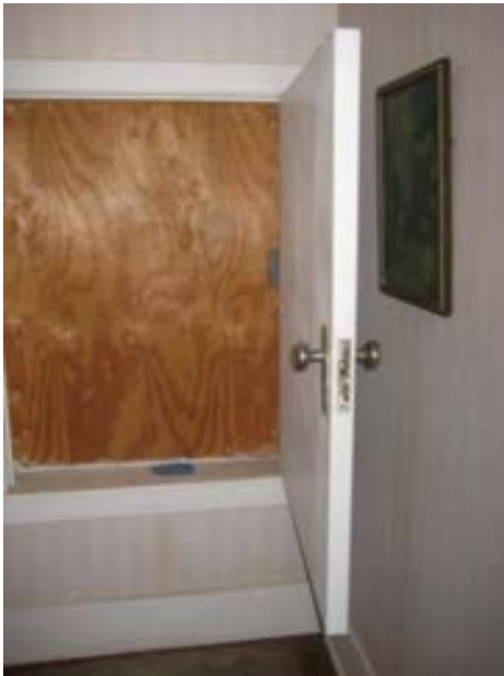
FIGURE 144. Hollow core door and plywood north wall where the exhaust fan used to be. Photograph by BVH, October 16, 2012.
