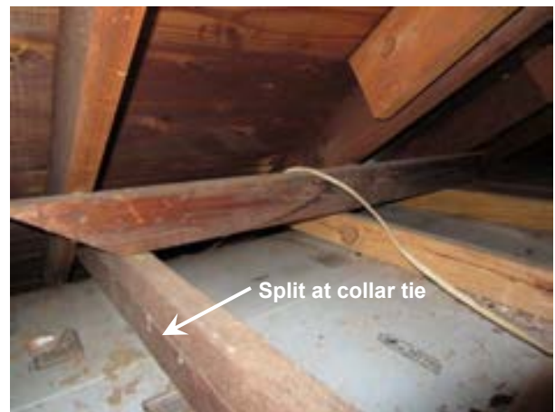
FIGURE 388. Splitting and checking observed at roof collar tie, view looking east. Photograph by WJE, October 17, 2012.
