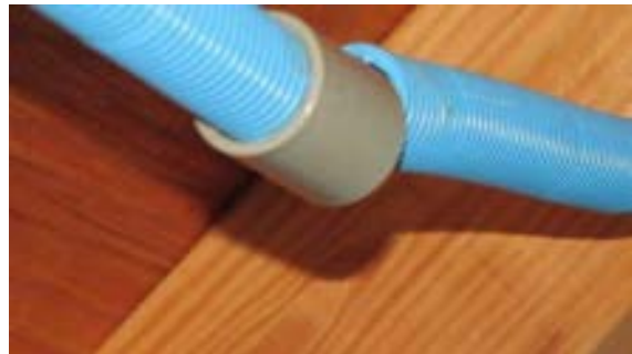
FIGURE 470. Unconnected conduit coupling in the attic of the comfort station. Photograph by Alvine, May 15, 2013.
