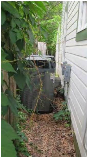
FIGURE 240. Cassidy House condensing unit disconnect switch on the east side of the house. Photograph by Alvine, May 15, 2013.
