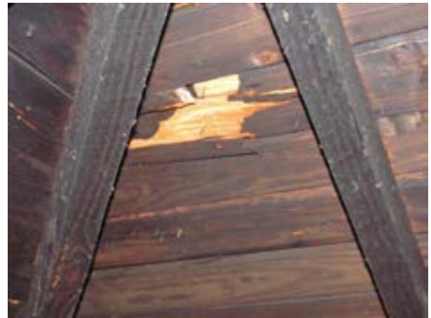
FIGURE 204. Typical area of localized cracking observed at roof planking, view looking southwest. Photograph by WJE, October 16, 2012.
