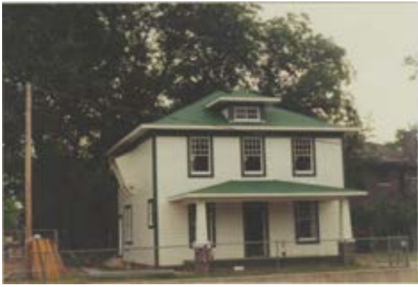
FIGURE 45. Main facade of Cassidy House as the exterior work neared completion, circa fall 1995. Image shows the front porch roof and columns completed. Photo by Terry Huitt from the Clinton Home Restoration Scrapbook prepared by Cromwell Architects, 1997, page 19.
