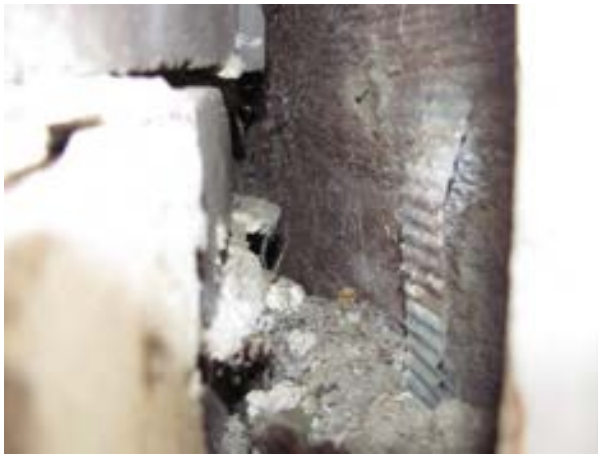
FIGURE 369. Close-up view of wood planking observed behind a the brick veneer at the location shown in Figure 368. The corrugated metal tie at right was intended to secure the veneer. Photograph by WJE, October 16, 2012.
