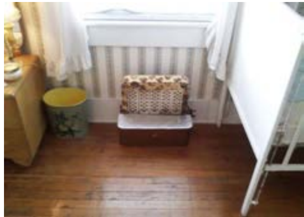
FIGURE 210. Second floor heater at west bedroom 204 of Cassidy House. Photograph by Alvine, May 15, 2013.
