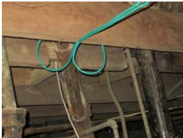
FIGURE 385. One location was observed where a significant portion of the joist had been notched in two locations to accommodate plumbing, view looking west. Photograph by WJE, October 17, 2012.
