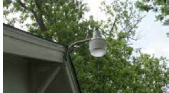
FIGURE 407. Exterior area lighting fixture. Photograph by Alvine, May 15, 2013.
