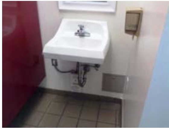
FIGURE 460. Wall-mounted lavatory at women's restroom 102. Photograph by Alvine, May 15, 2013.
