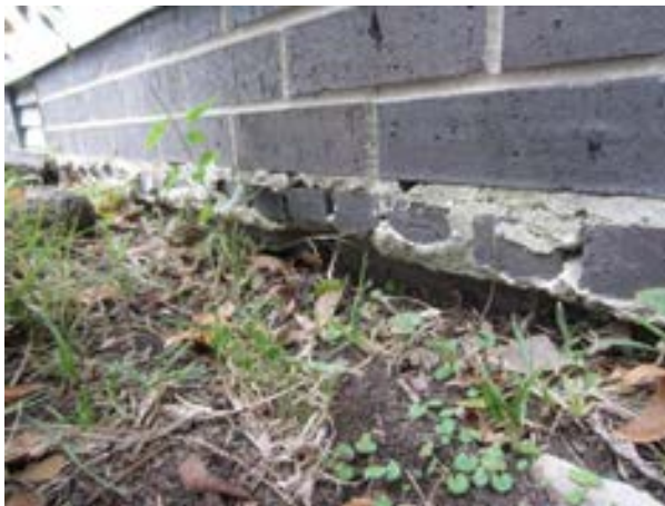
FIGURE 198. Misaligned transition between the new foundation (above) and old foundation bricks (below) observed at the south elevation, view looking northeast. Photograph by WJE, October 16, 2012.
