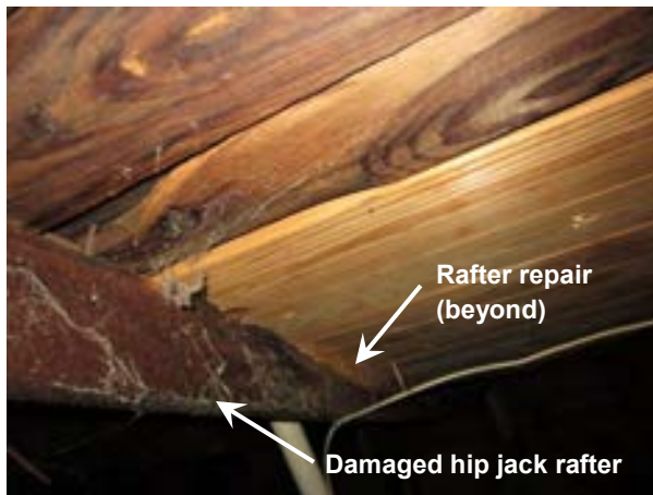
FIGURE 201. Previously repaired hip jack rafter at location of severe section loss, view looking east. Photograph by WJE, October 16, 2012.
