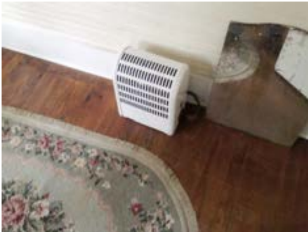
FIGURE 208. Second floor heater at northeast bedroom 202 of the Cassidy House. Photograph by Alvine, May 15, 2013.
