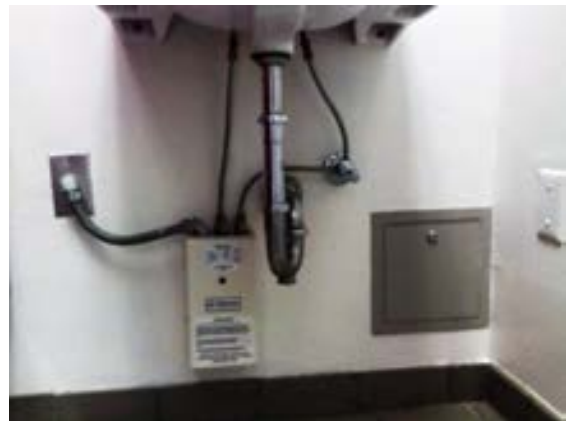
FIGURE 467. Existing 3-kW, tankless, instantaneous water heater and chase access door located below lavatory of women's restroom. Photograph by Alvine, May 15, 2013.
