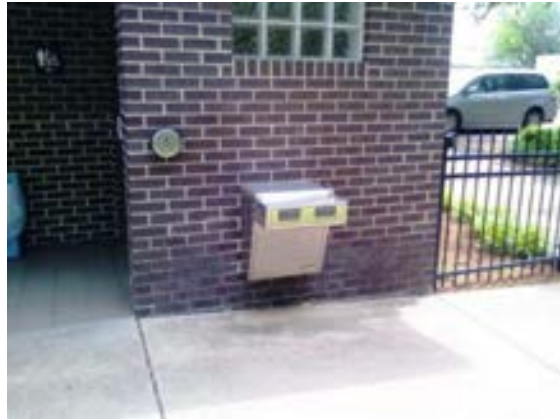
FIGURE 462. Wall-mounted electric water cooler located at west exterior wall of the comfort station. Photograph by Alvine, May 15, 2013.
