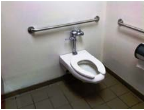
FIGURE 457. Wall-mounted flush valve water closet at men's restroom 103. Photograph by Alvine, May 15, 2013.
