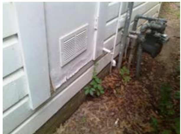
FIGURE 213. Bottom of exterior HVAC closet door indicating lower ventilation grille and door deterioration. Photograph by Alvine, May 15, 2013.
