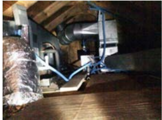
FIGURE 451. HVAC unit (left side of photo) at attic of the . Photograph by Alvine, May 15, 2013.
