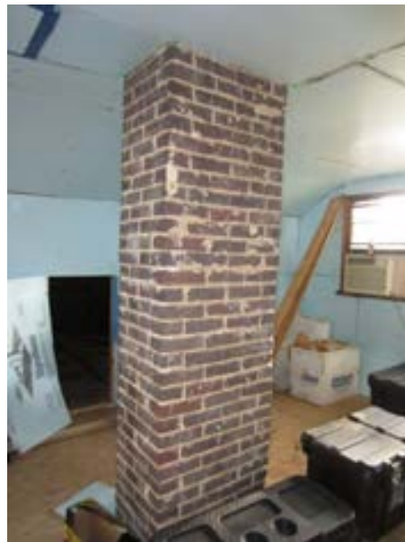
FIGURE 373. Masonry chimney located at the west area of the second floor, view looking southwest. Photograph by WJE, October 16, 2012.
