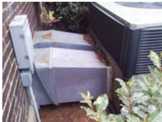
FIGURE 393. Supply and return air ductwork originating at packaged heating and cooling unit serving the visitor center. Photograph by Alvine, May 15, 2013.
