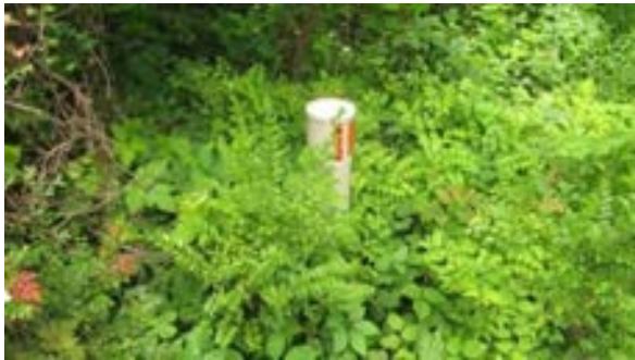
FIGURE 413. Telephone service pedestal. Photograph by Alvine, May 15, 2013.
