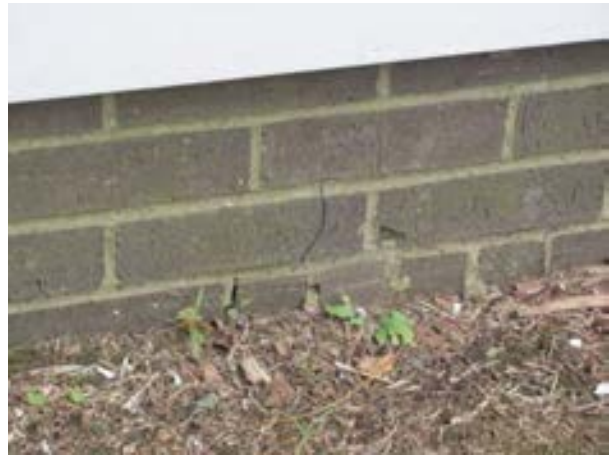
FIGURE 78. Step cracking is present in the brick masonry foundation. Photograph by WJE, October 16, 2012.
