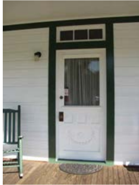
FIGURE 68. The main door to the house on the west elevation. The three-light transom is an original element dating to the period of significance. Photograph by WJE, October 15, 2012.
