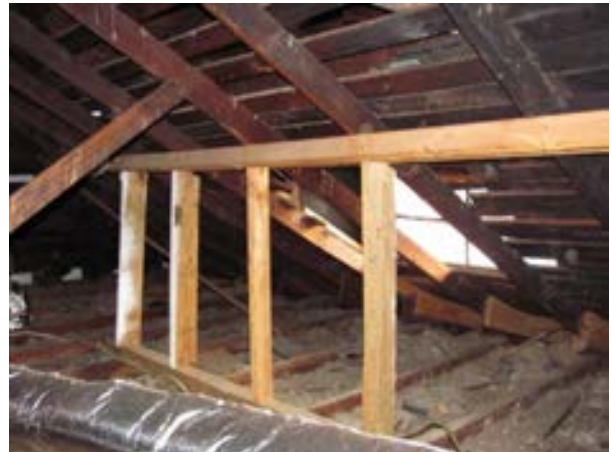
FIGURE 193. Common and hip jack rafters, which continue through the dormer opening at the west elevation, are supported on a non-original 2 by 4 knee wall frame, view looking southwest. Photograph by WJE, October 16, 2012.
