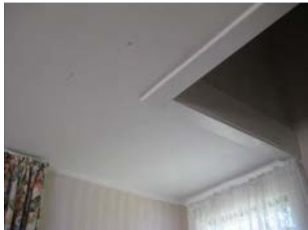
FIGURE 91. Ceiling cornice and trim at stair opening, replaced at time of the 1996 work, looking northwest in the living room. Photograph by BVH, October 16, 2012.
