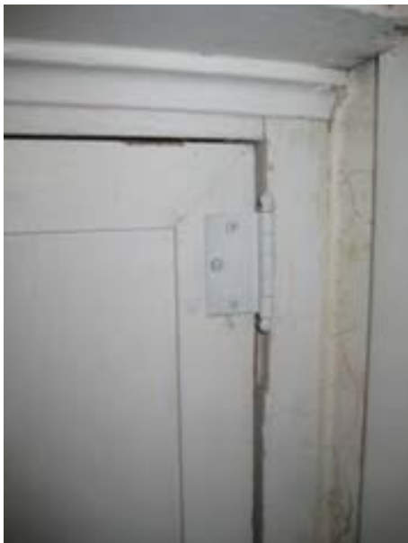
FIGURE 120. Newer face hinges, and evidence where previous hinges were located evidenced by the mortise in the frame below. Photograph by BVH, October 16, 2012.
