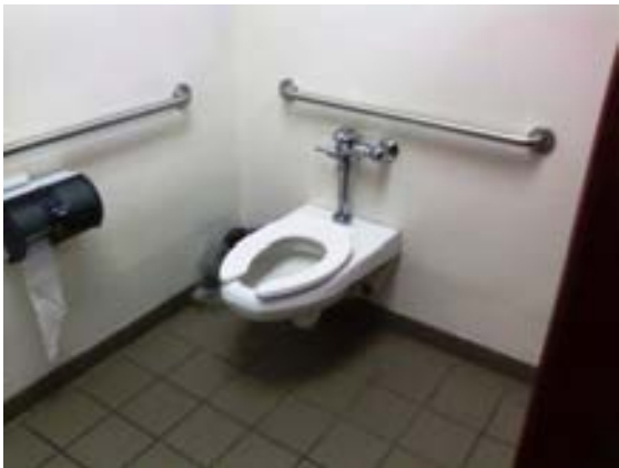
FIGURE 459. Wall-mounted flush valve water closet (typ-2) at women's restroom 102. Photograph by Alvine, May 15, 2013.
