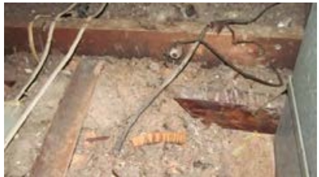
FIGURE 242. Original inactive knob and tube wiring and nonmetallic sheathed cable in attic. Photograph by Alvine, May 15, 2013.
