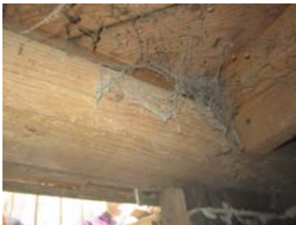
FIGURE 184. Typical joist support condition notched over a 6x8 perimeter beam with a 2 by 4 ledger, view looking east. Photograph by WJE, October 16, 2012.
