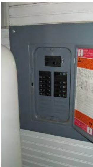
FIGURE 236. Cassidy house electrical load center. Photograph by Alvine, May 15, 2013.
