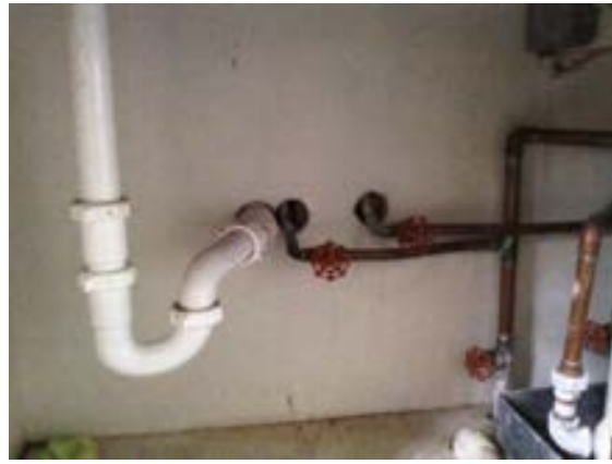
FIGURE 228. Cassidy House under-cabinet waste and water supply piping serving kitchen counter-mounted sink above. Photograph by Alvine, May 15, 2013.
