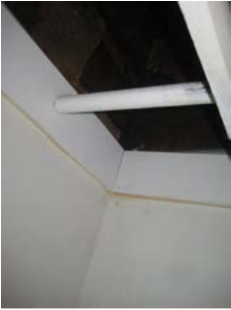
FIGURE 174. North plywood wall within the closet from the floor to a level above the door, painted white. Photograph by BVH, October 16, 2012.
