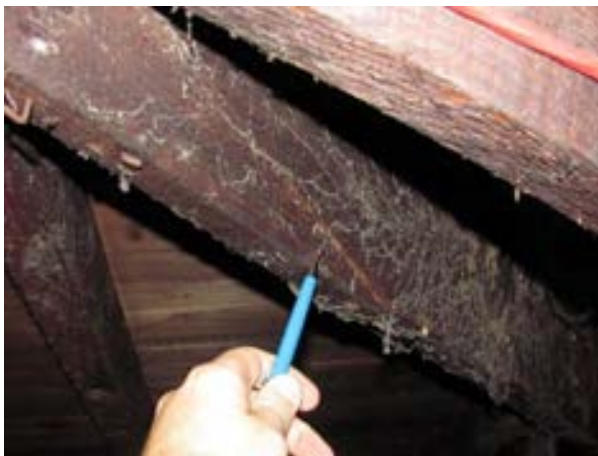
FIGURE 203. Northeast hip rafter with a break through the entire cross-section, view looking northeast. Photograph by WJE, October 16, 2012.
