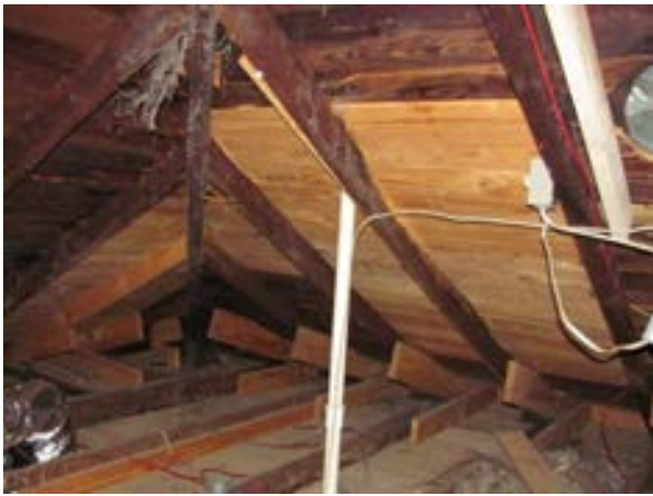
FIGURE 194. Northeast corner of the attic where portions of the roof and soffit framing were previously repaired or replaced, view looking northeast. Photograph by WJE, October 16, 2012.
