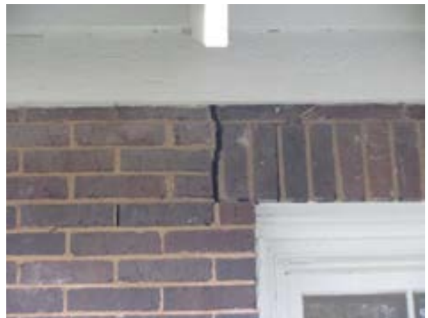
FIGURE 272. Cracking at the head of a window. Photograph by WJE, October 16, 2012.
