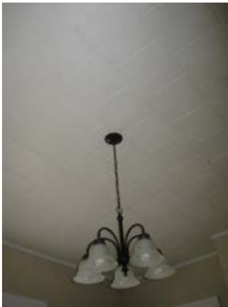
FIGURE 332. Chandelier and ceiling tile assembly, looking northwest. Photograph by BVH, October 16, 2012.
