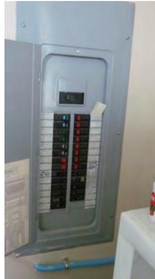
FIGURE 398. Electrical panel in office 108. Photograph by Alvine, May 15, 2013.
