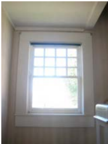
FIGURE 100. Small window at stair landing, north wall of living room. Photograph by BVH, October 16, 2012.
