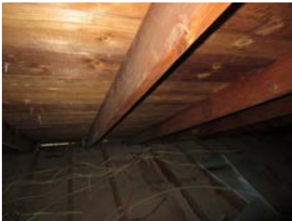
FIGURE 375. Roof rafters bear on the top plate of the exterior bearing walls, but do not coincide with first floor ceiling joists. Looking south. Photograph by WJE, October 17, 2012.
