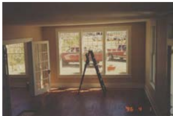
FIGURE 57. View of interior living room looking south showing the room near completion, April 1, 1996. Interior finishes are in place, new windows have been installed, new wood trim has been installed and painted, and the floor refinshed. Photo by Terry Huitt from the Clinton Home Restoration Scrapbook prepared by Cromwell Architects, 1997, page 31.
