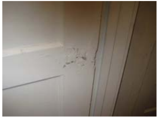
FIGURE 127. Back porch door located in the northeast corner of the kitchen. Note that the panels are not raised, and the infilled door knob at the hinge side of the door. Photograph by BVH, October 16, 2012.
