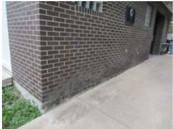
FIGURE 423. Staining observed at the concrete edge and the first six courses of brick at the west elevation. Photograph by WJE, October 17, 2012.
