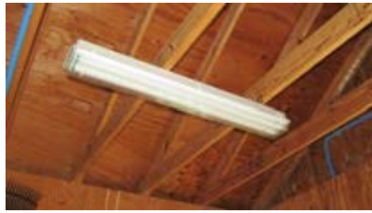
FIGURE 478. Storage Room lighting. Photograph by Alvine, May 15, 2013.
