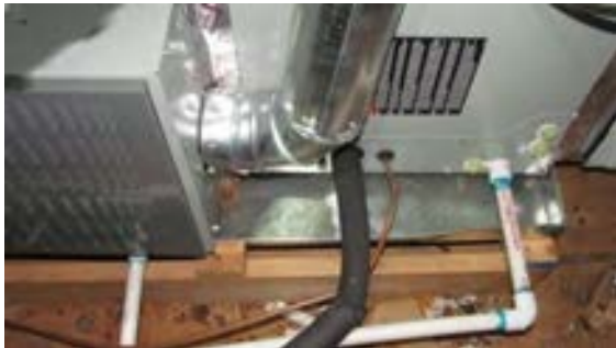
FIGURE 218. Horizontal furnace and secondary drain pan located in the attic. Photograph by Alvine, May 15, 2013.
