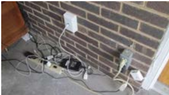
FIGURE 414. Communication wiring and power wiring near reception desk in entry 101. Photograph by Alvine, May 15, 2013.
