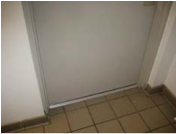
FIGURE 435. The steel outswing door of the women's room, looking south. Photograph by BVH, October 16, 2012.
