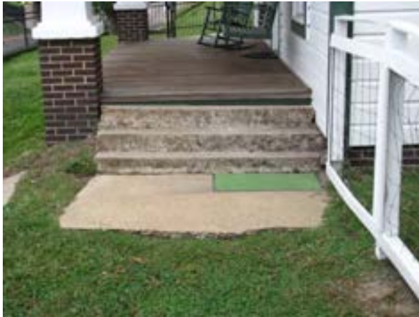
FIGURE 74. A view of the concrete slab and concrete steps leading to the front porch. These concrete elements date to the period of significance. Photograph by WJE, October 16, 2012.
