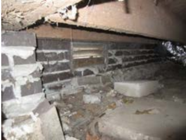
FIGURE 180. The brick masonry foundation consists of 1-foot-square piers and a one-wythe perimeter wall, which were rebuilt above grade during the 1995 work, view looking southwest. Photograph by WJE, October 16, 2012.
