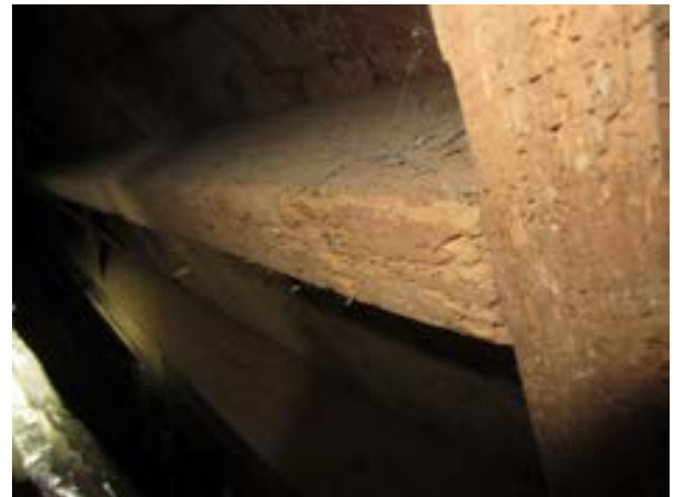
FIGURE 199. Evidence of termite damage was observed at the first floor framing, view looking northwest. Photograph by WJE, October 16, 2012.
