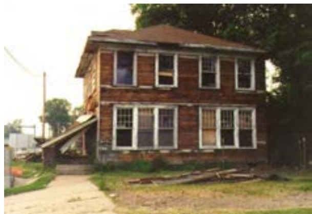
FIGURE 39. Photo showing the south side wall during renovation, with the front of the house at left, circa June 1995. The image shows the partially demolished front porch, with the original brick column bases intact. The original windows were still in place in this image, however the exterior siding had been removed. Also note the pile of debris in the yard. Photo by Terry Huitt from the Clinton Home Restoration Scrapbook prepared by Cromwell Architects, 1997, page 16.
