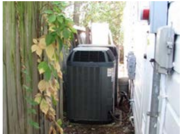
FIGURE 76. A view of the mechanical equipment on the south end of the east elevation. Photograph by WJE, October 15, 2012.
