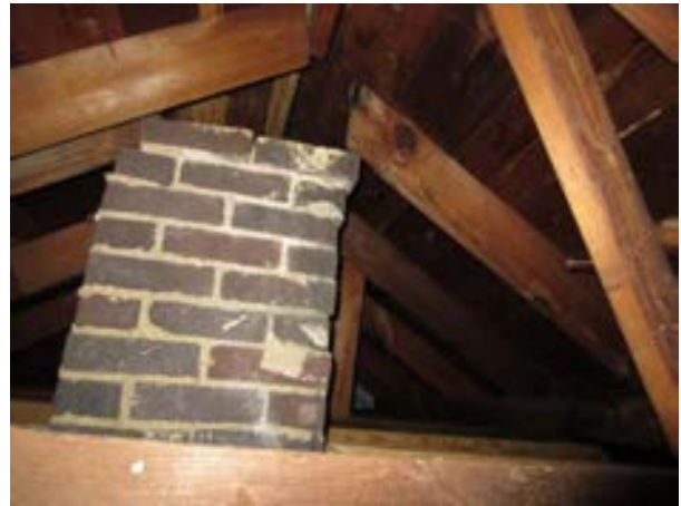
FIGURE 376. Supplemental 2 by 4 framing to support roof framing where masonry chimney was cut short, view looking west. Photograph by WJE, October 17, 2012.
