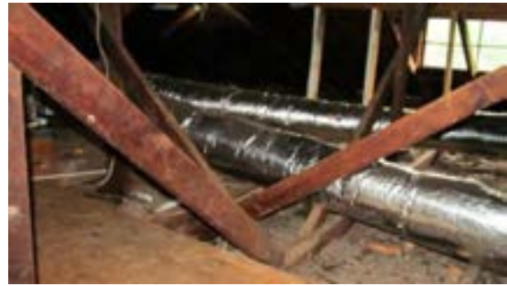
FIGURE 219. Insulated supply air ductwork, located in attic, serving second floor of Cassidy House. Photograph by Alvine, May 15, 2013.
