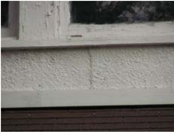
FIGURE 274. A repaired crack in the plaster at a dormer. Photograph by WJE, October 16, 2012.
