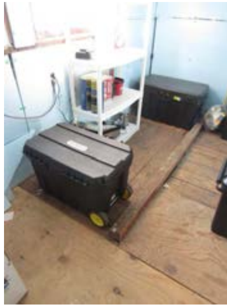
FIGURE 372. Two 2 by 10s framed north-south at the west end of the second floor, view looking northwest. Photograph by WJE, October 16, 2012.
