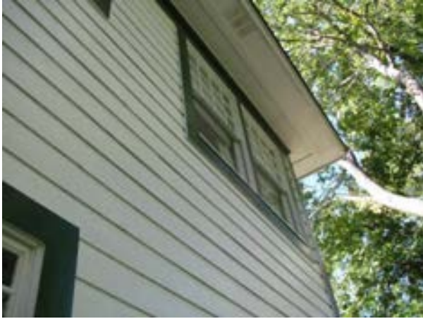
FIGURE 77. The set of double-hung windows at the north end of the east elevation. Photograph by WJE, October 15, 2012.
