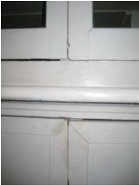
FIGURE 119. Two types of door construction; the lower doors are replacements. Photograph by BVH, October 16, 2012.
