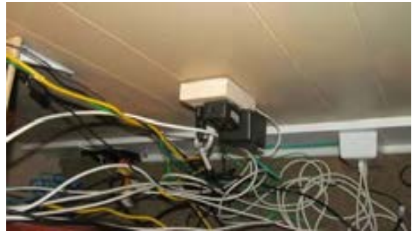
FIGURE 415. Communication wiring and power in office room 106, looking down the west wall. Photograph by Alvine, May 15, 2013.
