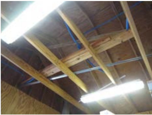
FIGURE 447. 2 by 4 gable end wall braced by 2 by 4 and 2 by 6 wood members framing over the roof rafter horizontal ties. Looking north. Photograph by WJE, October 17, 2012.
