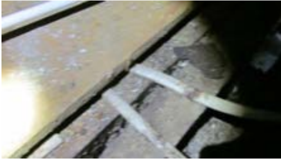
FIGURE 239. Cassidy House showing pinched nonmetallic sheathed cable under wood platform. Photograph by Alvine, May 15, 2013.
