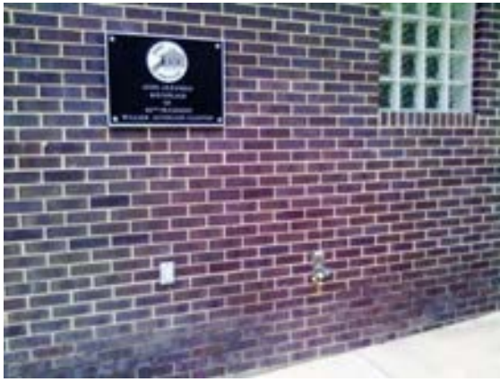
FIGURE 463. Wall hydrant located at west exterior wall of the comfort station. Photograph by Alvine, May 15, 2013.
