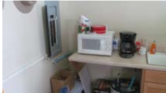
FIGURE 396. Visitor center electrical panel in office 108 showing insufficient working space clearance. An electric water heater is located below the counter the at first floor office. Photograph by Alvine, May 15, 2013.
