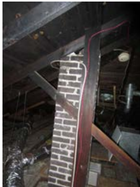
FIGURE 200. Roof framing was discolored and exhibited surface charring due to the 1992 fire at the second floor. Note, the discoloration is mostly limited to the upper portion of the attic, view looking west. Photograph by WJE, October 16, 2012.
