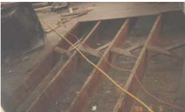
FIGURE 186. Interior of the west bedroom, February 5, 1996. Removal of the fire-damaged finish floor exposed the structural joists, bridging, and plank sheathing of the first floor ceiling below. Photo by Terry Huitt from the Clinton Home Restoration Scrapbook prepared by Cromwell Architects, 1997, page 27.
