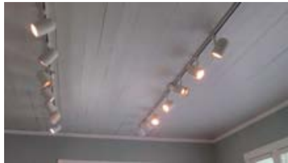
FIGURE 401. Exhibit 103 track lighting. Photograph by Alvine, May 15, 2013.
