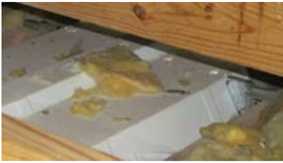
FIGURE 474. Exposed lighting fixture in the attic. Photograph by Alvine, May 15, 2013.
