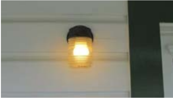
FIGURE 249. Cassidy House front porch lighting fixture. Photograph by Alvine, May 15, 2013.
