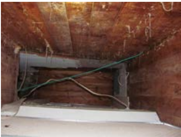
FIGURE 367. Wood sheathing at interior partition walls, viewed above the suspended ceiling of the first floor corridor, view looking west. Photograph by WJE, October 17, 2012.
