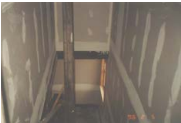
FIGURE 52. Stairwell to second floor, February 5, 1996, showing new gypsum board. Photo by Terry Huitt from the Clinton Home Restoration Scrapbook prepared by Cromwell Architects, 1997, page 26.
