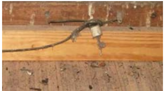
FIGURE 241. Original inactive knob and tube wiring in attic. Photograph by Alvine, May 15, 2013.
