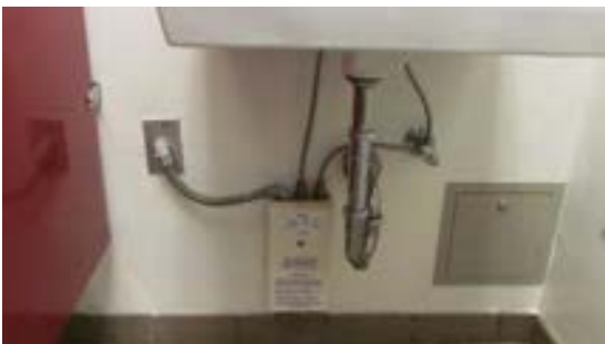
FIGURE 473. Instantaneous electric water heater in toilet room. Photograph by Alvine, May 15, 2013.
