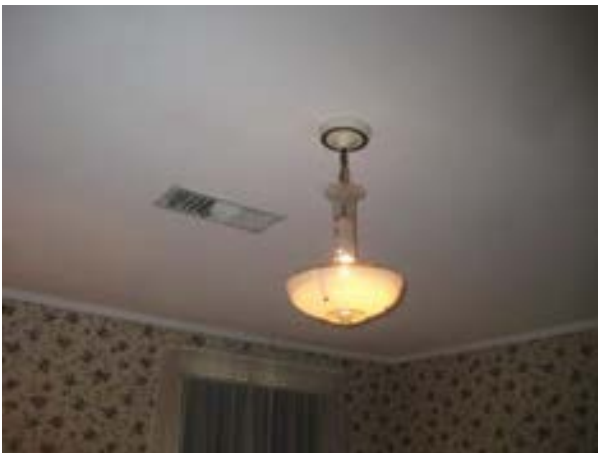
FIGURE 170. Ceiling and light fixture in bedroom 205, looking south. Photograph by BVH, October 16, 2012.
