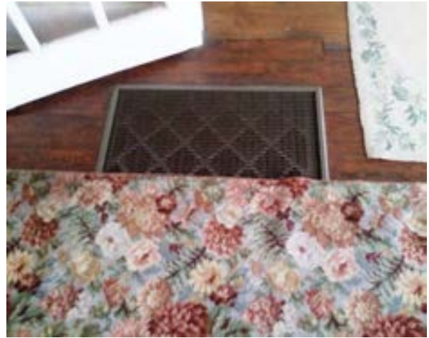
FIGURE 205. Return air filter grille for the first floor furnace system located in the living room floor (living room 101). Photograph by Alvine, May 15, 2013.
