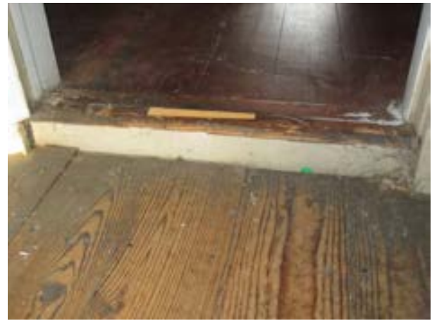
FIGURE 370. Location where floor framing steps down from 2 by 10 joists to 2 by 6 joists at the west area of the second floor. A similar condition exists at the east area, view looking east. Photograph by WJE, October 16, 2012.
