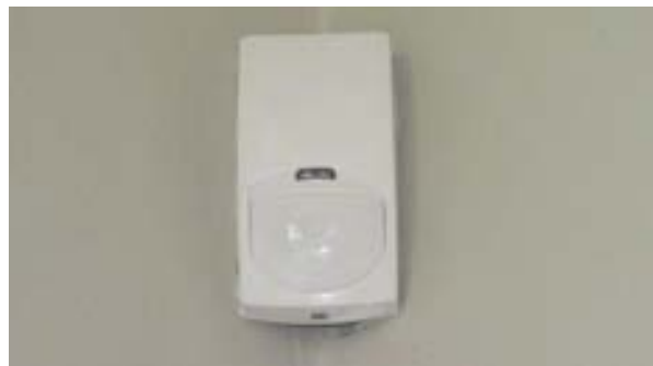
FIGURE 412. Intrusion alarm motion detector. Photograph by Alvine, May 15, 2013.
