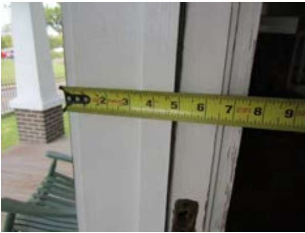
FIGURE 185. Perimeter wall measuring approximately 7-1/2 inches at the first floor indicates stud wall framing, view looking north. Photograph by WJE, October 17, 2012.
