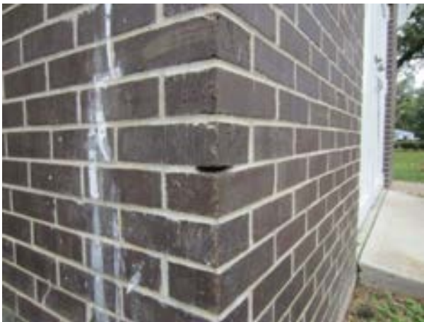
FIGURE 422. Missing mortar at northeast corner masonry joint. Looking southwest. Photograph by WJE, October 17, 2012.
