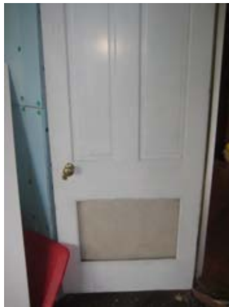
FIGURE 351. Three panel door with bottom panel replaced with air circulation grille, facing west. Photograph by BVH, October 16, 2012.
