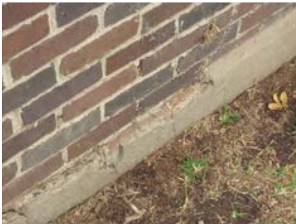
FIGURE 269. An instance of cracking at the cast concrete foundation. Photograph by WJE, October 16, 2012.
