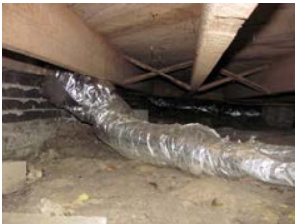
FIGURE 183. First floor framing consists of 2 by 8 joists at 20 inches on center with bridging at midspan and diagonal tongue-and-groove decking, view looking west. Photograph by WJE, October 16, 2012.
