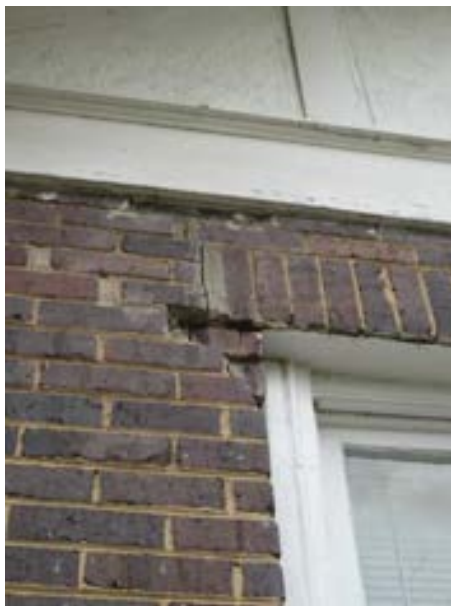
FIGURE 380. Typical step cracking and displacement observed at the masonry facade, view looking west. Photograph by WJE, October 17, 2012.
