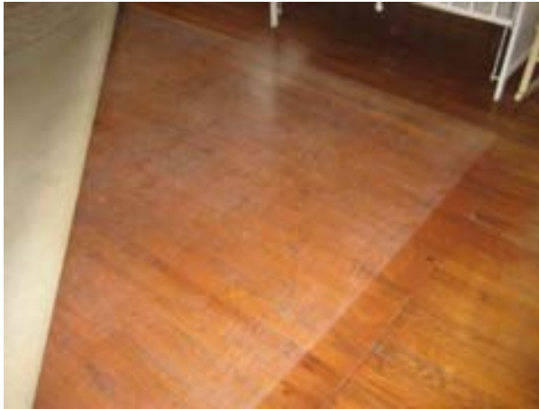
FIGURE 158. The continuous seam in the floor denotes the replacement portion of the floor due to the fire. The original flooring is at right, looking west. Photograph by BVH, October 16, 2012.
