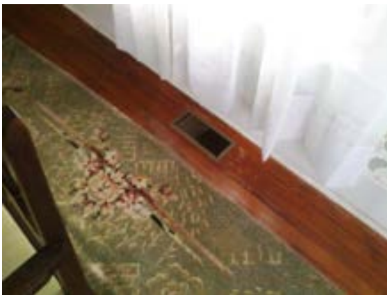
FIGURE 216. Floor supply air register in dining room 102 of the Cassidy House (typical of all first floor supply air registers). Photograph by Alvine, May 15, 2013.
