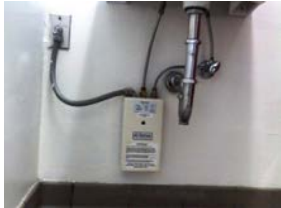
FIGURE 466. Existing 3-kW, tankless, instantaneous water heater located below lavatory of men's restroom. Photograph by Alvine, May 15, 2013.
