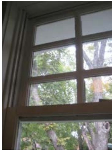
FIGURE 156. Bathroom window located on the east wall of the room. Photograph by BVH, October 16, 2012.
