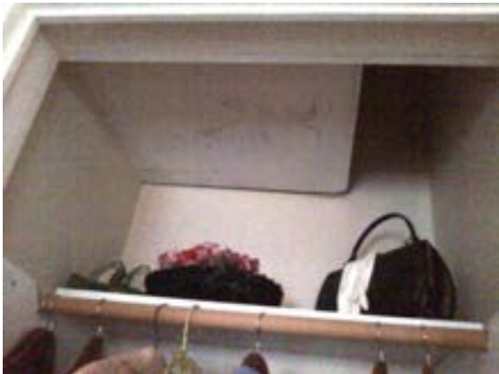
FIGURE 222. Return air duct connected to hallway return grille, located in the closet of southeast bedroom 205 of Cassidy House. Photograph by Alvine, May 15, 2013.
