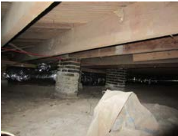
FIGURE 364. Additional masonry foundation piers were observed supporting the midspan of select first floor joists, view looking northeast. Photograph by WJE, October 17, 2012.
