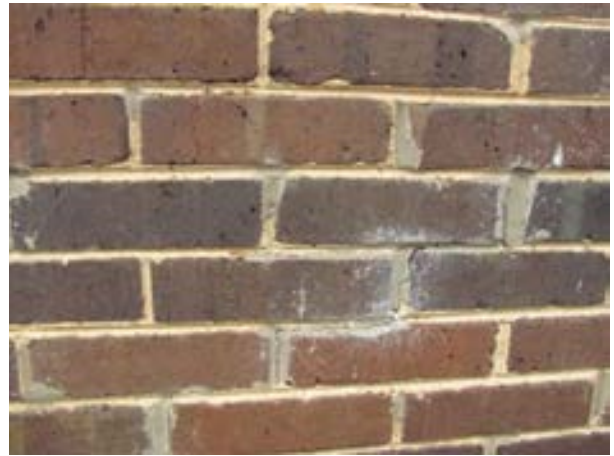
FIGURE 271. A view of stepped cracking on the field of an exterior wall. Photograph by WJE, October 16, 2012.
