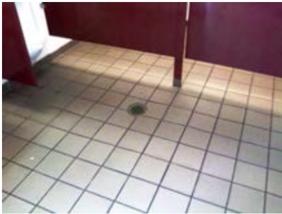
FIGURE 464. Floor drain in men's restroom. Photograph by Alvine, May 15, 2013.
