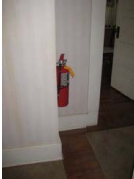
FIGURE 140. West wall assembly of the second floor hall. Photograph by BVH, October 16, 2012.
