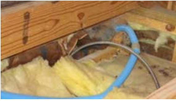
FIGURE 471. Electrical nonmetallic conduit and metal clad cable in the attic of the comfort station. Photograph by Alvine, May 15, 2013.
