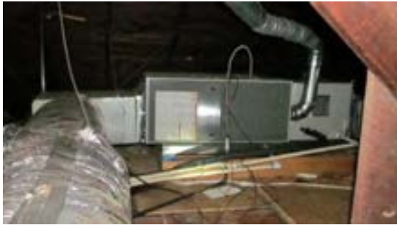
FIGURE 217. Horizontal furnace located in the attic, serving the second floor of Cassidy House. Photograph by Alvine, May 15, 2013.
