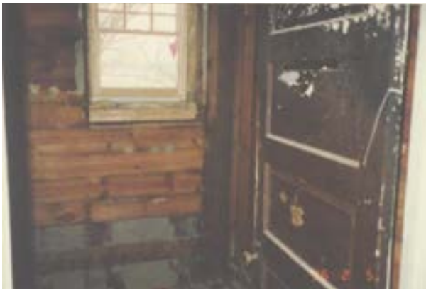
FIGURE 51. Interior of the bathroom, February 5, 1996. All interior finishes and fixtures have been removed. Photo by Terry Huitt from the Clinton Home Restoration Scrapbook prepared by Cromwell Architects, 1997, page 25.
