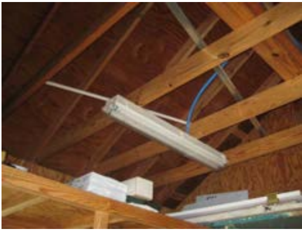
FIGURE 427. Exposed roof structure in the maintenance storage room, looking south. Photograph by BVH, October 16, 2012.
