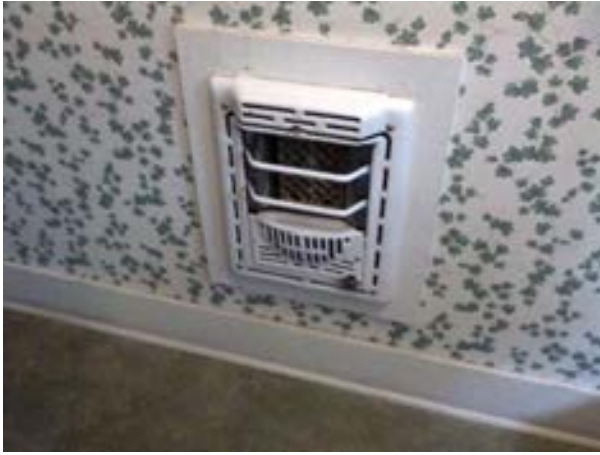
FIGURE 207. Second floor wall-located heater in bathroom 203 of the Cassidy House. Photograph by Alvine, May 15, 2013.
