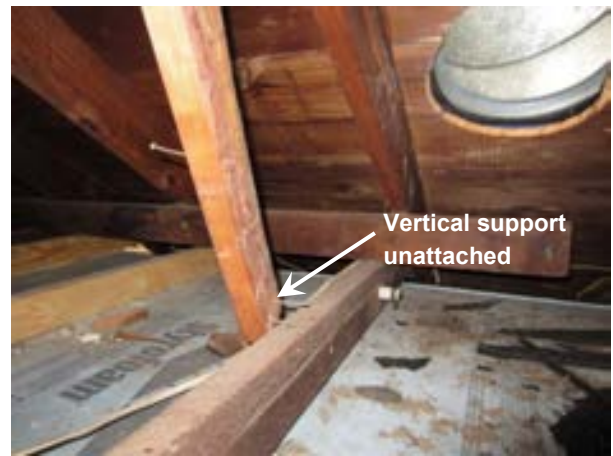
FIGURE 387. Supplemental vertical support assumed to be installed during chimney modification is detached at the collar tie connection, view looking north. Photograph by WJE, October 17, 2012.
