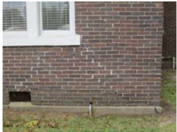
FIGURE 379. Step cracking and displacement in excess of 1 inch typically noted at the masonry foundation and facade, view looking south. Photograph by WJE, October 17, 2012.
