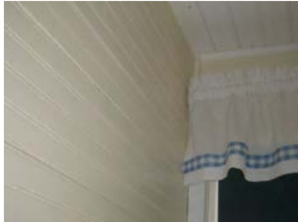
FIGURE 145. Wall assembly of the west wall in bedroom 202. Photograph by BVH, October 16, 2012.
