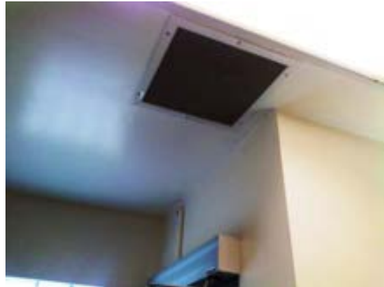
FIGURE 455. Ceiling exhaust air grille at women's restroom 102 of the comfort station (men's restroom 103 grille is similar). Photograph by Alvine, May 15, 2013.
