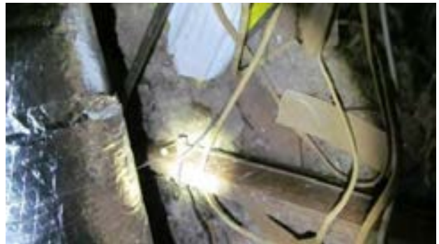
FIGURE 243. Inactive knob and tube wiring and incorrectly supported nonmetallic sheathed cable. Photograph by Alvine, May 15, 2013.
