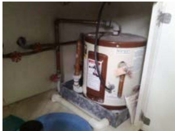
FIGURE 229. Cassidy House under-cabinet electric water heater serving kitchen counter-mounted sink. Photograph by Alvine, May 15, 2013.
