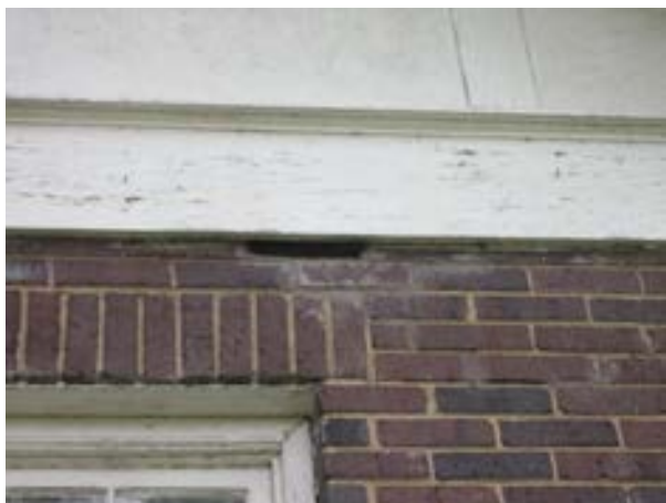
FIGURE 381. Missing brick at the west elevation, view looking east. Photograph by WJE, October 17, 2012.
