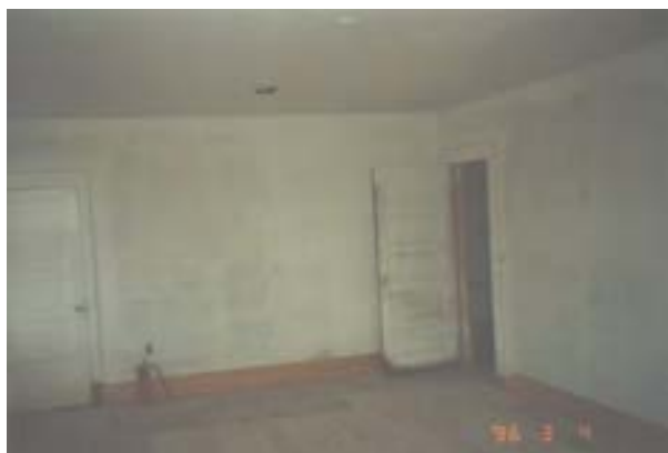
FIGURE 56. Interior of the west bedroom, March 4, 1996. New gypsum board finishes have been primed, and fire-damaged portions of the hardwood floor have been replaced. Photo by Terry Huitt from the Clinton Home Restoration Scrapbook prepared by Cromwell Architects, 1997, page 30.
