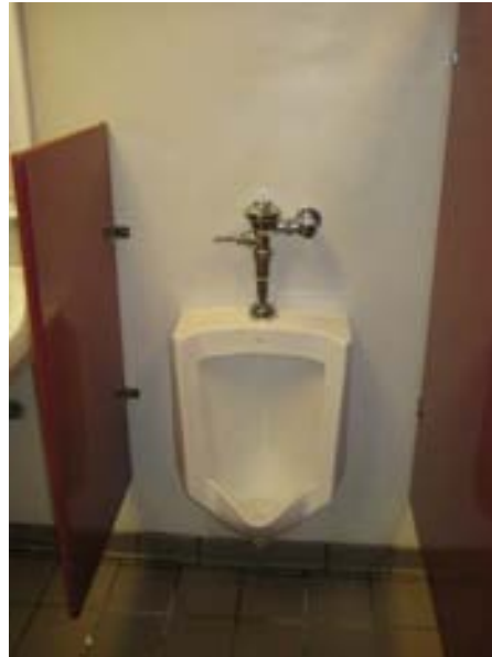
FIGURE 438. Men's room urinal on the north wall. Photograph by BVH, October 16, 2012.
