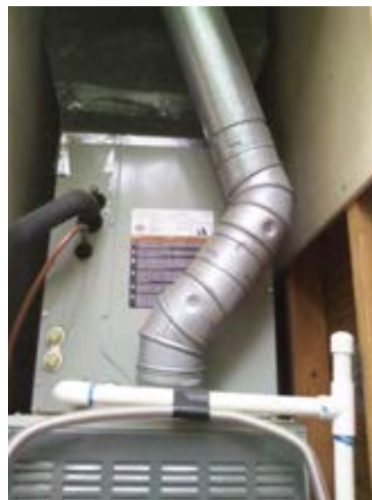
FIGURE 214. Furnace in Clinton House exterior equipment closet. Photograph by Alvine, May 15, 2013.
