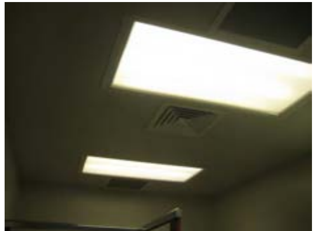
FIGURE 434. Ceiling with mechanical openings and fluorescent light fixtures, looking east. Photograph by BVH, October 16, 2012.
