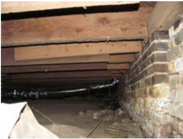
FIGURE 366. 2 by 8 sister joist retrofits observed at the south end of first floor joists, toenailed to the perimeter ledger beam, view looking east. Photograph by WJE, October 17, 2012.
