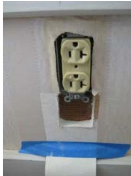
FIGURE 87. Material assembly of wall construction, showing the horizontal half-lap wood wall boards behind the gypsum board, located below the south window of the living room. Photograph by BVH, October 16, 2012.
