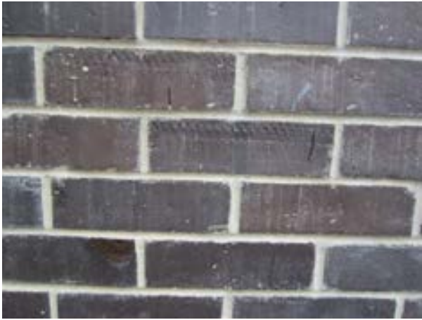
FIGURE 421. Typical location where bricks exhibit vertical splitting, a likely manufacturing defect, was observed with no signs of related distress in the mortar. Looking north. Photograph by WJE, October 17, 2012.
