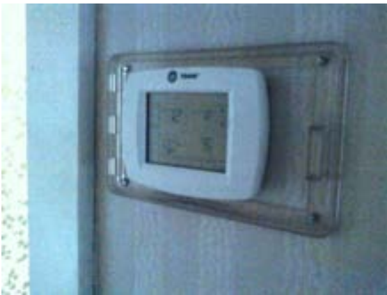
FIGURE 225. Cassidy House second floor HVAC system control thermostat located in hallway 201. Photograph by Alvine, May 15, 2013.
