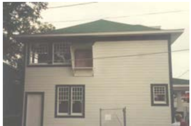
FIGURE 44. View from the north as the exterior work neared completion, circa fall 1995. Photo by Terry Huitt from the Clinton Home Restoration Scrapbook prepared by Cromwell Architects, 1997, page 18.
