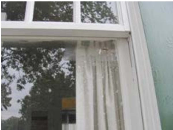
FIGURE 80. Cracked window glass was observed in several locations. Photograph by WJE, October 16, 2012.
