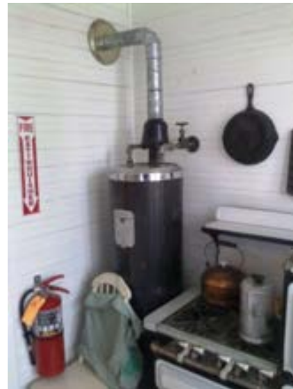
FIGURE 233. Existing non-functional water heater, flue duct, and water supply piping at first floor kitchen 201 of Cassidy House. Photograph by Alvine, May 15, 2013.
