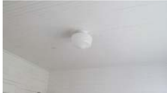
FIGURE 245. Kitchen 104 lighting fixture. Photograph by Alvine, May 15, 2013.
