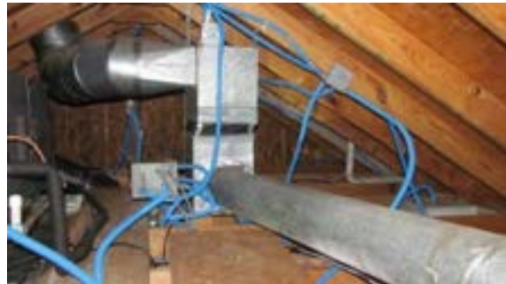
FIGURE 469. Incorrectly routed and unsupported conduit in the attic of the comfort station. Photograph by Alvine, May 15, 2013.
