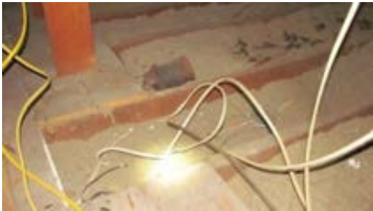
FIGURE 400. Electrical wiring in attic with incorrectly routed and unsupported cables. Photograph by Alvine, May 15, 2013.
