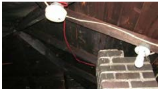
FIGURE 206. In the attic of the Cassidy House, the existing chimney has been removed to below the level of the attic ceiling. Also note the existing lighting fixture. Photograph by Alvine, May 15, 2013.
