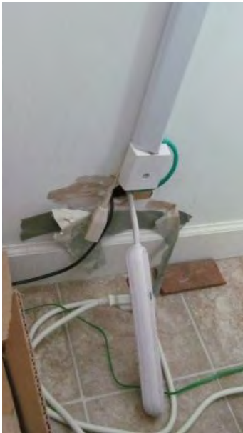
FIGURE 409. Electrical cord in room 107, routed through wall into room 106. Photograph by Alvine, May 15, 2013.
