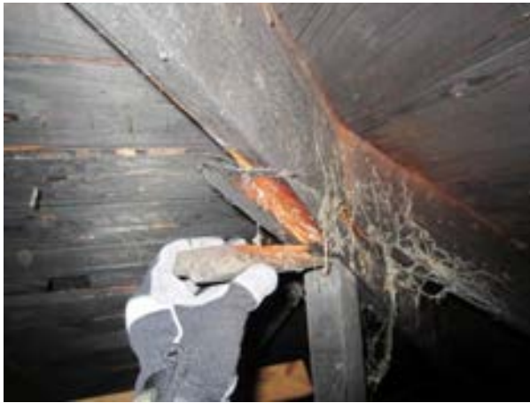
FIGURE 202. Split and displacement observed at the northwest hip rafter. Note, a post repair had been implemented prior to the 1992 fire. Looking northwest. Photograph by WJE, October 17, 2012.
