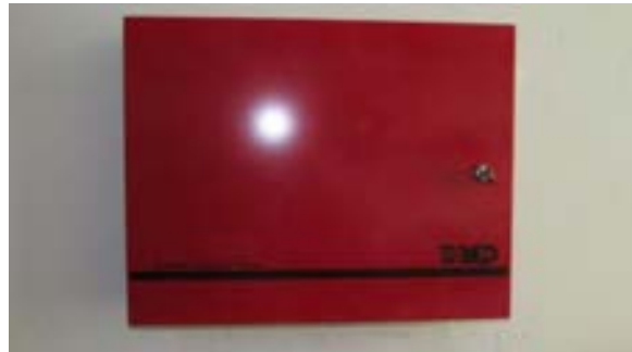
FIGURE 411. Intrusion alarm panel in the copy machine room. Photograph by Alvine, May 15, 2013.
