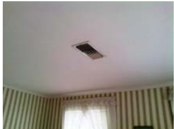
FIGURE 220. Ceiling-located supply air diffuser at second floor west bedroom 204 of Cassidy House (typical of all second floor rooms). Photograph by Alvine, May 15, 2013.
