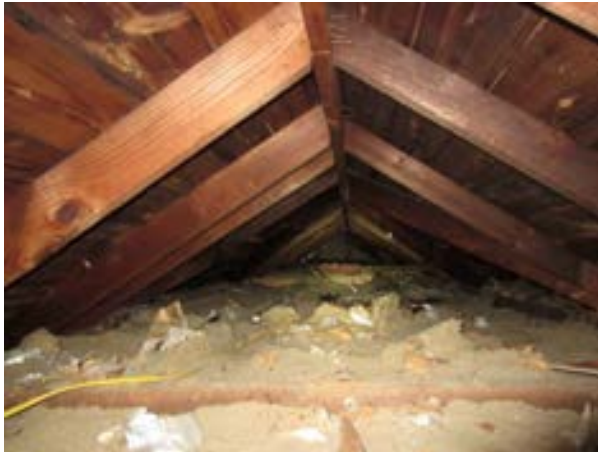
FIGURE 374. Typical gable roof framing with 2 by 6 common rafters framing into a 2 by 6 ridge and 2 by 4 collar ties, view looking east. Photograph by WJE, October 17, 2012.
