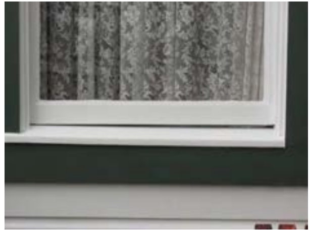
FIGURE 81. View of a window that is unable to fully close due to the settlement of the house. Photograph by WJE, October 16, 2012.
