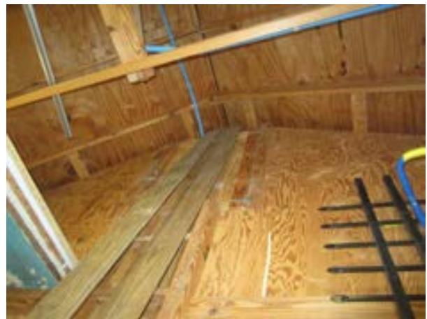
FIGURE 446. Condition noted at the fifth rafter where 2x4 purlins replace the horizontal tie due to a conflict at the plywood wall hatch. Looking south. Photograph by WJE, October 17, 2012.
