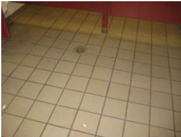
FIGURE 440. ceramic tile floor in the men's room looking east. Photograph by BVH, October 16, 2012.
