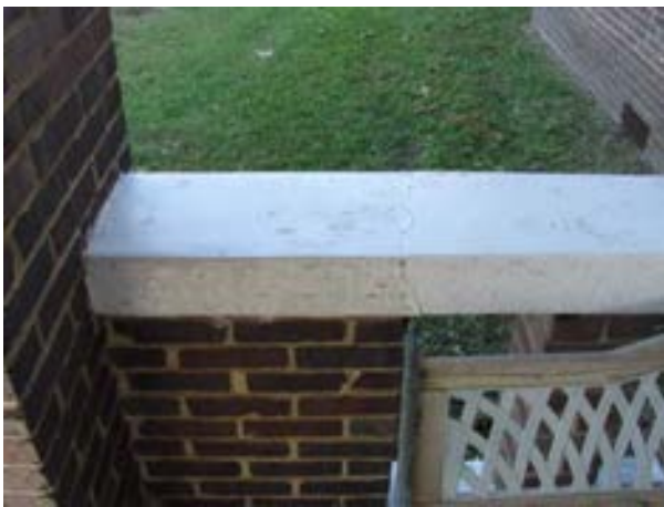
FIGURE 275. A crack in the precast concrete at the north porch. Photograph by WJE, October 15, 2012.
