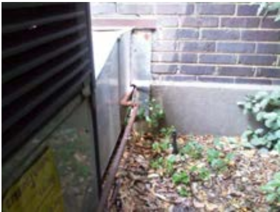
FIGURE 395. Gas piping exiting the visitor center south crawlspace wall to grade-mounted packaged heating and cooling unit. Photograph by Alvine, May 15, 2013. M32
