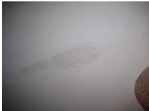
FIGURE 163. Water staining on the ceiling. Photograph by BVH, October 16, 2012.
