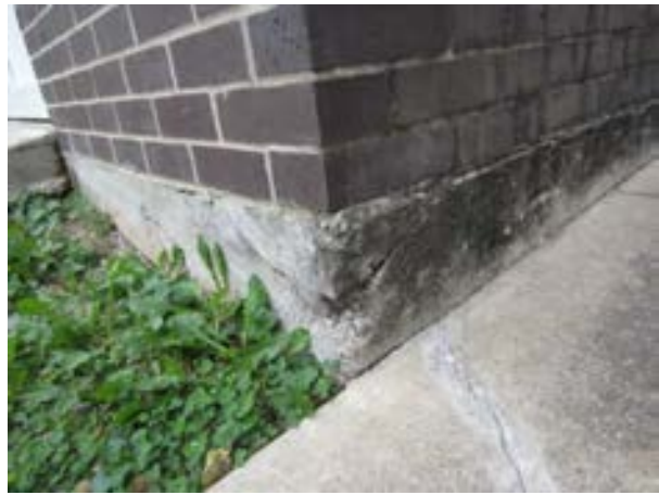
FIGURE 448. Cracking and spalling at northwest corner of concrete slab-on-grade. Looking southeast. Photograph by WJE, October 17, 2012.
