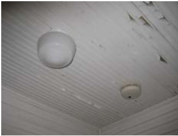
FIGURE 137. Light fixture and peeling paint of the ceiling of the back porch. Photograph by BVH, October 16, 2012.
