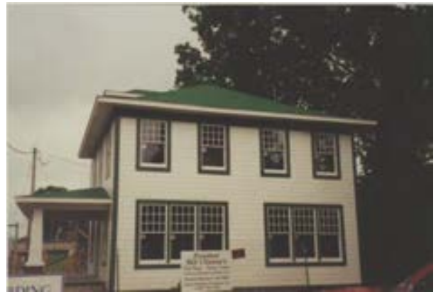
FIGURE 42. View from the southwest as the exterior work neared completion, circa fall 1995. Image shows the new siding completely installed, new windows, and front porch reconstructed. Photo by Terry Huitt from the Clinton Home Restoration Scrapbook prepared by Cromwell Architects, 1997, page 18.
