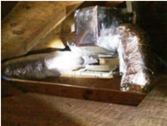
FIGURE 453. Exhaust ductwork and in-line exhaust fan, located in attic, serving restrooms of the comfort station. Photograph by Alvine, May 15, 2013.
