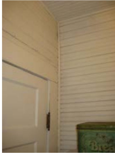
FIGURE 136. The beadboard on the wall above the door on the north wall is original, but the beadboard on the east wall dates from the 1996 work. Photograph by BVH, October 16, 2012.
