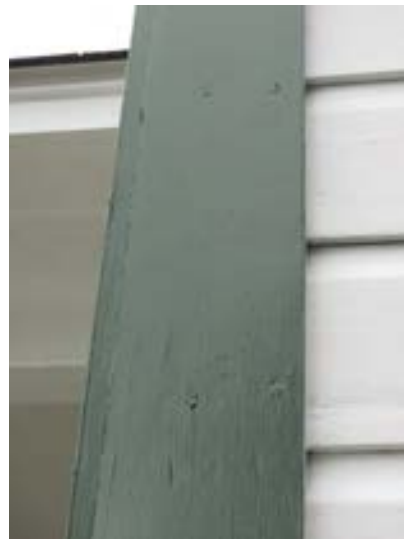
FIGURE 83. A view of an exterior wood trim element that was minimally prepared prior to painting. Photograph by WJE, October 16, 2012.
