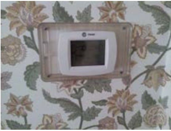
FIGURE 224. Cassidy House first floor HVAC system control thermostat located in dining room 102. Photograph by Alvine, May 15, 2013.
