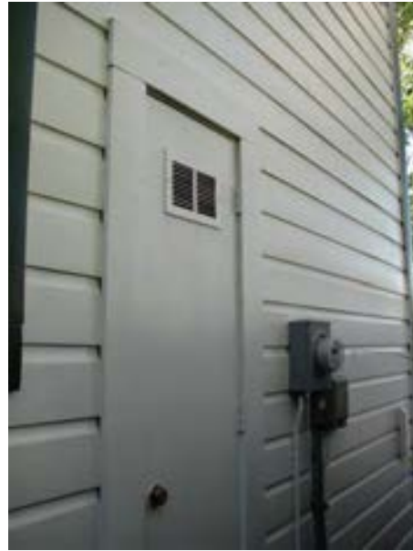
FIGURE 75. A view of the mechanical closet door and the building's gas and electric meters. Photograph by WJE, October 15, 2012.
