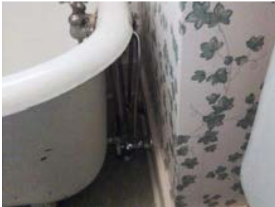
FIGURE 232. Waste and water supply piping serving bathtub at Cassidy House second floor bathroom. Photograph by Alvine, May 15, 2013.
