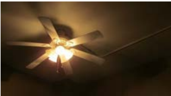
FIGURE 405. Ceiling fan/ light in office 106. Photograph by Alvine, May 15, 2013.
