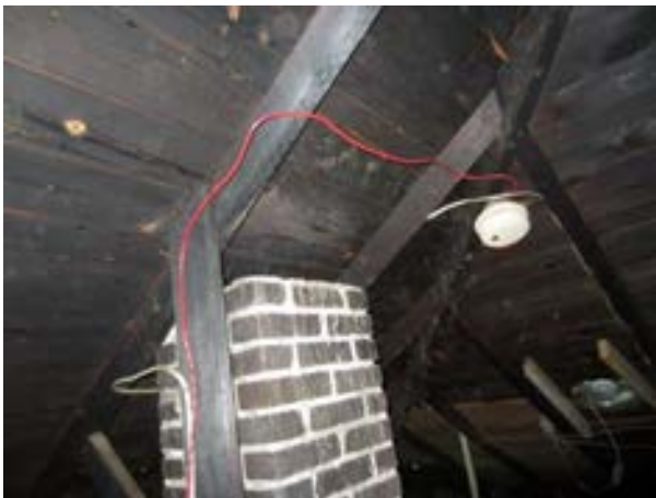
FIGURE 195. A 16-inch-square brick chimney was noted to have been cut below the roofline prior to the 1992 fire, evidenced by the charred wood planking directly above it, view looking northeast. Photograph by WJE, October 16, 2012.
