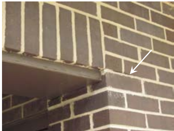
FIGURE 450. Horizontal crack in the mortar joint to the south of the lintel at the west building entrance. Looking east. Photograph by WJE, October 17, 2012.
