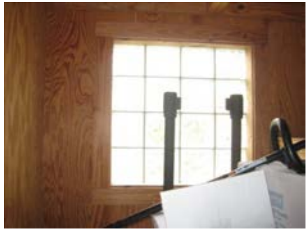
FIGURE 429. Glass block windows, one on each of the east and west sides of the room. Photograph by BVH, October 16, 2012.
