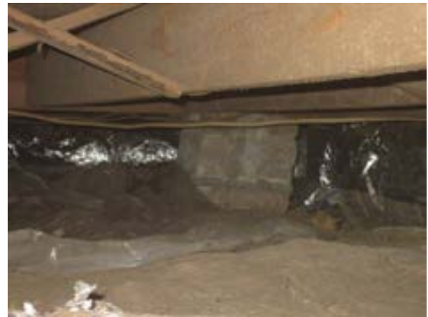
FIGURE 181. Detached 1-foot-square piers were observed along the north-south centerline of the house, view looking west. Photograph by WJE, October 16, 2012.
