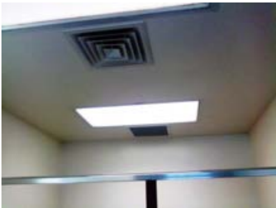
FIGURE 454. Ceiling supply and return air diffuser and grille at women's restroom 102 of the comfort station (men's restroom 103 is similar). Photograph by Alvine, May 15, 2013.
