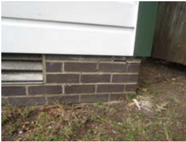
FIGURE 196. Typical cracking and deflections up to 3/8 inch observed at the masonry foundation, view looking north. Photograph by WJE, October 16, 2012.
