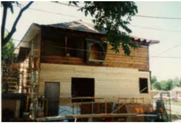
FIGURE 40. Image of the north side wall of the Cassidy House during construction, July 7, 1995. This view shows scaffolding in place, new wood siding in the process of installation, and the opening for the whole house fan. Note that the window sash and door have been removed. Photo by Terry Huitt from the Clinton Home Restoration Scrapbook prepared by Cromwell Architects, 1995-1996, page 17.
