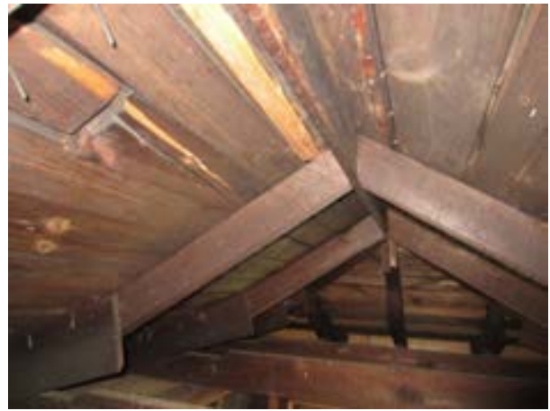
FIGURE 192. View of roof framing at the hipped dormer on the west side of the roof, view looking west. Photograph by WJE, October 16, 2012.
