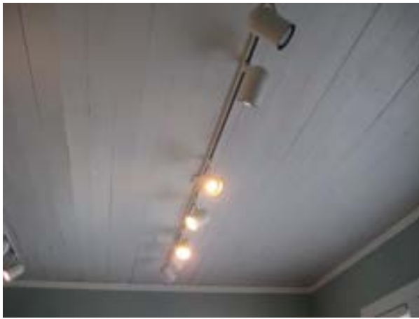
FIGURE 299. Track lighting in the exhibit space, looking west. Photograph by BVH, October 16, 2012.
