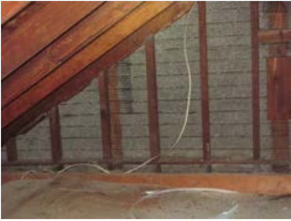
FIGURE 377. Partial view of a typical gable end wall framed with 2 by 4 studs to support stucco cladding, view looking west. Photograph by WJE, October 16, 2012.
