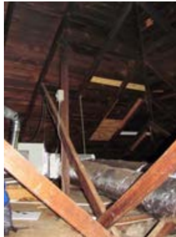
FIGURE 189. Common rafter with brace members that cross at midspan in the north-south direction. Hip jack rafters frame into a hip rafter beyond, view looking southwest. Photograph by WJE, October 17, 2012.
