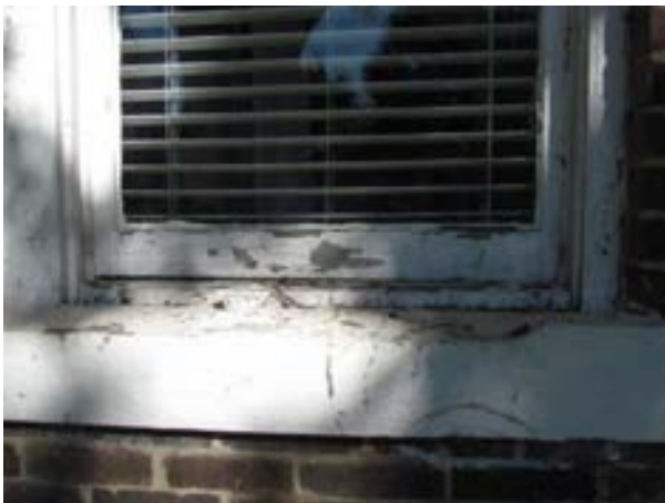
FIGURE 276. A view of a typical window showing paint and glazing putty failure. Photograph by WJE, October 15, 2012.
