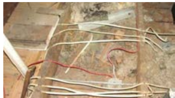
FIGURE 237. Cassidy House showing incorrectly supported nonmetallic sheathed cable in attic. Photograph by Alvine, May 15, 2013.
