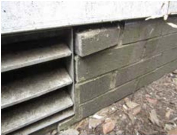
FIGURE 197. Loose brick observed at the east side of the masonry foundation, view looking west. Photograph by WJE, October 16, 2012.
