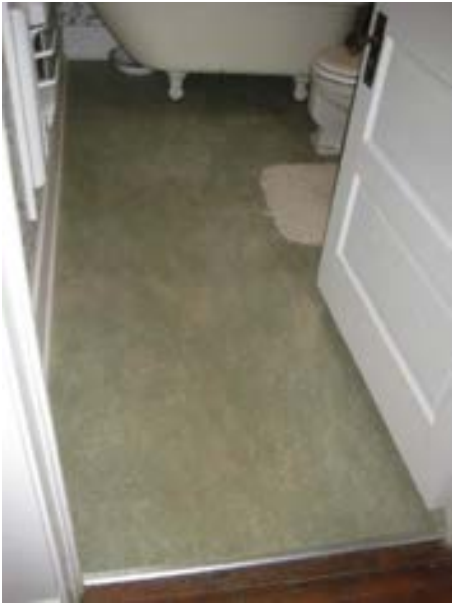
FIGURE 152. Flooring in the bathroom with a metal transition strip at the door to the hall, looking east. Photograph by BVH, October 16, 2012.
