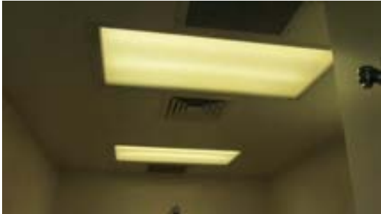
FIGURE 475. Ceiling-mounted lighting fixtures in the toilet room. Photograph by Alvine, May 15, 2013.
