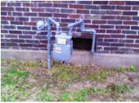
FIGURE 394. Gas meter and service entrance location at west side of the visitor center. Photograph by Alvine, May 15, 2013.
