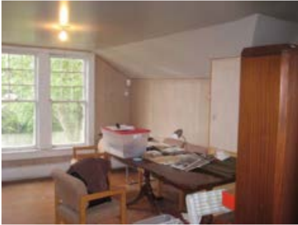
FIGURE 342. White painted plaster ceiling with bare bulb light fixture, looking south. Photograph by BVH, October 16, 2012.
