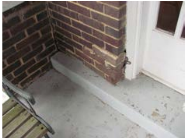
FIGURE 368. Location of loose bricks at north elevation where an inspection opening was made to view the condition behind the brick veneer, view looking southeast. Photograph by WJE, October 16, 2012.
