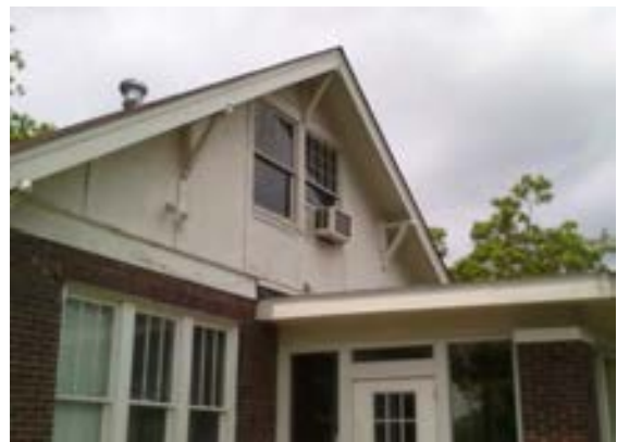
FIGURE 389. Window air conditioner at east storage 202 of the second floor of the visitor center. Photograph by Alvine, May 15, 2013.
