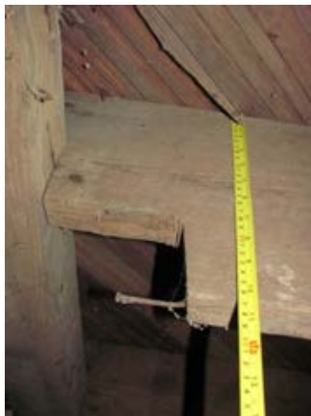
FIGURE 383. Two joists were noted to have a second notch at the tension face, view looking west. Photograph by WJE, October 17, 2012.
