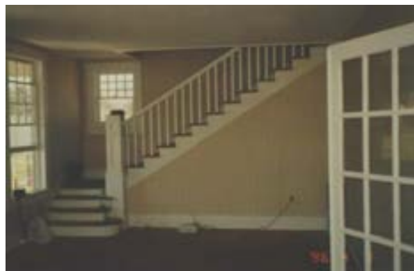
FIGURE 58. Interior view of living room looking north showing the room near completion, April 1, 1996. The staircase has been repainted, and new wallpaper has been installed. Photo by Terry Huitt from the Clinton Home Restoration Scrapbook prepared by Cromwell Architects, 1997, page 31.
