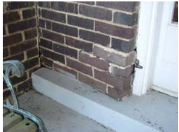
FIGURE 273. A view of displaced brick adjacent to the door on the north elevation. Photograph by WJE, October 15, 2012.
