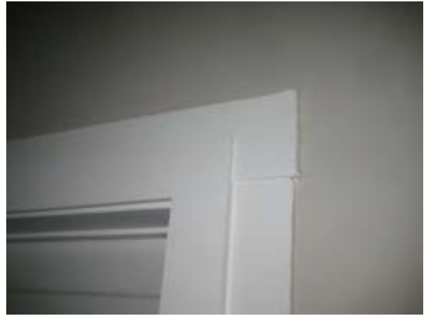
FIGURE 314. New door jamb and trim inserted into original south wall door opening. Photograph by BVH, October 16, 2012.
