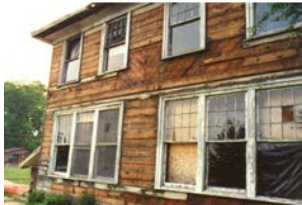
FIGURE 38. Photo showing the south side exterior wall of the Cassidy house during renovation, circa June 1995. The non-original cement asbestos siding has been removed, exposing remnants of the original wood siding, as well as portions of the underlying diagonal wood sheathing. The original window sashes were still in place. Photo by Terry Huitt from the Clinton Home Restoration Scrapbook prepared by Cromwell Architects, 1997, page 16.
