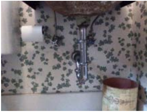
FIGURE 230. Waste and water supply piping serving lavatory at Cassidy House second floor bathroom 203. Photograph by Alvine, May 15, 2013.
