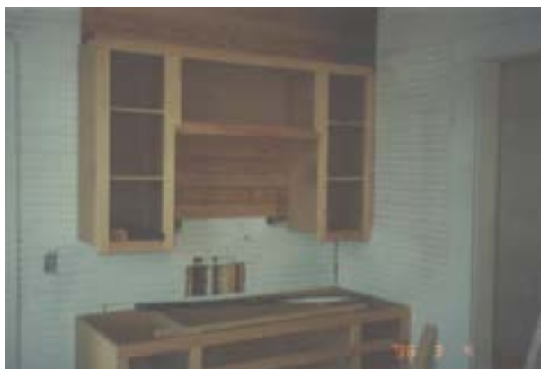
FIGURE 55. Interior of the kitchen, March 4, 1996. New built-in casework is in the process of being built. Surviving original beadboard wall cladding has been cut to allow plumbing to be run in the east wall. Photo by Terry Huitt from the Clinton Home Restoration Scrapbook prepared by Cromwell Architects, 1997, page 28.
