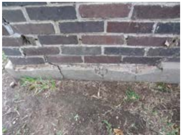
FIGURE 382. Typical cracking and displacement seen at foundation parge coat. Note, bricks beneath parge are also cracked, view looking east. Photograph by WJE, October 17, 2012.
