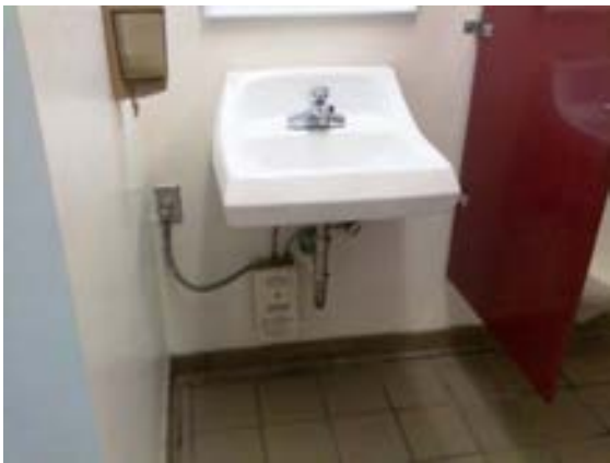
FIGURE 458. Wall-mounted lavatory at men's restroom 103. Photograph by Alvine, May 15, 2013.
