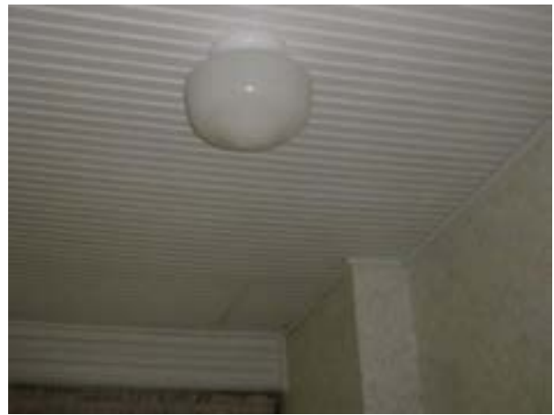
FIGURE 114. Hallway ceiling and light fixture. Photograph by BVH, October 16, 2012.
