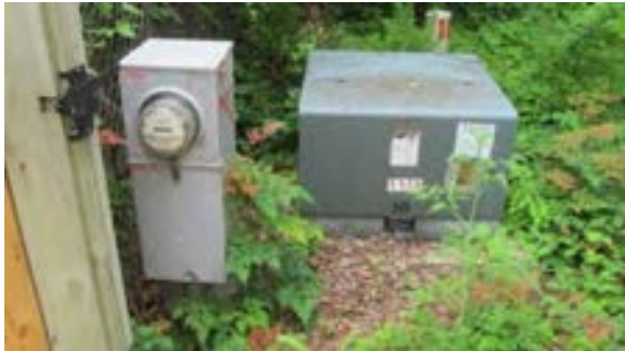
FIGURE 397. Power company pad-mounted transformer and the visitor center meter pedestal. Photograph by Alvine, May 15, 2013.
