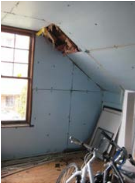
FIGURE 349. Walls of rigid insulation, with missing sections and rough seams, facing east. Photograph by BVH, October 16, 2012.
