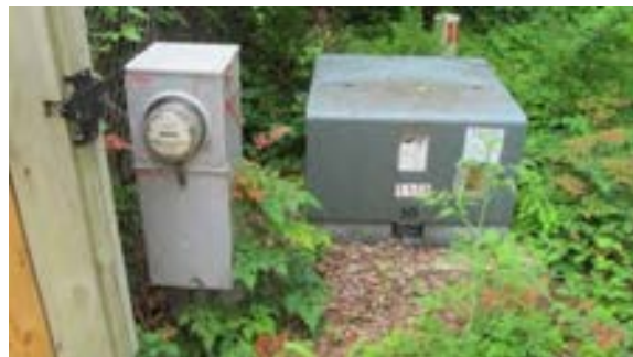
FIGURE 234. Power company pad-mount transformer and visitor center meter pedestal located in the former alley behind a wood fence, 25 feet south of comfort station. Photograph by Alvine, May 15, 2013.
