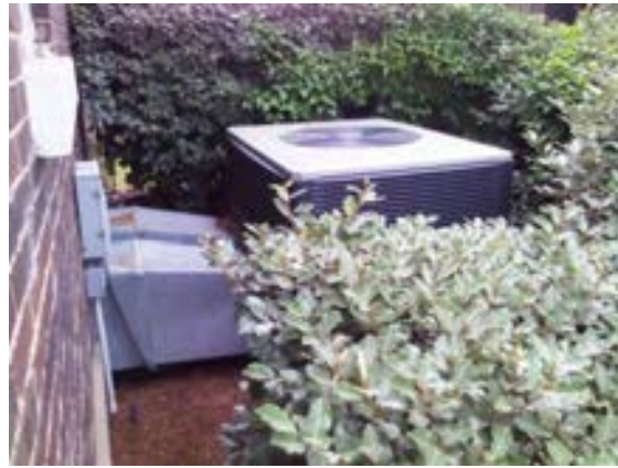
FIGURE 392. Grade-mounted packaged heating and cooling unit serving the visitor center. Photograph by Alvine, May 15, 2013.
