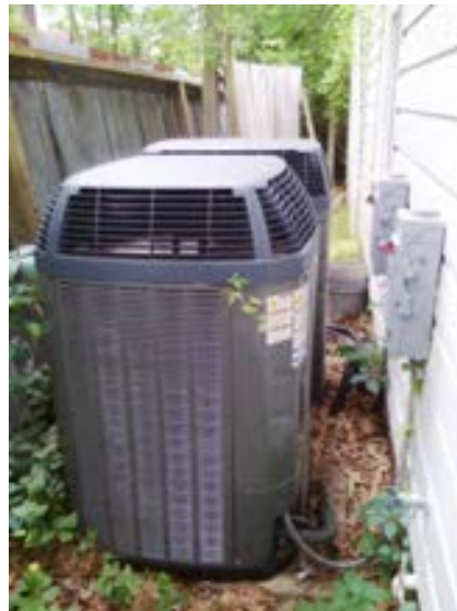
FIGURE 223. Cassidy House air-cooled heat pumps located on grade between house and adjacent property fence. Photograph by Alvine, May 15, 2013.
