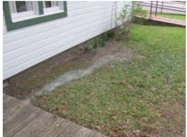
FIGURE 82. Erosion is present at locations around the house due to the lack of gutters and downspouts. Photograph by WJE, October 16, 2012.
