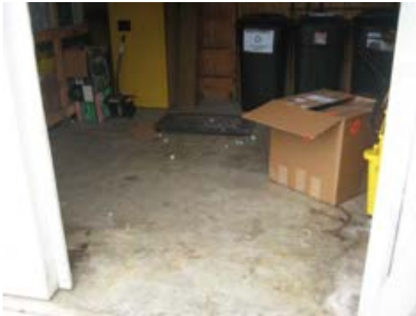
FIGURE 424. Concrete slab floor of the maintenance storage room, looking south. Photograph by BVH, October 16, 2012.
