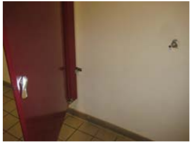
FIGURE 433. Damage to the gypsum board of the south wall due to the water closet door hardware puncturing the wall. Photograph by BVH, October 16, 2012.
