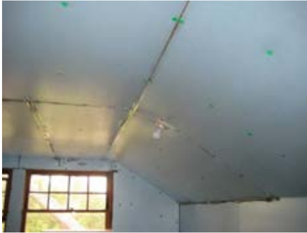
FIGURE 359. Ceiling with rigid insulation and bare bulb light fixtures, facing west. Photograph by BVH, October 16, 2012.
