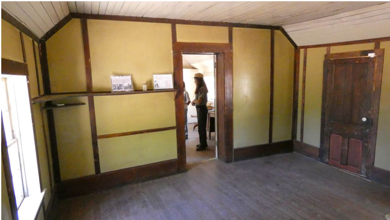
Figure 7. (a) Top, view of Room 3 interior by Paul Beaubien, August 1935, looking north. WACA 4330. (b) Bottom, the northeastern corner of Room 3, 2017, with the built-in shelves visible in the image above. (Photo credit: David E. Purcell).
