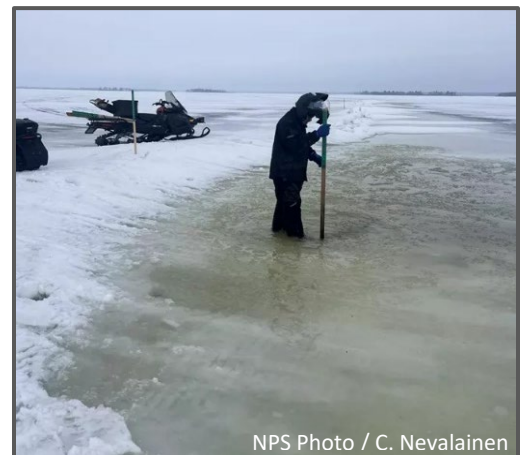
NPS Photo / C. Nevalainen Maintenance worker Jason Christenson inspects a pressure ridge on Kabetogama Lake that resulted in over one foot of standing water on top of the frozen lake surface along the green snowmobile trail.
