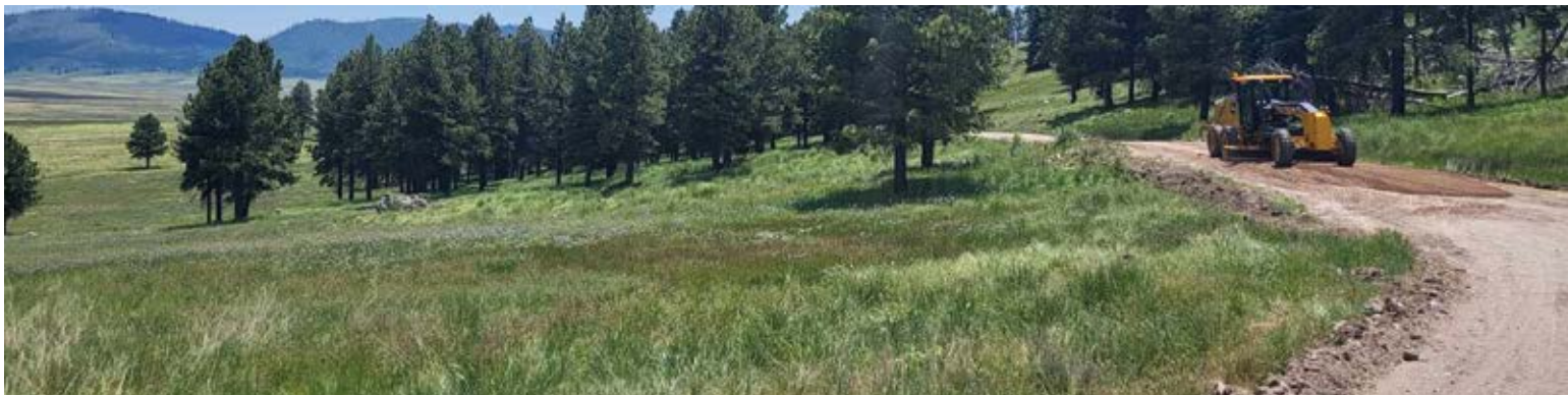
Park road grader working a section of the backcountry route near Cerro Piñon | NPS/L. Ray
