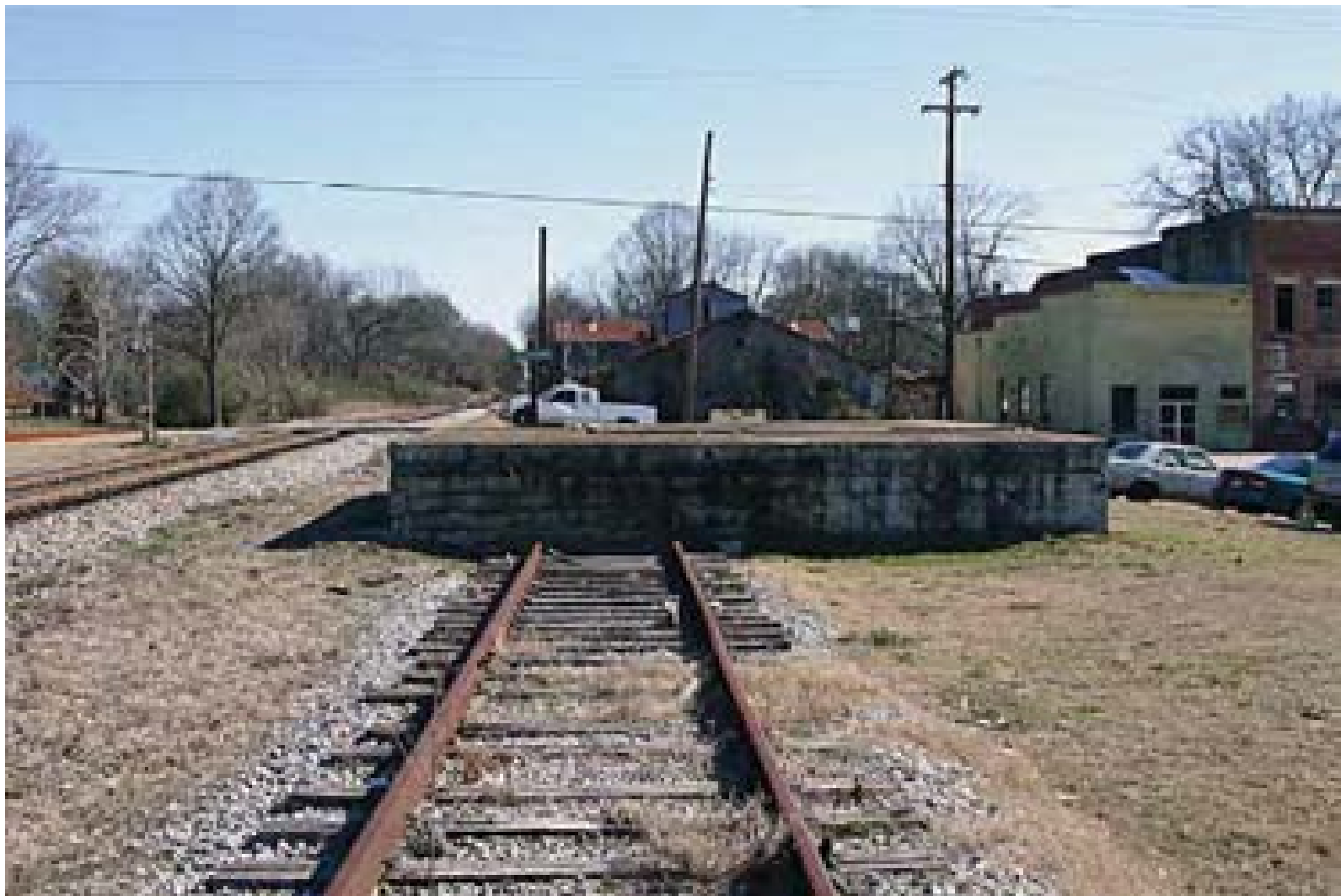
Figure 3.54 Leighton, Alabama Railroad Depot. The foundation is not the original depot foundation but this is probably the original location of the depot. Photo by Marty King.
