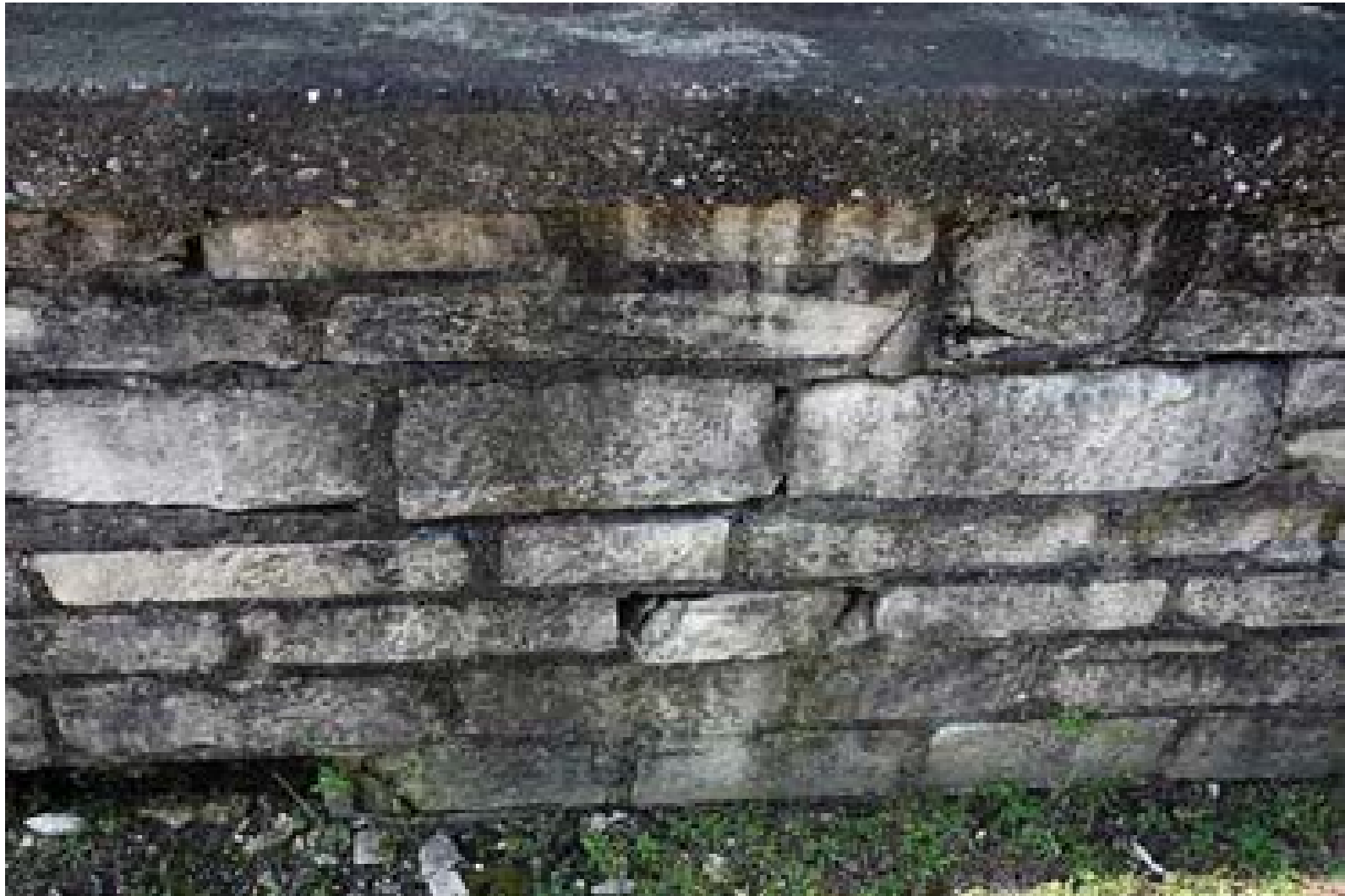
Figure 3.48 Close up of the Town Creek Railroad Depot foundation. Photo by Marty King.
