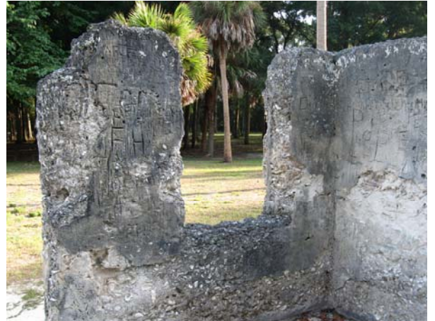
Evidence of vandalism in a slave cabin
