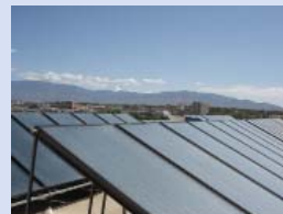
The solar panels are set back and installed at a low angle to the roof top so as not to be seen from the street.
