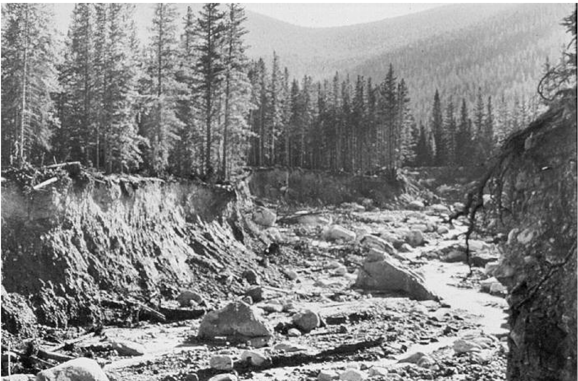
FIGURE 2. 1982 LAWN LAKE DAM FAILURE; A PRIVATE DAM WITHIN ROCKY MOUNTAIN NATIONAL PARK, COLORADO. EROSIONAL DAMAGE FROM THE FAILURE OF THE 26-FOOT-HIGH LAWN LAKE DAM. THE EROSION SCAR AND THE ALLUVIAL FAN DOWNSTREAM ARE STILL VISIBLE TODAY.
