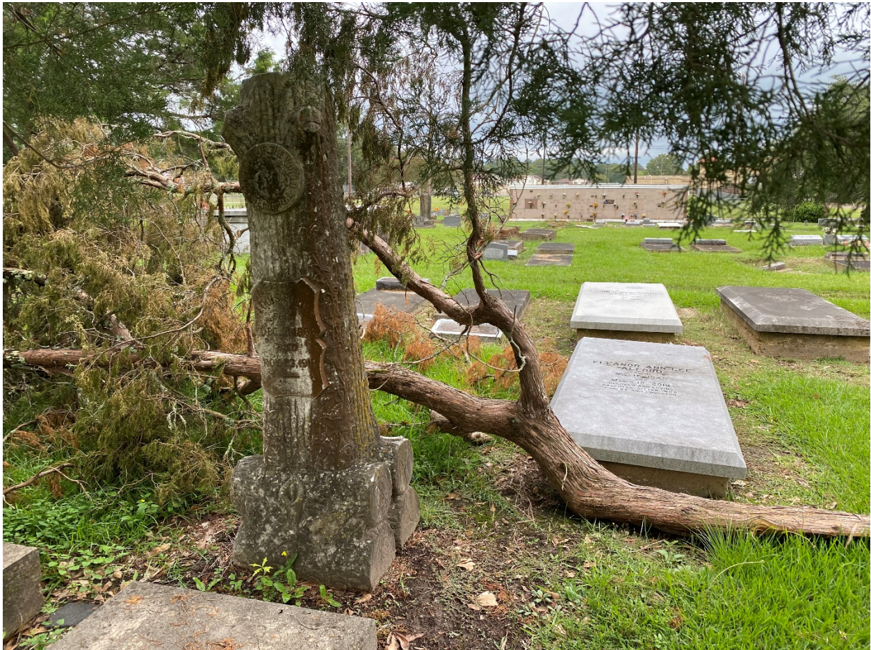
Dead wood should be pruned yearly to avoid potentially falling and damaging grave markers. Catholic Cemetery, Natchitoches, Louisiana
