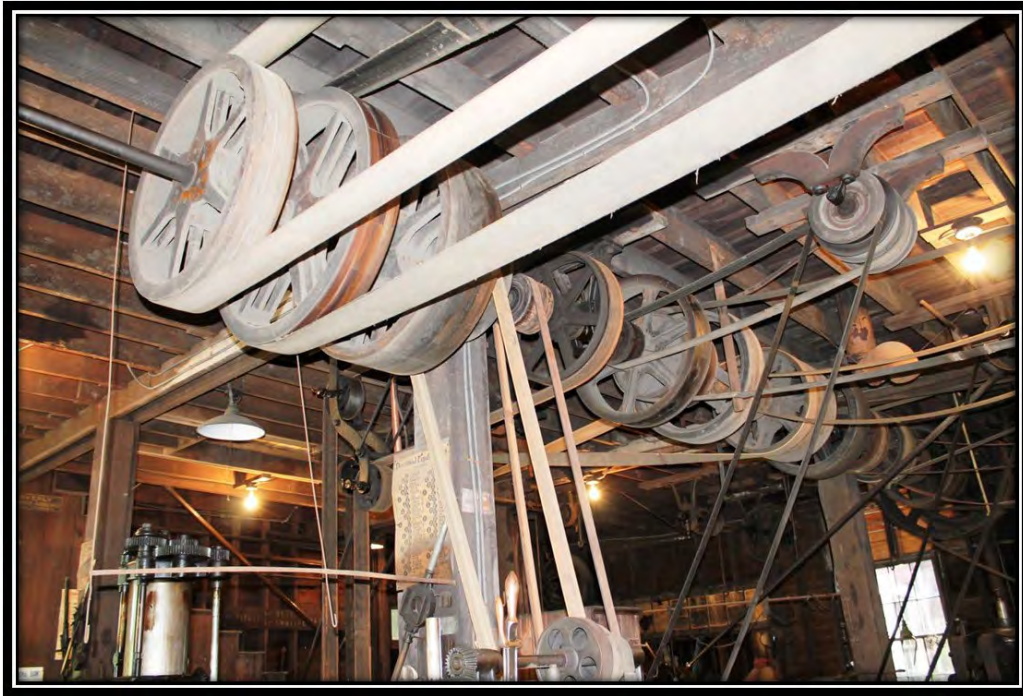
Photograph 12. PA_Greene County_W.A. Young & Sons Foundry and Machine Shop_0012. Horizontal line shaft in the Front Shop, facing southeast.
