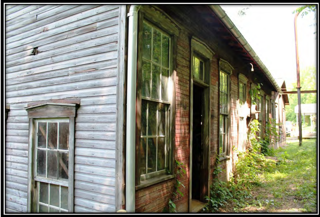
Photograph 9. PA_Greene County_W.A. Young & Sons Foundry and Machine Shop_0009. Rear (south) elevation of the Back Shop, facing east.
