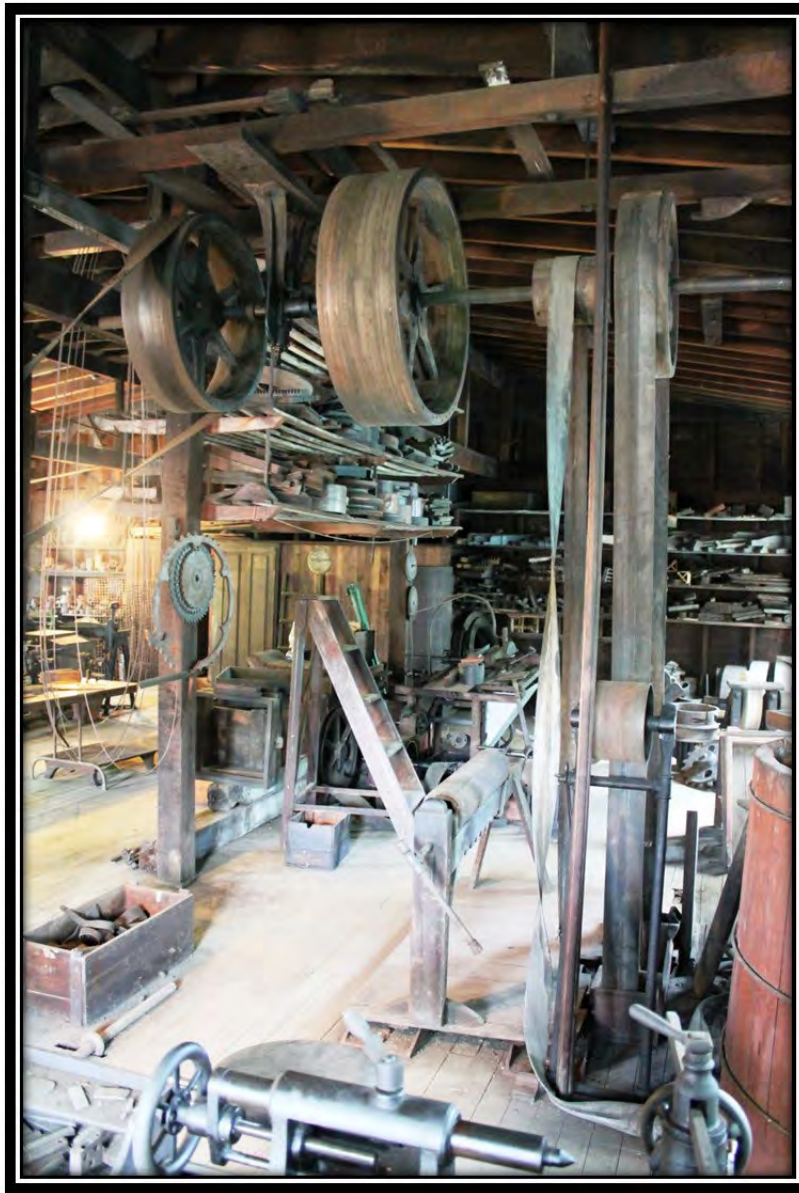
Photograph 27. PA_Greene County_W.A. Young & Sons Foundry and Machine Shop_0027. Belt from the main line shaft and Pattern-Shop line shaft, facing east. A portion of the water tank for the gravity-fed cooling system is also visible on the right.
