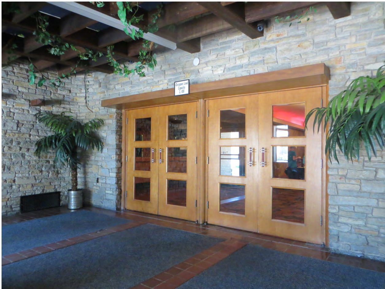
Photograph 9: Interior: Vestibule, looking northwest. The entrance vestibule retains original face-stone walls, timber beamed ceiling, glazed terra cotta tile floor, and paired, wood doors with Bakelite handles. A comparison with the 1948 historic photograph reveals no discernible alteration of the vestibule. (McDowell, 2018)
