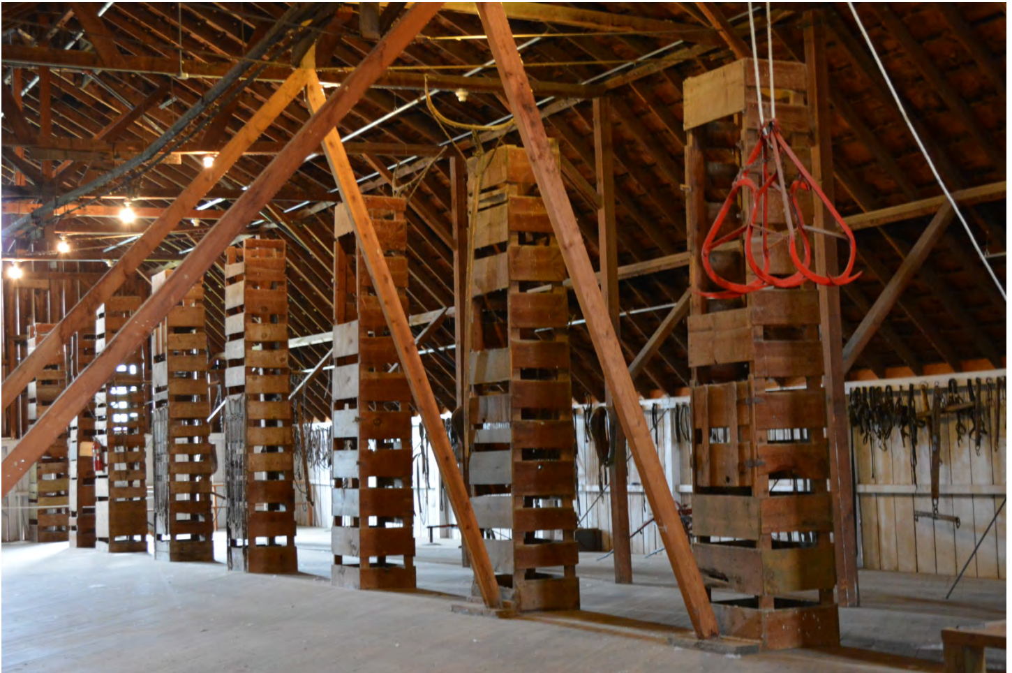
SCOUT'S REST RANCH HEADQUARTERS, North Platte, Nebraska Horse Barn second floor interior, hay storage and chutes Photo by Hannah Braun, June 2015
