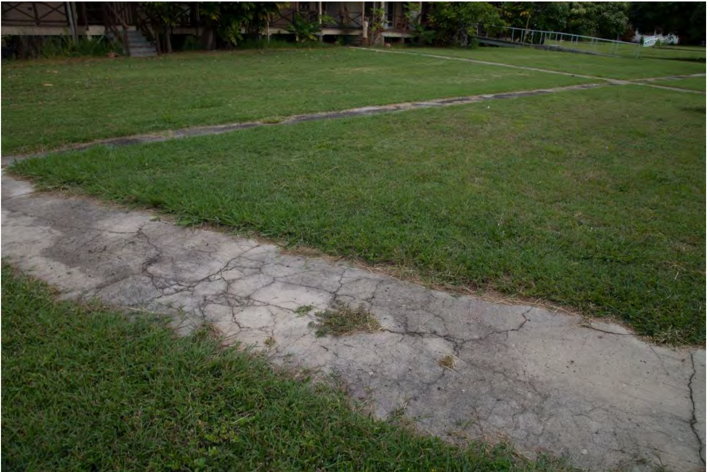
Photo 33: Section of the contributing Bay View Sidewalks (860) which link the buildings of the Bay View Home, camera facing southeast.
