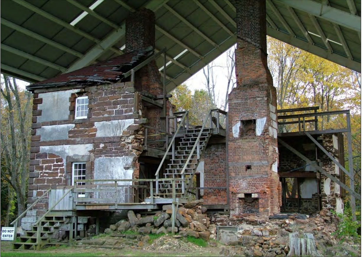
FIGURE 7. MENOKIN – A PLANTATION ONCE OWNED BY FRANCIS LIGHTFOOT LEE IN RICHMOND COUNTY, IS CURRENTLY THE SUBJECT OF AN INNOVATIVE RESTORATION AND STABILIZATION PROGRAM
