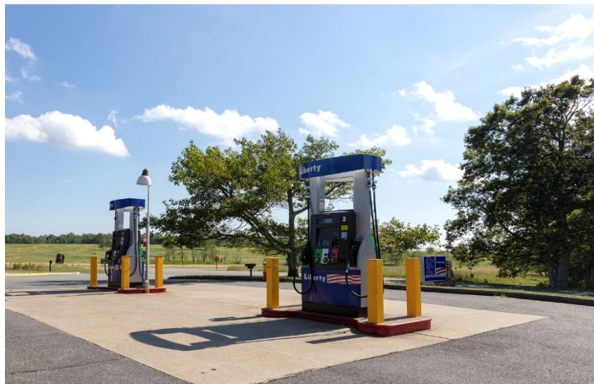
Pictured: Gas Pumps at Big Meadows Wayside
