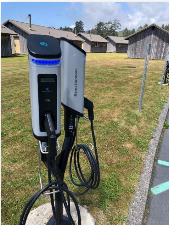
EV Charging Station, National Park Service
