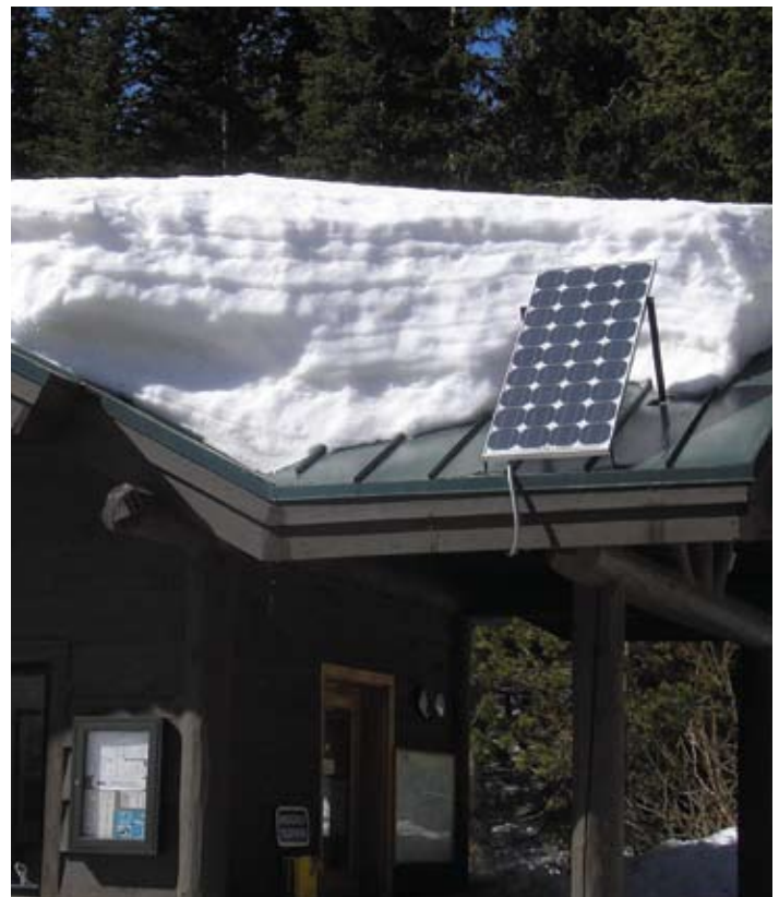
Solar Array on a Rocky Mountain Park building
