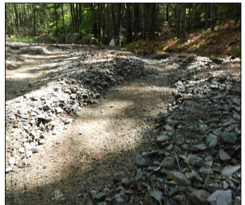
Exceptional flooding removed three layers of surface from multiple sections of carriage roads in Acadia National Park. NPS Photo.
