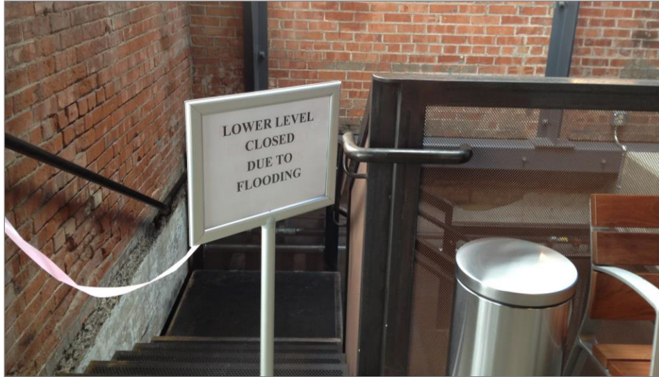
Photo 2. Basement flooding in the visitor center at Rosie the Riveter WWII Home Front National Historical Park. This photograph was taken on December 5, 2012 —12 years after the establishment of the park. Photo credit: Maria Caffrey.
