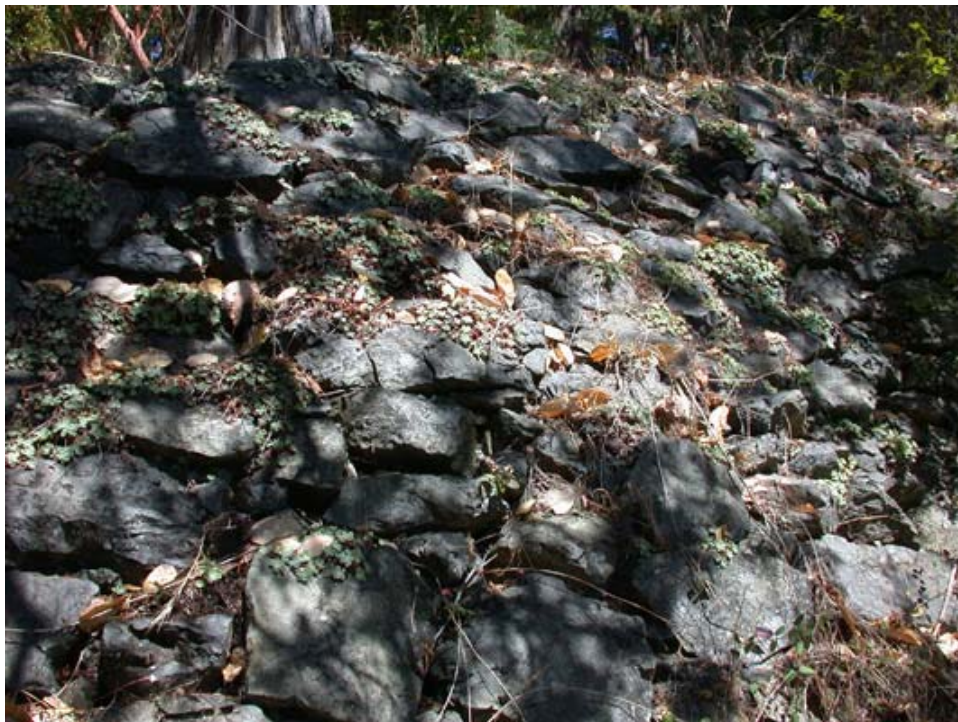
Contemporary view of a retaining wall on Officers' Hill. The lichens and herbaceous vegetation growing in the wall do not pose a significant threat to the wall's integrity. (CCSO, 2003)
