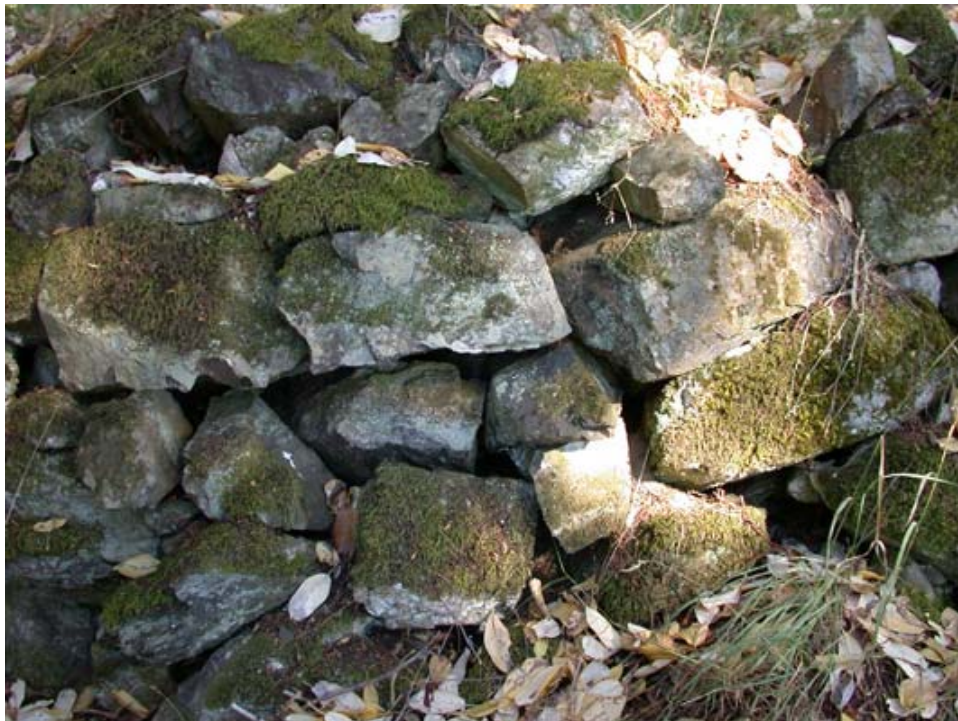
Contemporary photo showing a detail of a retaining wall. This shows a construction method of dry and mortared stone typical of the circulation and retaining walls at English Camp. (CCSO, 2003)
