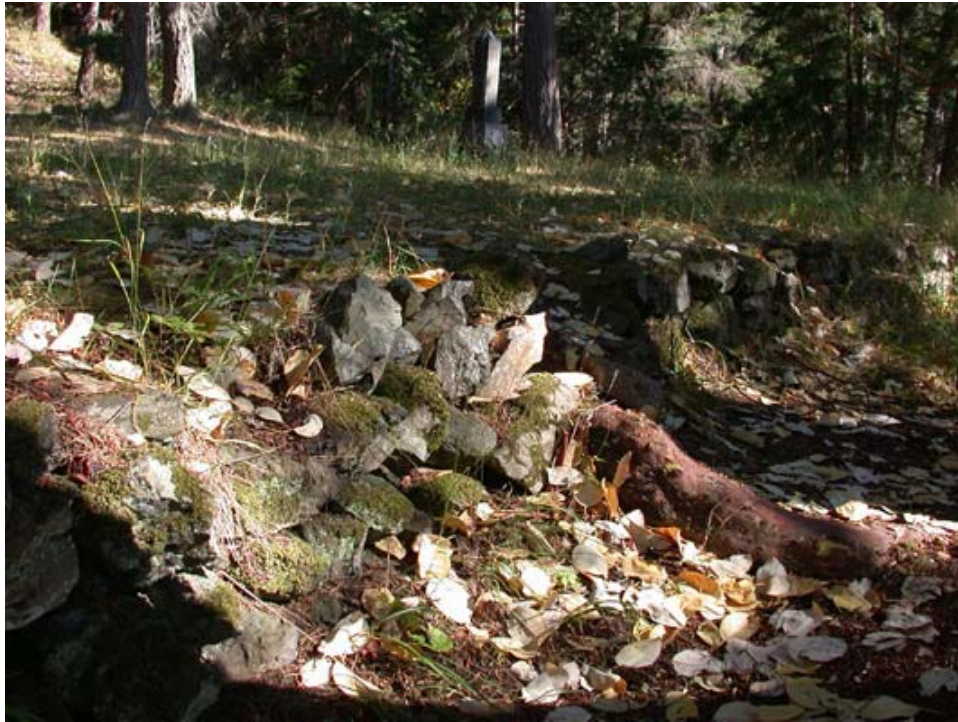
Contemporary view of a retaining wall on the top terrace of Officers' Hill. This wall has been damaged by visitor traffic over the wall. (CCSO, 2003)
