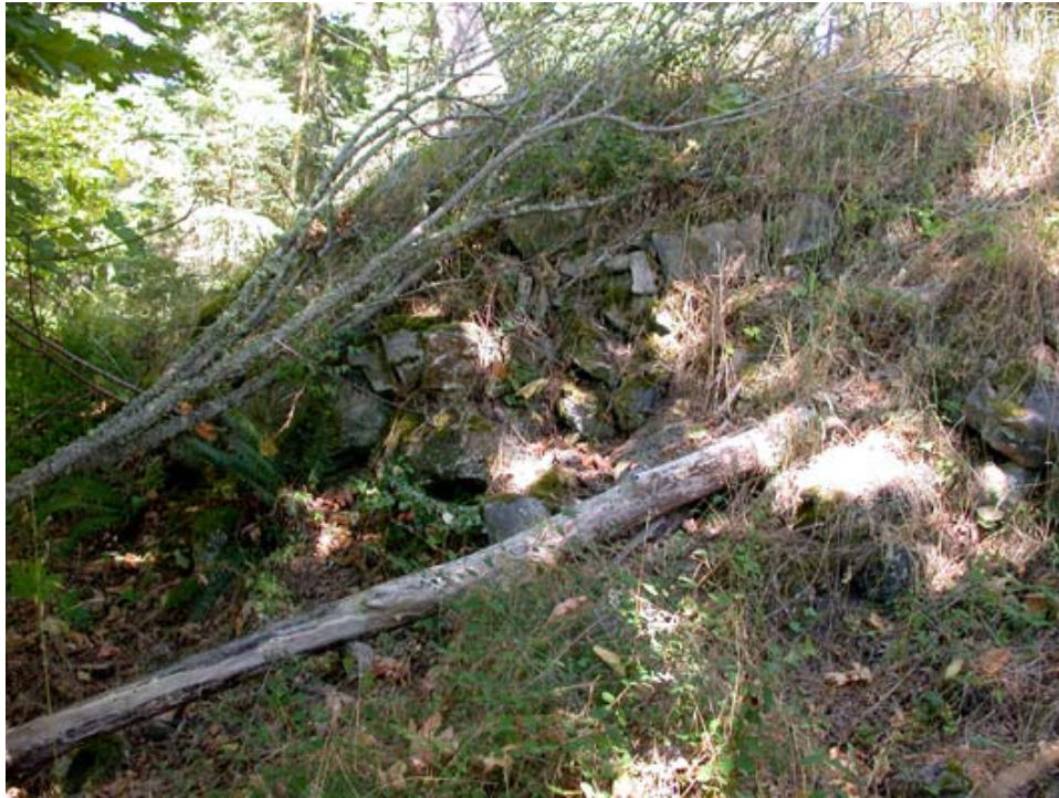
Contemporary view showing damage to a retaining wall by vegetation and erosion. (CCSO, 2003)
