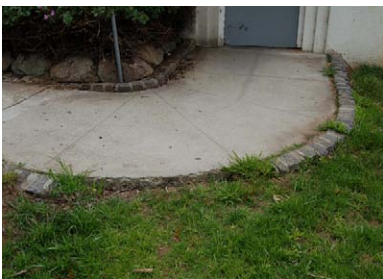
Figure 94. Missing block curbing at the West Convenience Station should be repaired using in-kind materials. (NPS, 2007)
