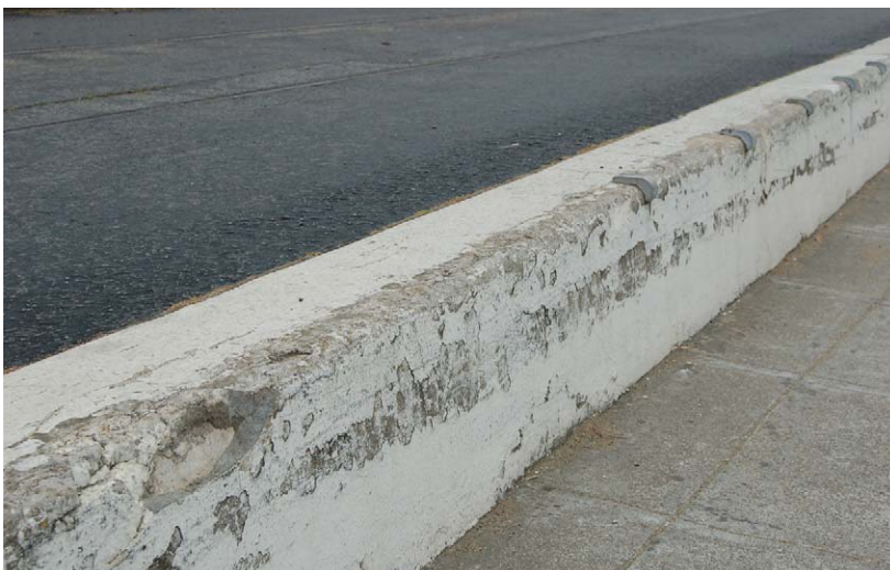
Figure 96. Flaking and loss of material along the concrete wall occurs as deterrent bolts fail and water penetrates the under layers of the concrete. Repair may require patching, reapplication of a skim-coat, or some combination. View of the east end of the wall, looking west. (NPS, 2007)
