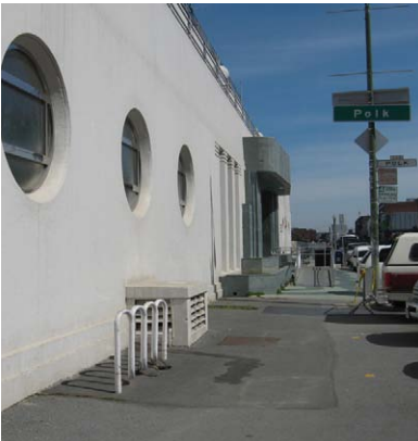
Figure 89. On the west side of the front entrance to the Bathhouse, a bicycle rack, accessibility ramp, and various small-scale features and utilities create a cluttered appearance. Note asphalt paving where planting bed was originally located. (NPS, 2010)
