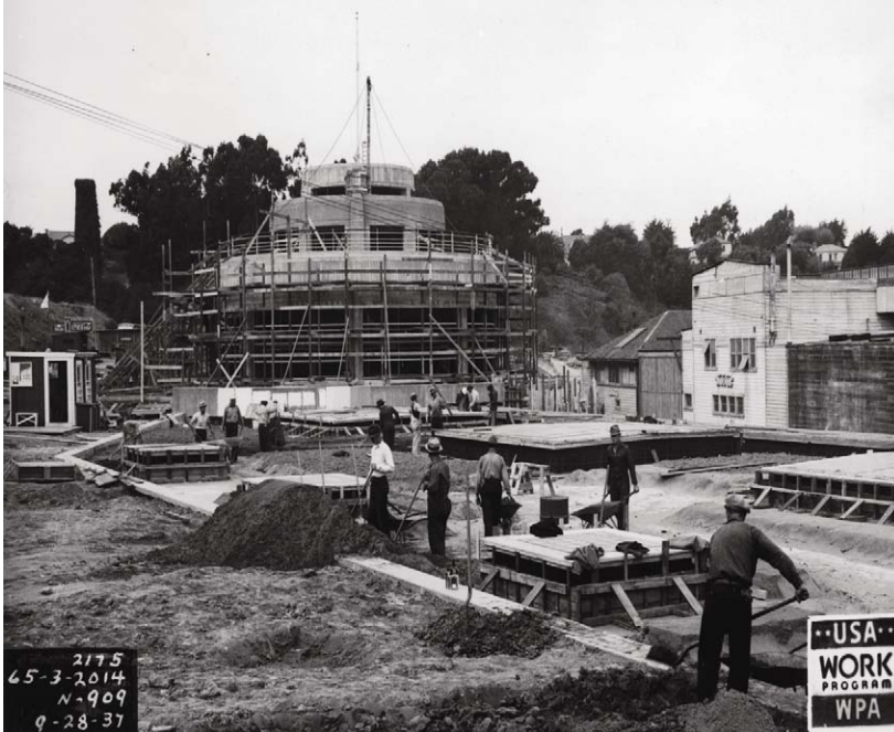
Figure 20. Site work and rough grading east of the Bathhouse moved quickly through the fall of 1937. View looking west. ( San Francisco Maritime NHP, Historic Documents, Photograph Collection, P88-035.00087 )
