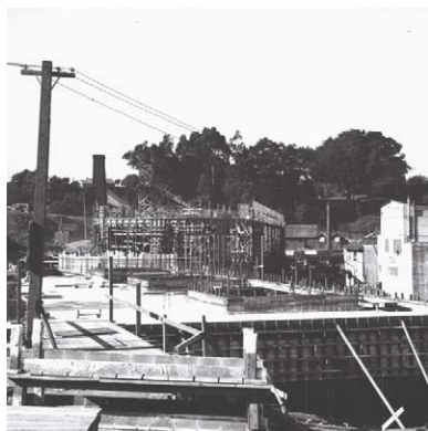
Figure 18. By February 1937, crews were framing and completing concrete work for the upper floors of the Bathhouse. ( San Francisco Maritime NHP, Historic Documents, Photograph Collection, P88-035.00074 )
