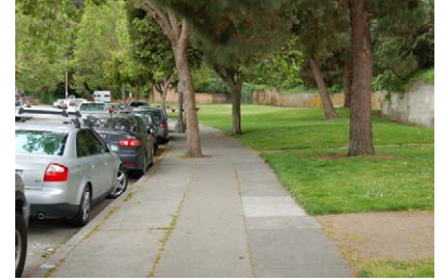
Figure 108. Displaced, cracked, and patched sidewalk along Van Ness Avenue next to Pocket Park. At a certain point, rather than patching, a holistic approach to rehabilitation of the sidewalk will assure a more uniform character. View looking south. (NPS, 2008)
