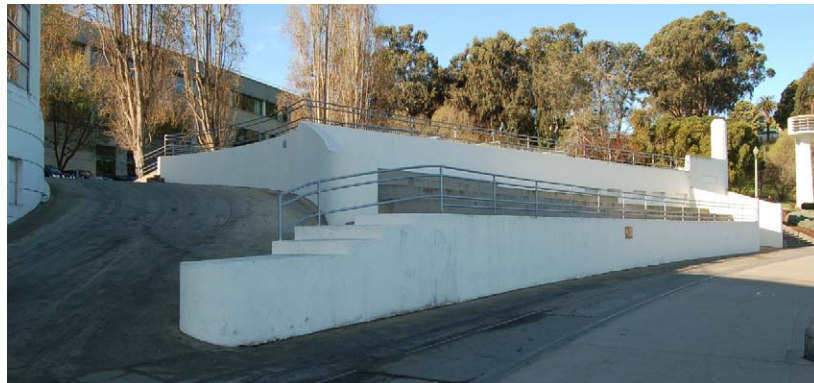
Figure 57. West Bleachers prior to rehabilitation. Note the ramp between the bleachers and the Bathhouse. View looking southwest. (NPS, 2007)
