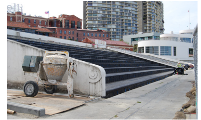
Figure 90. View of the East Bleachers showing new waterproofing material applied during rehabilitation. Note mildew on the concrete wall. Cleaning and repainting this portion of the structure is important to the character of the structure, and should be integrated into overall maintenance. (NPS, 2009)
