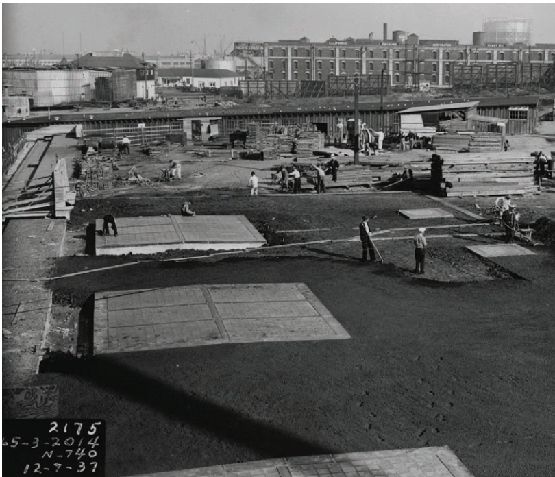
Figure 21. By December, 1937, finish grading around the skylights provided the level area needed for the establishment of turf grass and planting beds east of the Bathhouse. View looking east. ( San Francisco Maritime NHP, Historic Documents, Photograph Collection, P88-035.00102 )
