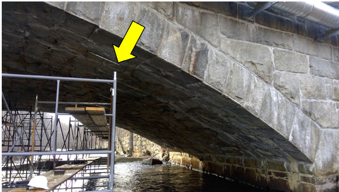
Figure 1.16: View of a stone arch bridge instrumented with a vibrating wire strain gage (indicated with an arrow) to measure strains during a load test. (Author 2018)
