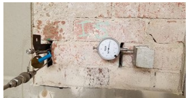
Figure 1.14: In situ shear index testing at a clay brick masonry wall in accordance with ASTM C1531. (Author 2018)
