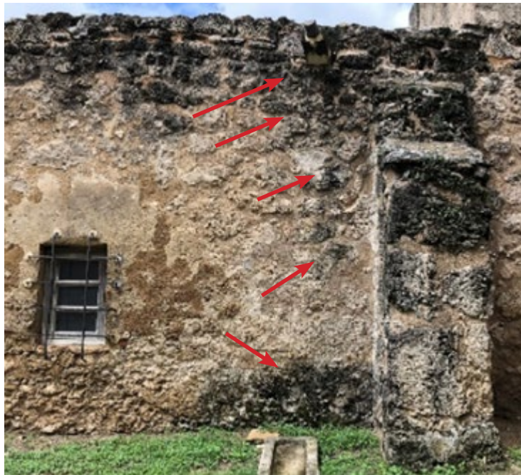
Figure 3.3: Evidence of roof drainage discharging close to the building and/or directly onto the masonry walls.
