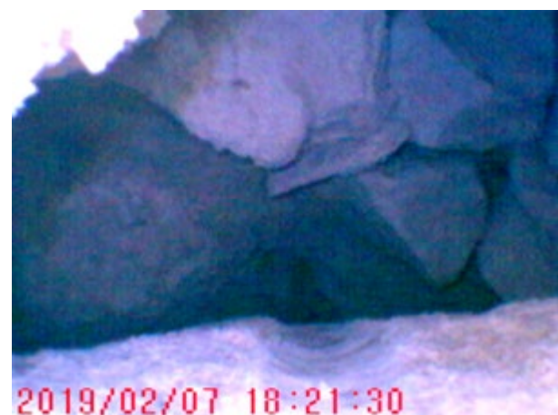
Figures 1.1a and b: Examples of borescope imagery from a historic stone masonry wall showing void areas. (Author 2019)
