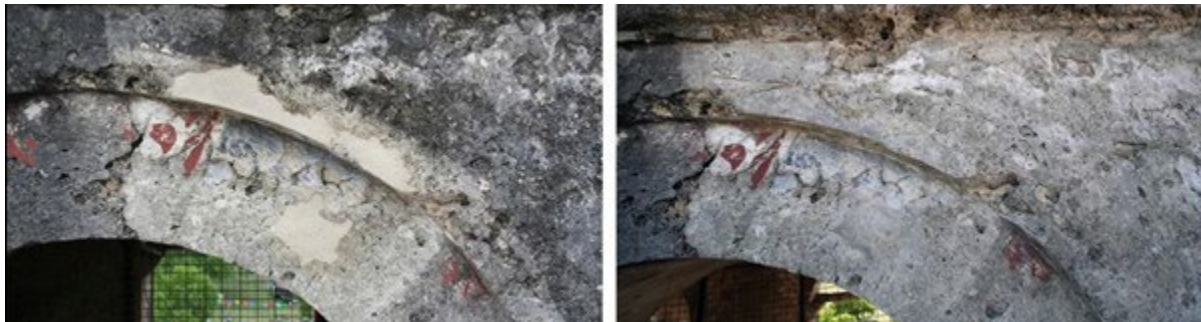
Figure 8.11: At left, loss compensation using a hydraulic lime-based repair mortar on the belfry arch, south tower, east elevation. The filled loss at the belfry window arch reestablishes the shape of that element; this fill is ready for toning. At right, the fill was toned while still wet to match the color of the surrounding plaster. As part of this pilot treatment, a portion of the historic plaster was cleaned; over a period of five years or so, cleaned surfaces were re-colonized by surface biota (Conservation Associates, 2013)
