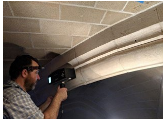
Figure 1.9: View of engineer holding UPE array against the surface of a stone rib at a church structure. (Author 2018)
