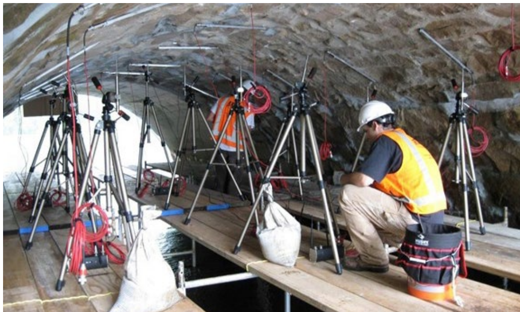
Figure 1.15: Structural monitoring system installation at stone arch bridge prior to load testing. (Author 2008)
