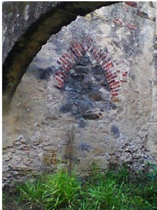
Figure 3.2: Rising damp, in which subgrade moisture rises via capillary action through the porous masonry walls. Rising damp results in deterioration, staining, biological growth, and efflorescence on the walls. Rising damp is especially likely to affect stone units installed with the bedding planes oriented vertically.
