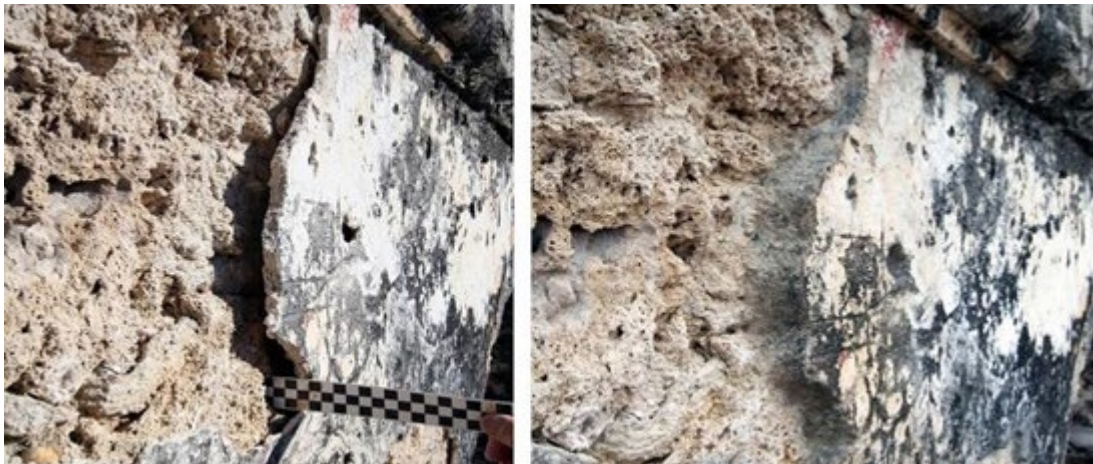
Figure 8.10: Before (left) and after emergency stabilization (reattachment by grouting and edging of the fragment) of the south tower belfry arch, west elevation. The plaster was buckling and detached, with a void over 25 centimeters deep. The fragment was secured in place by injection grouting; the applied edging mortar supports the edges of the fragment and was toned to blend with the patina of the existing plaster. In a later phase of treatment, a compensating plaster will be applied over the exposed masonry. (Conservation Associates, 2012)
