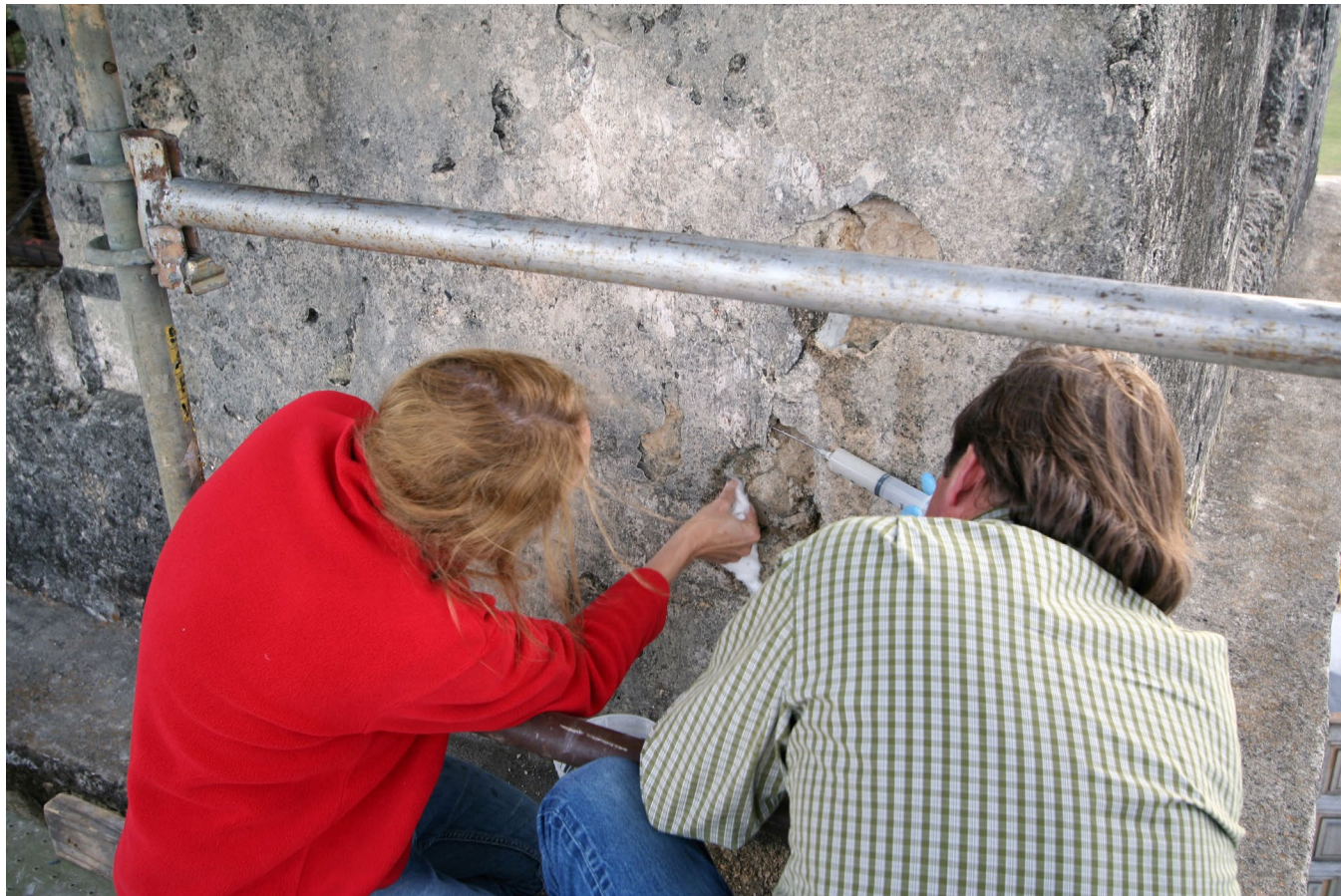
Figure 0.6: Angelyn Bass and Douglas Porter at Mission Concepción reattaching and stabilizing delaminated plaster by grout injection.
