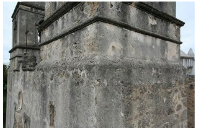
Figure 8.4: Weathering of the plaster on the south facade of the south tower at Mission Concepción church is severe on north-facing exposures, less so on the south. The south facade plaster on the south tower, seen here, is approximately 77% intact, including several surviving fragments on the chamfered tower pedestal, while there are large losses in the same zone on the west facade. Note the large losses in the frieze, many of them located below gaps in the moldings and other horizontal elements, resulting in water infiltration, detachment and loss of the plaster, and concentrations of biological growth along these paths.
