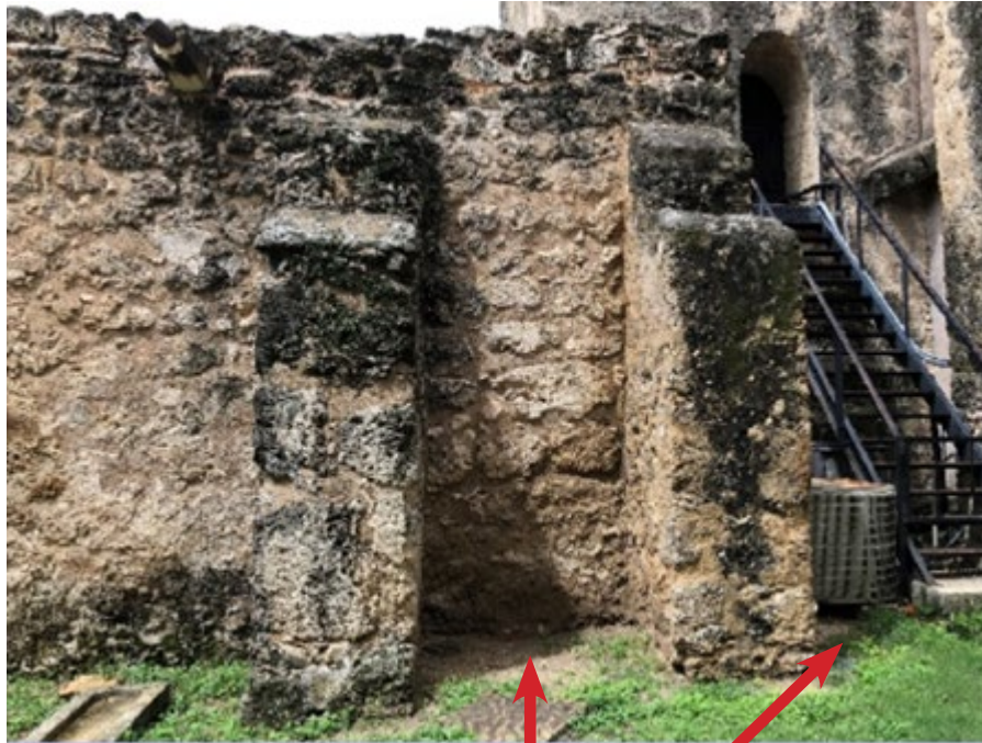
Figure 3.1: Poor site drainage, resulting in ponding water near the walls. At some sites, the slope of the ground directs water toward the historic structures, or changes in grade over time result in the present-day exterior ground level being above the level of the interior floor.
