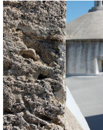
Figure 8.3: This loss at the southwest corner of the north tower reveals a plaster stratigraphy consisting of an extruded mortar that fills joints, a base-coat plaster that levels larger voids, covered with a thin finish coat forming a beautifully executed corner. On the bell towers, there are typically two distinct plaster layers; on the main block, there are two to three. (Conservation Associates, 2012)
