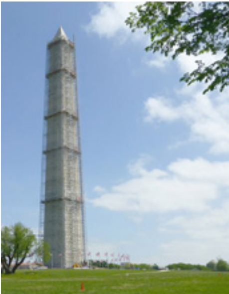
On the Cover: Damaged by an earthquake in 2011, the Washington Monument undergoes repairs funded through a public-private partnership. NPS photo.
