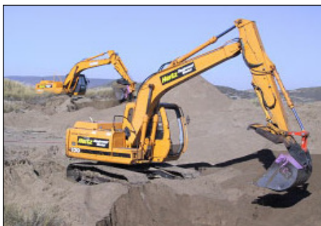
Contract and volunteer crews as well as heavy equipment are restoring dune ecosystems.
