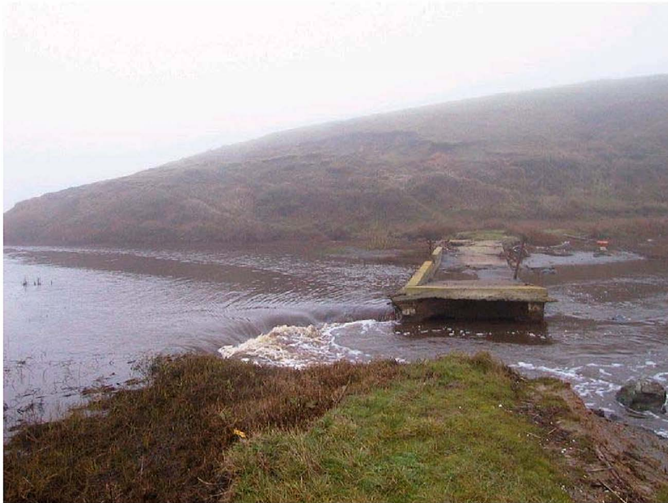
Figure 12. Photo of spillway failure as water continues to drain out of Horseshoe Pond. January 3, 2002.
