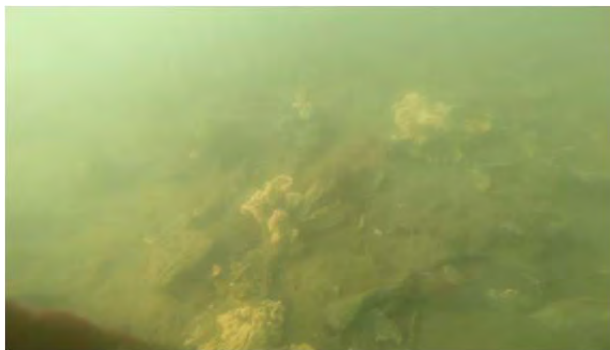
Upper end of moderate class of debris under rack 9C on 1/29/2015
