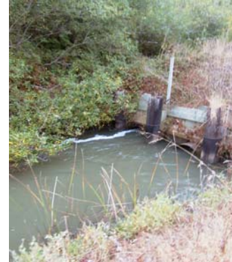
Leaky gate on Fish Hatchery Creek
