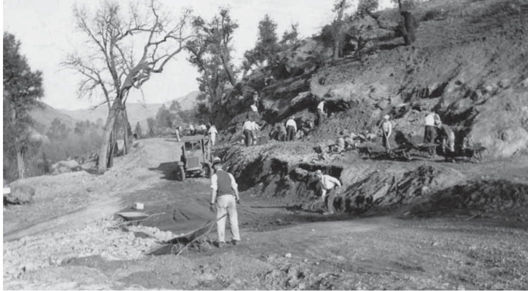
Figure 33. CWA laborers working on road cut at Chalone Wye (intersection at the bottom of Bear Gulch), 1934. [Landscape Architects' Reports, PINN Coll. 3658, Misc. Boxes, PNM.]
