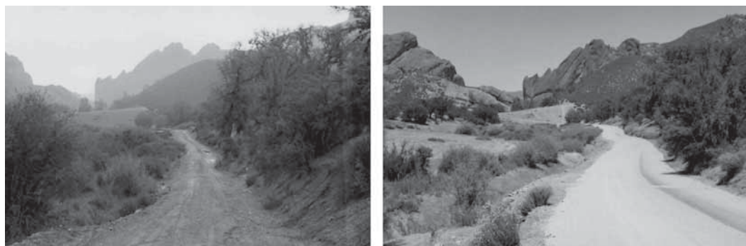
Figure 53. West entrance road approaching Chaparral Area in 1966, before construction (left) and after (right). [Mus. Coll. PINN 4372, PNM.]
