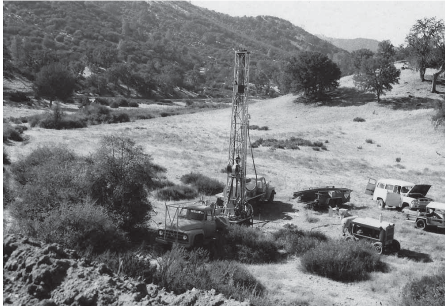
Figure 54. BZM Drilling Co. at Test Well No. 2 in the Chaparral Area in 1965. This well produced a strong artesian flow at a depth of one hundred feet. [Mus. Coll. PINN 4372.]
