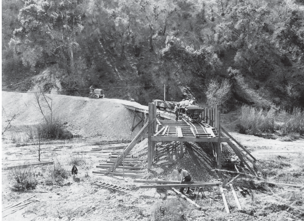
Figure 27. Construction of Bear Gulch entrance road in 1932. Waste rock from cut slopes being deposited in Chalone Creek to establish abutments for future bridge. [Mus. Coll. PINN 4372, PNM.]
