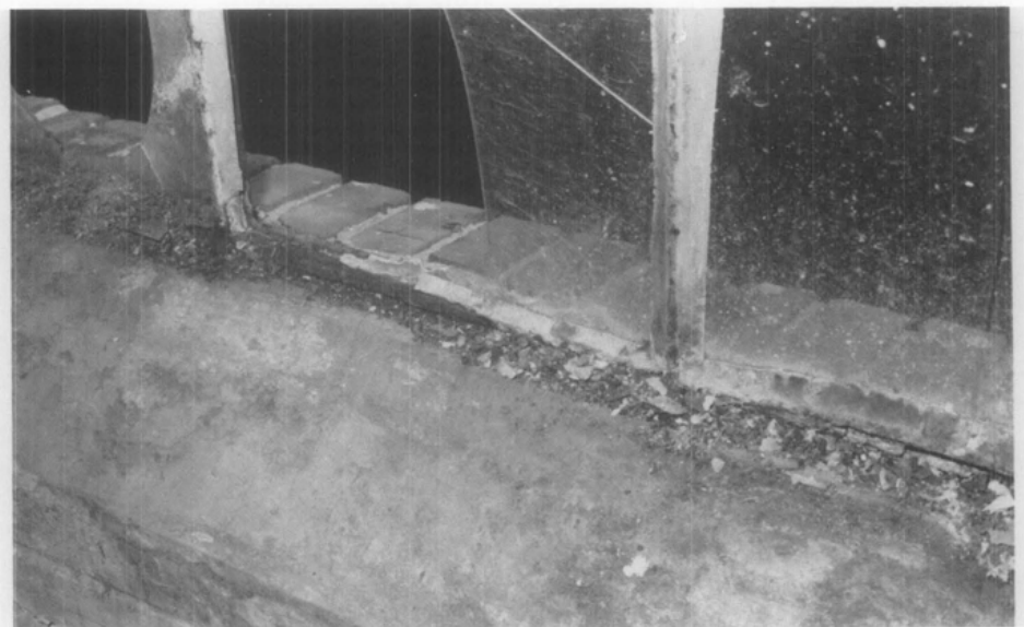
Figure 5. Sill corrosion typically found on 95% of the windows. Photo: Clío Group.
