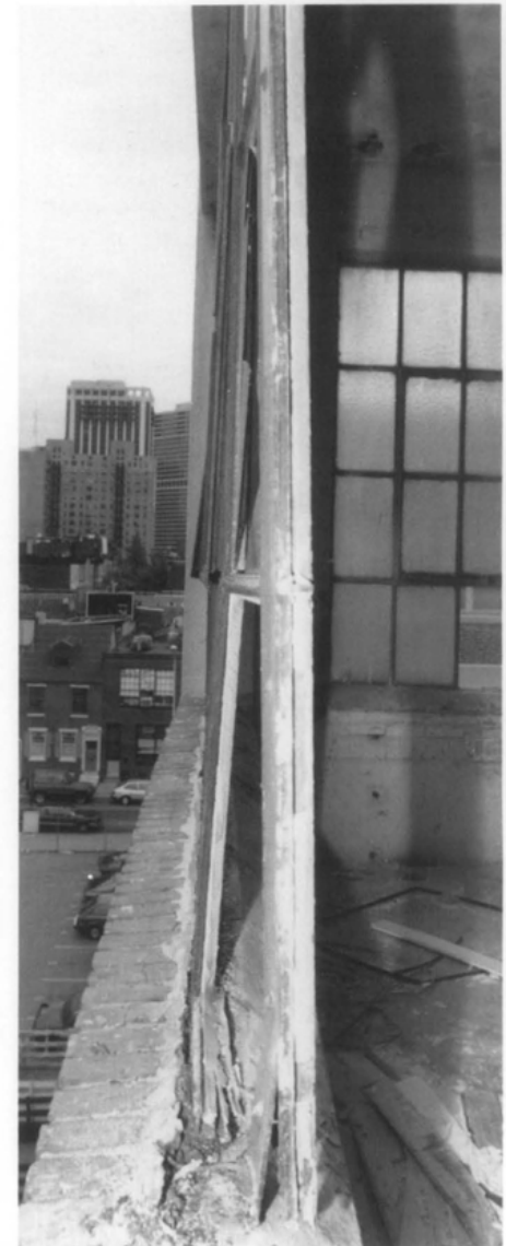
Figure 8. Bowed and corroded window during construction. Photo: Clío Group.
