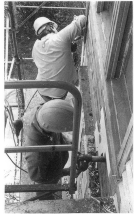
Figure 5. Using scaffolding, workers remove the paint with heat guns. Cracked or deteriorated siding was repaired or replaced. Photo: Alan O'Bright
