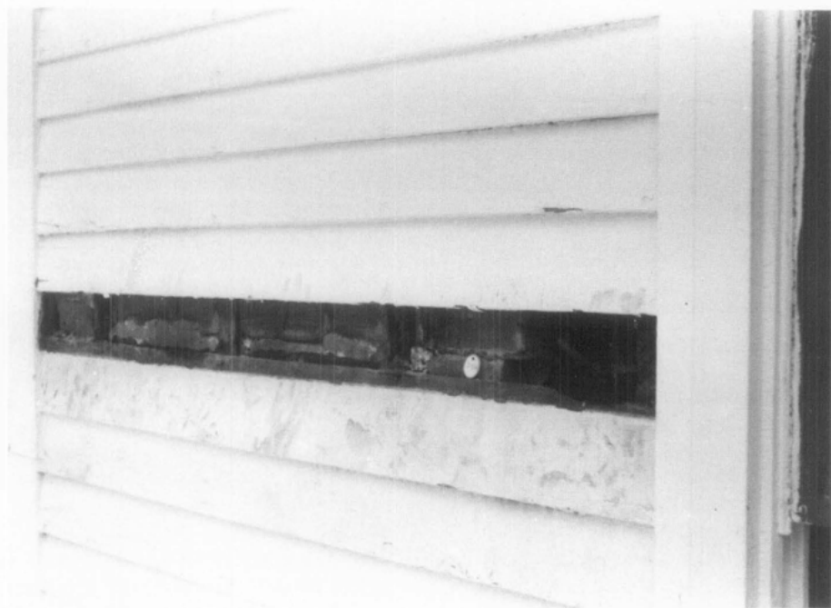
Figure 2. In assessing the safety of using thermal heat to remove paint from the siding, an investigation was performed to determine wall construction and condition. In this portion of the structure, there was no sheathing backing the siding but brick nogging extended from the foundation to the soffit. Photo: Alan O'Bright
