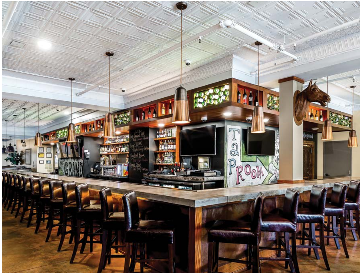
Figure 17. Metal ceilings commonly present code challenges when fire separation is required between different uses on the first and upper floors. Acceptable code solutions permitting retention may include the application of intumescent coatings, the addition of a sprinkler system, or the addition of fire-rated material above the ceiling, in which case the original metal ceilings can be salvaged and reinstalled or, if not possible, replaced with matching new ceiling tiles. Photo: Benton Henry
