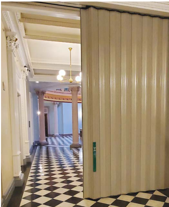
Figure 4: Creative life- and fire-safety code solutions may be required for special buildings and conditions, such as the use of an automatic accordion type, horizontal-sliding fire and security door to meet code requirements. Concealed when not in use, such systems can provide up to a 3-hour fire-resistance rating. Photo: U.S. General Services Administration
