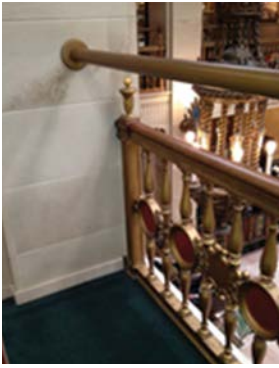
Figure 10. A modern horizontal element was installed to meet the code-required railing height while still retaining the lower historic railing. Photo: Nicholas Vann
