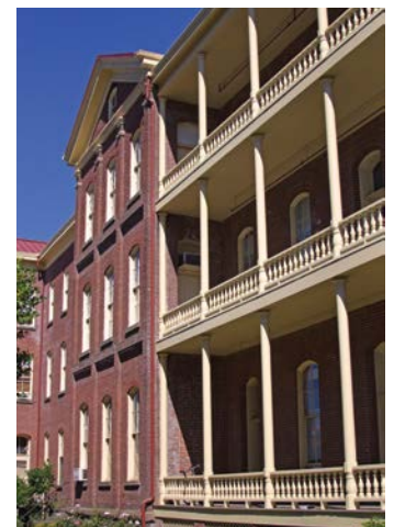
Figure 1: The installation of an exterior automatic fire sprinkler system for the historic multi-story porches allowed these important, character-defining features to be retained to meet life and fire-safety code requirements. Photo: Robert Holcomb
