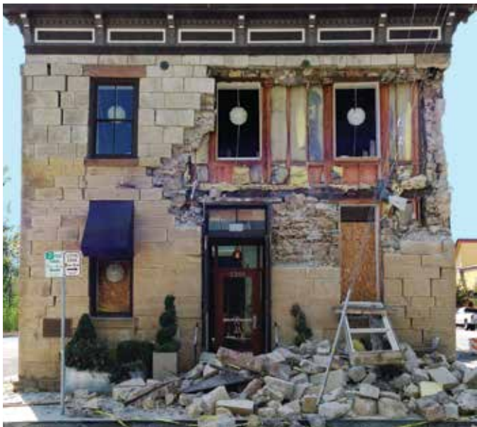
Figure 8. Unreinforced masonry buildings, such as this 1875 stone building damaged during the 2014 South Napa, California earthquake, can be particularly vulnerable to earthquake damage. Photo: Architectural Resources Group.
