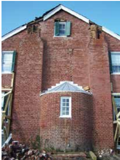
Figure 19. Chimneys are common nonstructural features susceptible to earthquake damage, even in zones of low-to medium-seismic activity as shown on this building
