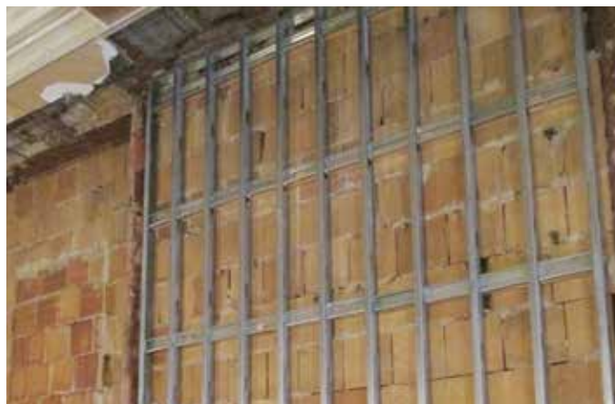
Figure 22. A new steel stud wall is being added to one side of this interior hollow-clay tile wall. The side with the least amount of historic finishes was chosen as the least disruptive location for the added reinforcement. The wall will be returned to its original appearance by installing new finishes matching the historic finishes. Photo: Wiss, Janney, Elstner and Associates, Inc.
