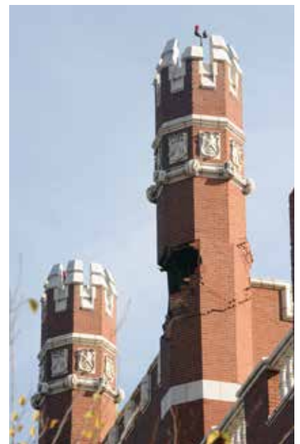
Figure 1. In 2011, a 5.6 magnitude earthquake substantially damaged all four turrets atop St. Gregory's University Benedictine Hall in Shawnee, Oklahoma. Photo: St. Gregory University.
