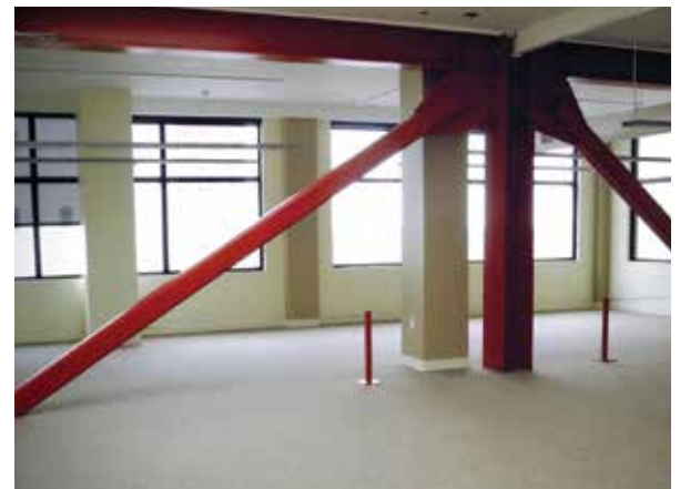
Figures 4-5. Using moment frames (horizontal and vertical steel members identified by the arrows) set back behind storefront openings as seen in Figure 4 (left), or placing brace frames (in red) away from the windows as illustrated in Figure 5 (right) are solutions that meet historic preservation goals. Figure 4. Photo: Elizabeth Hilton.
