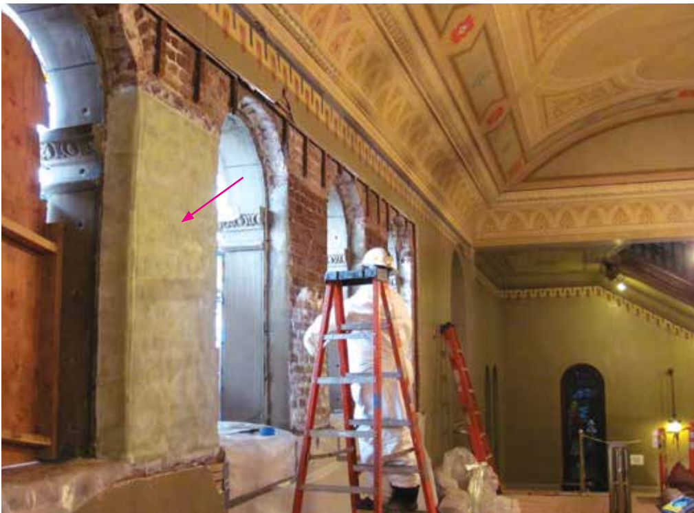
Figure 21. Epoxy-embedded fiberglass mesh is being bonded to the back of the brick pilasters of this 1906 unreinforced masonry building. New finishes matching the appearance and detailing of the original finishes will be applied over the mesh. Photo: Wiss, Janney, Elstner and Associates, Inc.
