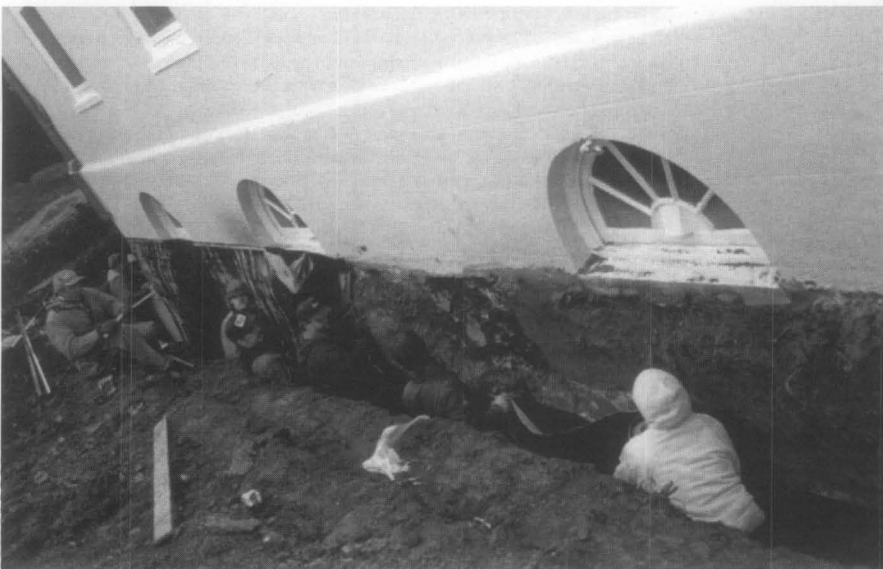
I. Critically damp foundation walls were protected with a layer of bentonite clay to reduce moisture penetration. This work was in combination with new downspouts that were connected to drainage boots that deposited captures roof run-off away from the foundation. Photo: Courtesy, Larry D. Dermody and the National Trust for Historic Preservation.
