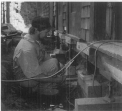
B. Wood sills set on grade were replaced with concrete pier foundation and new wooden sill plates. Changes were not visible on the exterior (see C). Photo: WPTC, NPS.
