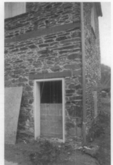
E. Mechanical systems on the lower level were placed on platforms above the flood line. Harper's Ferry Center, NPS.
