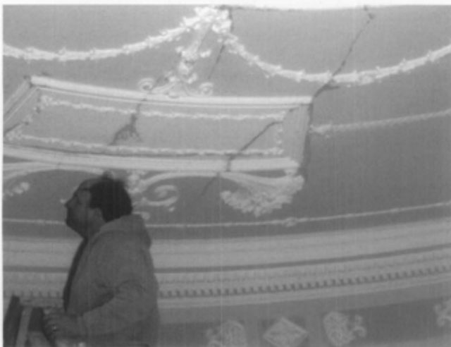
Fig. 6. Uninsulated plumbing pipes close to the exterior wall froze and cracked, wetting this ornamental plaster ceiling before the water supply line could be shut off. As a result, limited portions of the ceiling needed reattaching. Photo: author.
