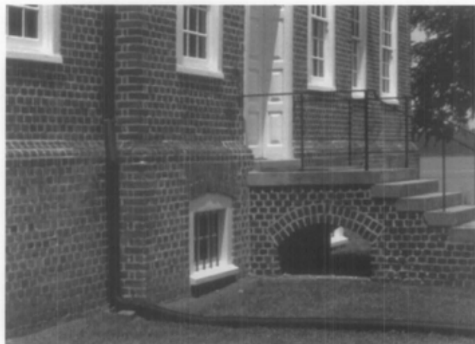
Fig. 17. In testing a theory for the cause of basement wetness, the owner used long black extender pipes to direct roof run-off away from the foundation. This test established that the owner did not need expensive waterproofing of the foundation, but a better drainage system. Photo: Baird M. Smith.
