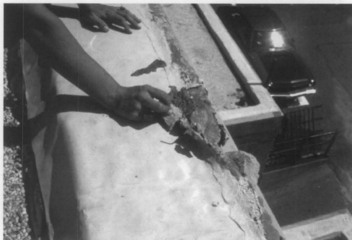
Fig. 1. Moisture problems, if not properly corrected, will increase damage to historic buildings. This waterproof coating trapped moisture from the leaking roof, causing portions of the masonry parapet to fail. Photo: NPS Files.
