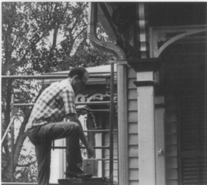
Fig. 19. Maintaining gutters and downspouts in good operable condition, repairing exteriors to keep water out, redirecting damaging moisture away from foundations and controlling interior moisture and condensation are all important when holding the line on moisture deterioration. Photo: Nebraska State Historical Society.
