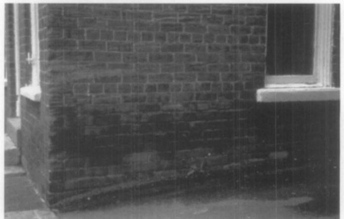
Fig. 11. Capillary rise of moisture in masonry is often accompanied with a horizontal tide-mark line several feet above the grade, as seen here. Removing or redirecting as much ground moisture as possible usually helps reduce moisture within a wall. Photo: NPS Files.
