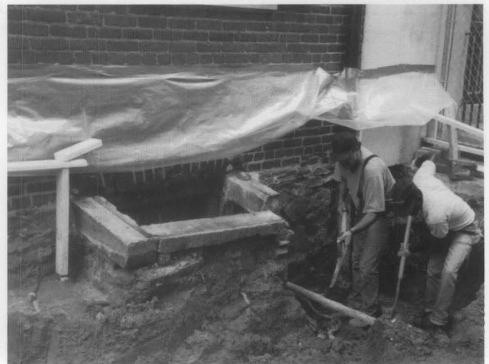
Fig. 5. Excavating this foundation revealed that the downspout pipe had corroded at the “u-trap” and was leaking moisture into the soil. Openings around the horizontal water supply line and cracks in the wall allowed moisture to penetrate the basement in multiple locations. Photo: author.
