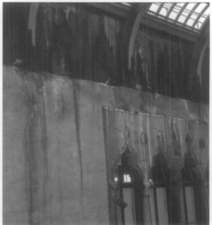
Fig. 7. Condensation dripping from the large overhead courtyard skylight was damaging the masonry in this museum. A new skylight with thermal glazing was installed, replacing the deteriorated single-glazed unit. A new climate control system monitors interior temperature and humidity. Photo: © Isabella Stewart Gardner Museum, Boston.
