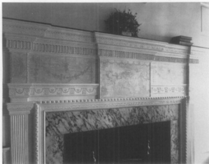
Figure 29. The ghost marks of compo past—floral swags or festoons—are in clear evidence on a mantelpiece in the back bedroom of the George Read II House, New Castle, Delaware. This physical evidence will be used to assure their accurate re-creation in a restoration project. Photo: Courtesy, Gold Leaf Studios, Inc.
