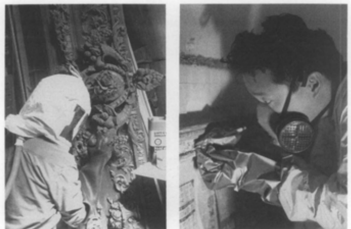
Figure 23. Methylene chloride fumes can be deadly, so protecting the worker is imperative. Left: a hooded, air-fed unit. Right: a vapor mask with organic solvent cartridges. Photo left: William Adair. Photo right: Lonnie J. Hovey, AIA.
