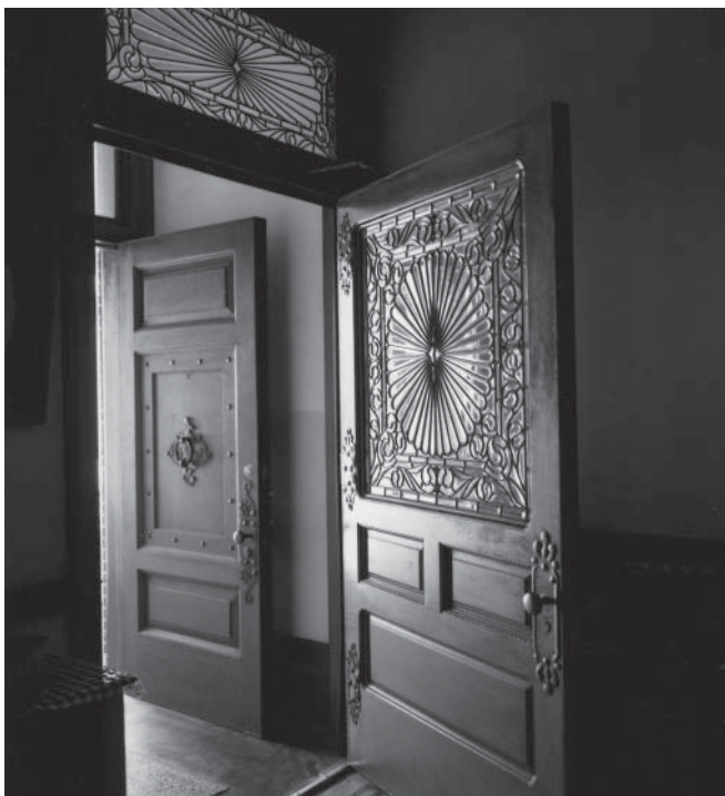
Figure 1. This door and transom suggest the richness of 19th century leaded glass. Photo: Jack E. Boucher, HABS.
