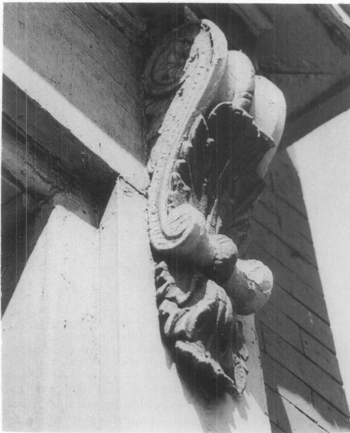
Fig. 1 Excessive paint build-up on architectural details such as this ornamental bracket does not in itself justify total paint removal. If paint is cracked and peeling down to bare wood, however, it should be removed using the gentlest means possible. Photo: David W. Look, AIA.
