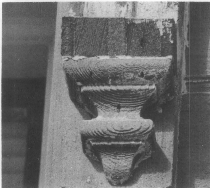
Fig. 12 Sandblasting has permanently damaged this ornamental bracket. Even paint will not be able to hide the deep erosion of the wood. Photo: David W. Look, AIA.
