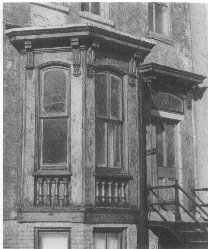
Fig. 2 A traditionally painted bay window has been stripped to bare wood, then varnished. In addition to being historically inaccurate, the varnish will break down faster as a result of the sun's ultraviolet rays than would primer and finish coats of paint. Photo: David W. Look, AIA.
