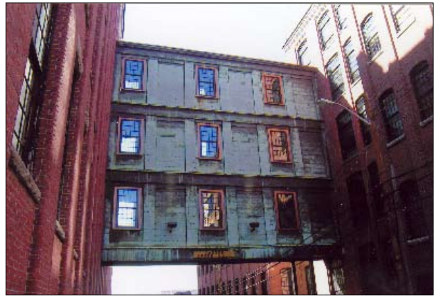
Repair and replacement in kind allowed this industrial bridge to retain its historic appearance and to continue its service as a connector.
