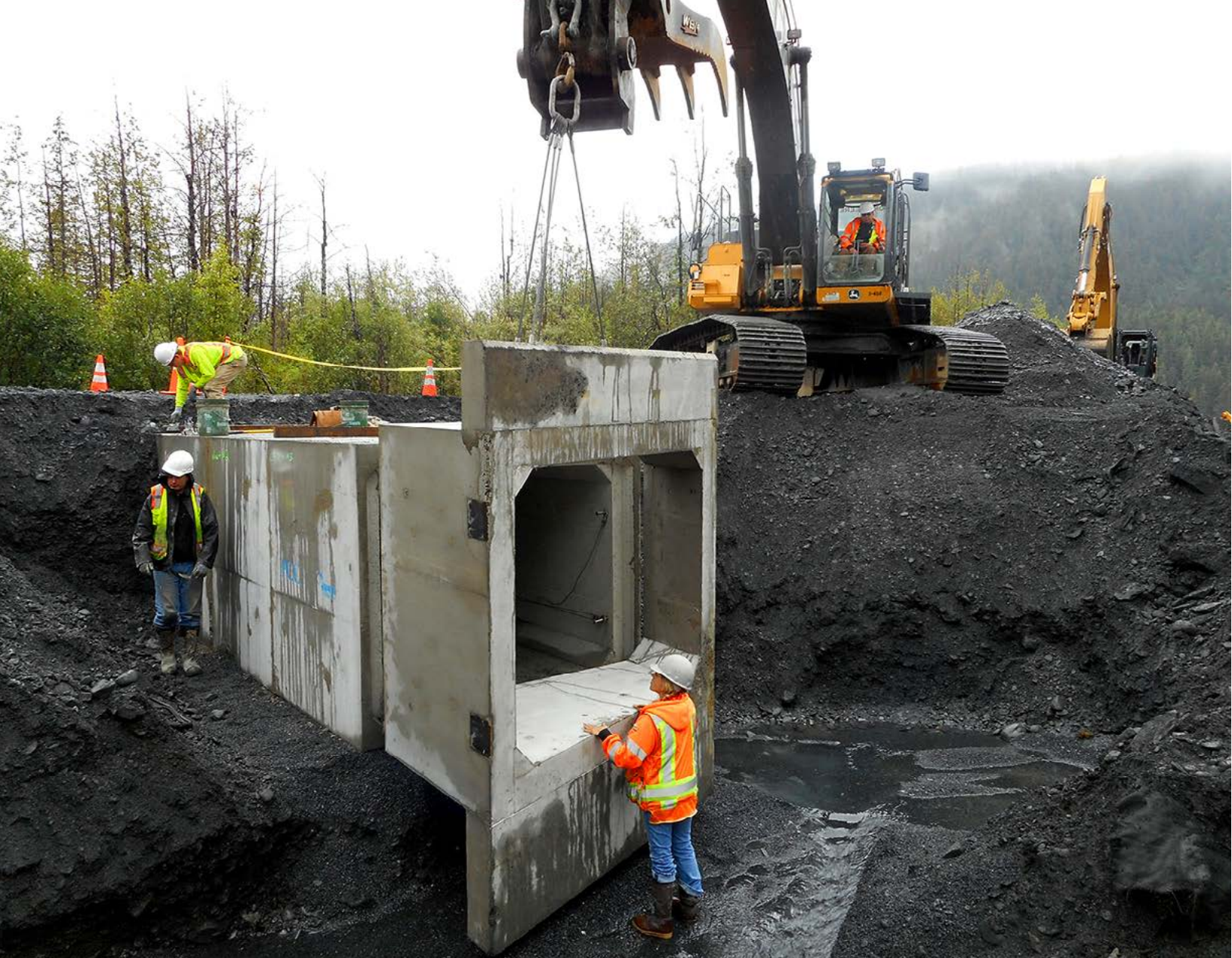
Installation of one of the five new concrete box culverts under Exit Glacier Road at Kenai Fjords National Park.
