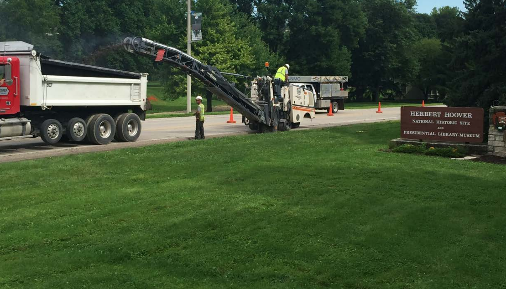
Asphalt Shoulder removal on Parkside Drive in Herbert Hoover National Historic Site.
