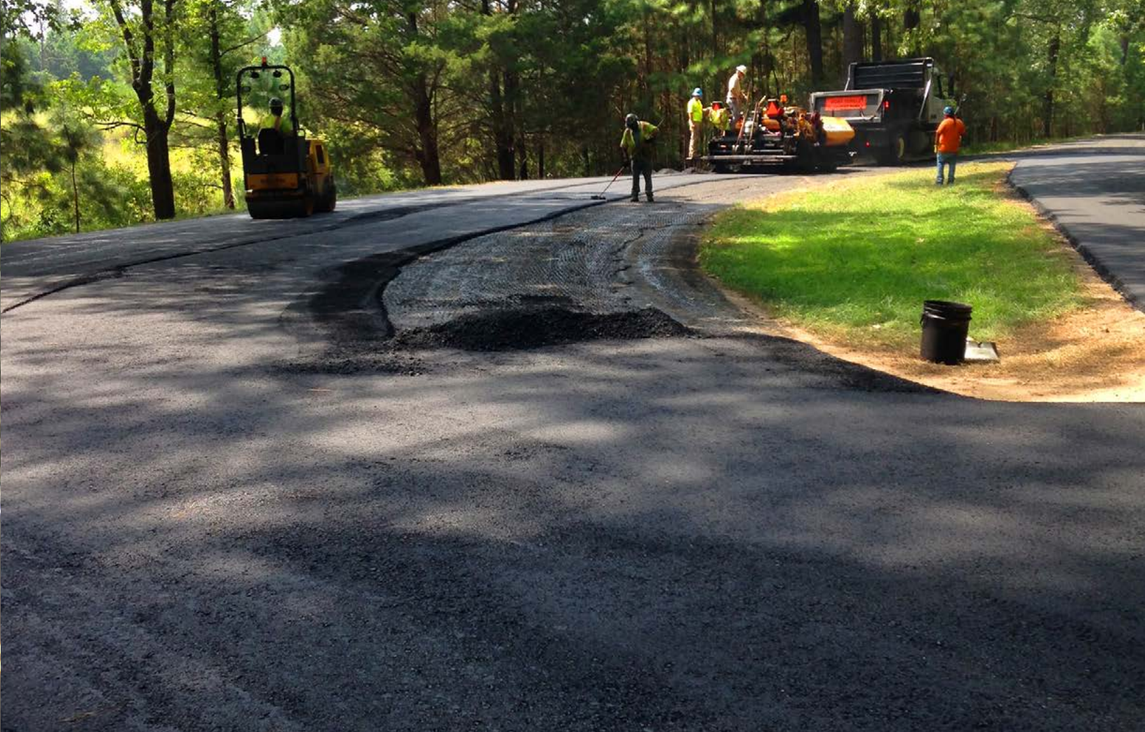
Mill and overlay paving work on Island Drive Loop in Colonial National Historical Park.
