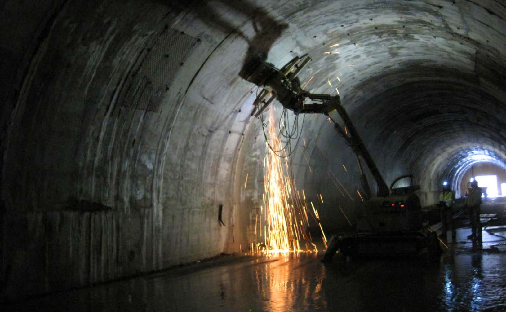
Maintenance work inside the Tanbark Ridge Tunnel at Blue Ridge National Park.
