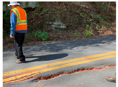
Road damage from a slide at New River Gorge National River. (NPS Photo)
