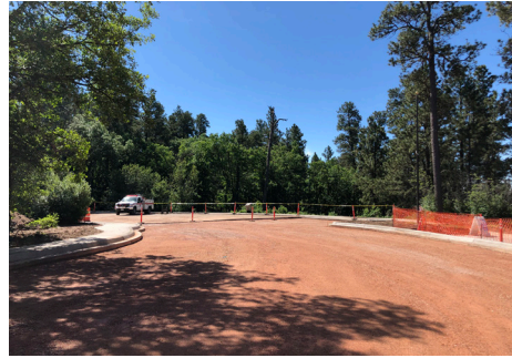
Construction on the Devils Tower Parking Area to improve accessibility. (NPS Photo)
