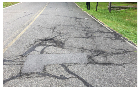
Road damage at Morristown National Historical Park. (NPS Photo)
