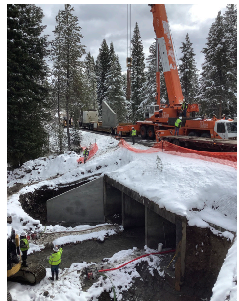
Improvements to the Arizona Creek Bridge at Grand Teton National Park. (NPS Photo)
