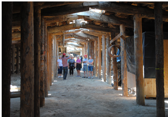
Contractor Sol Martin leads a tour of the work in the root cellar. Photo courtesy of the Heart Mountain Wyoming Foundation.
