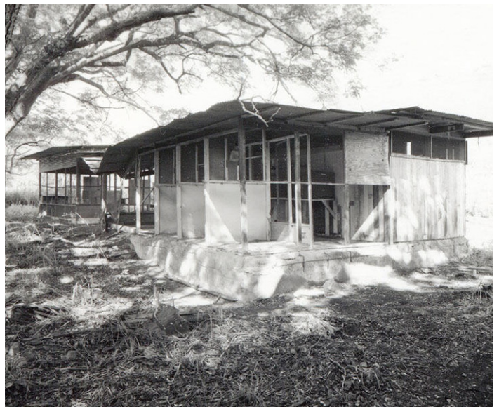
Two remaining buildings at Honouliuli were evaluated as part of an educational practicum. Photo courtesy of Minatoishi Architects.
