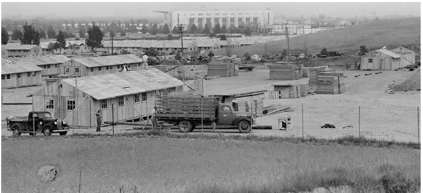
General view of "assembly center" being constructed on Pomona Fairgrounds, California, April 8, 1942. Photo courtesy: Densho (ddr-densho-37-390), National Archives and Records Administration Collection, photo by Clem Albers
