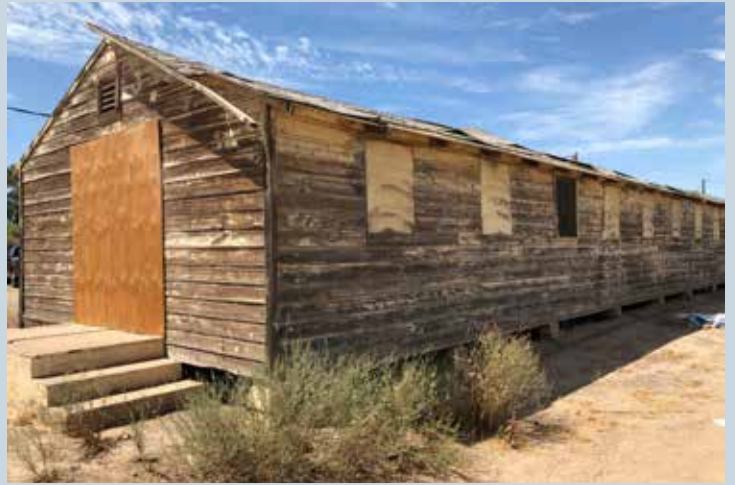
Historic barrack from Poston incarceration site in Arizona. Photo courtesy of Barbara Darden, Scheuber + Darden Architects.
