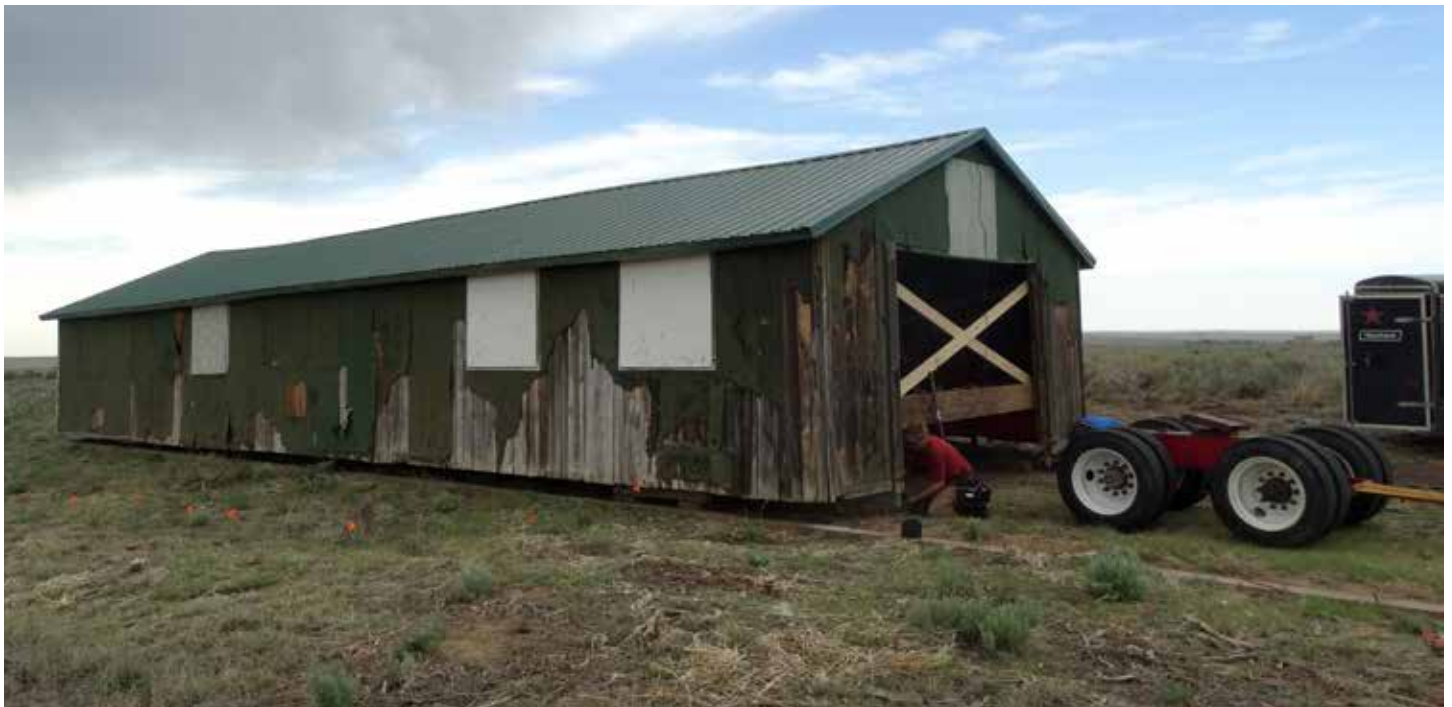
Moving the historic recreation hall back to Amache. Photo courtesy of Barbara Darden, Scheuber + Darden Architects.
