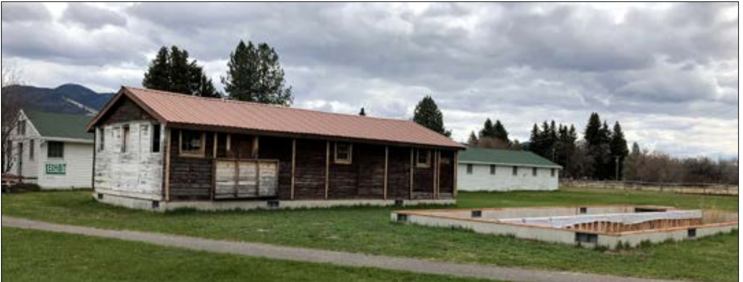
The Historical Museum at Fort Missoula will conduct an assessment of two original barracks moved back to the former World War II Department of Justice internment site to inform future restoration of the buildings and interpretation of the site's history. Image courtesy of Historical Museum at Fort Missoula.
