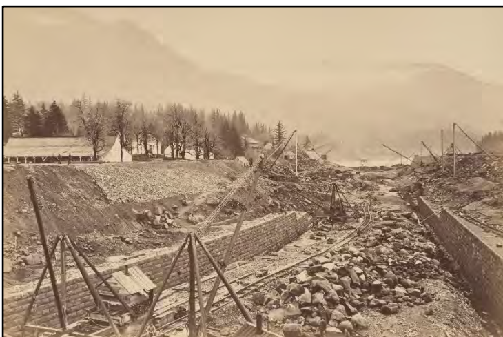
Figure 48. Cascade Locks under construction, viewed from the east. Photograph by Carleton E. Watkins, ca. 1883.
