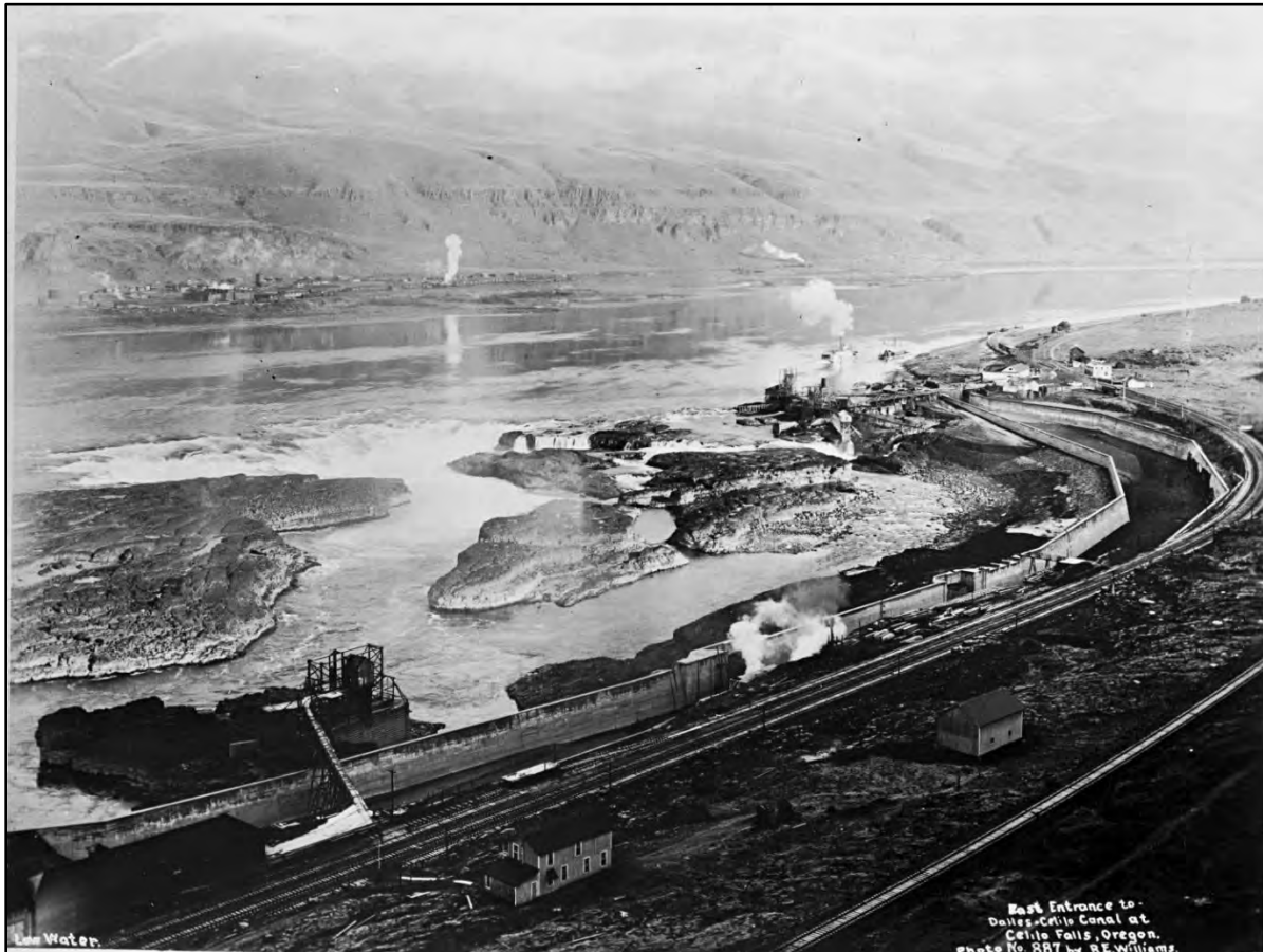
Figure 51. The Celilo Canal under construction in the foreground, viewed from the south bank of the Columbia River. The railroads on both sides of the river are visible, as is a steamboat just upstream of the falls. Photography by R. E. Williams, 1913.
