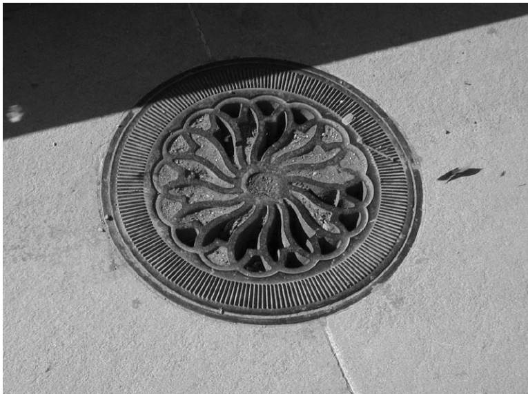
The ornamental flourish of the drainage grates set around the reflecting pool contrast with the stark simplicity of the rest of the SOM design. (CLP file "decorative grate" Feb. 24 2006)
