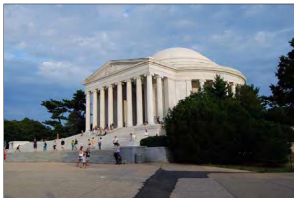
Temporary paving repairs have been made on the north plaza to correct problems caused by the settling seawalls. Permanent repairs have been funded through the American Recovery and Reinvestment Act of 2009.
