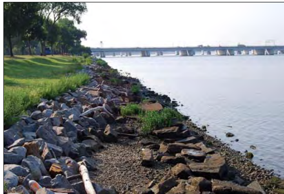
Dry-laid stone riverwalls have deteriorated, and riprap is used in some areas to control erosion.
